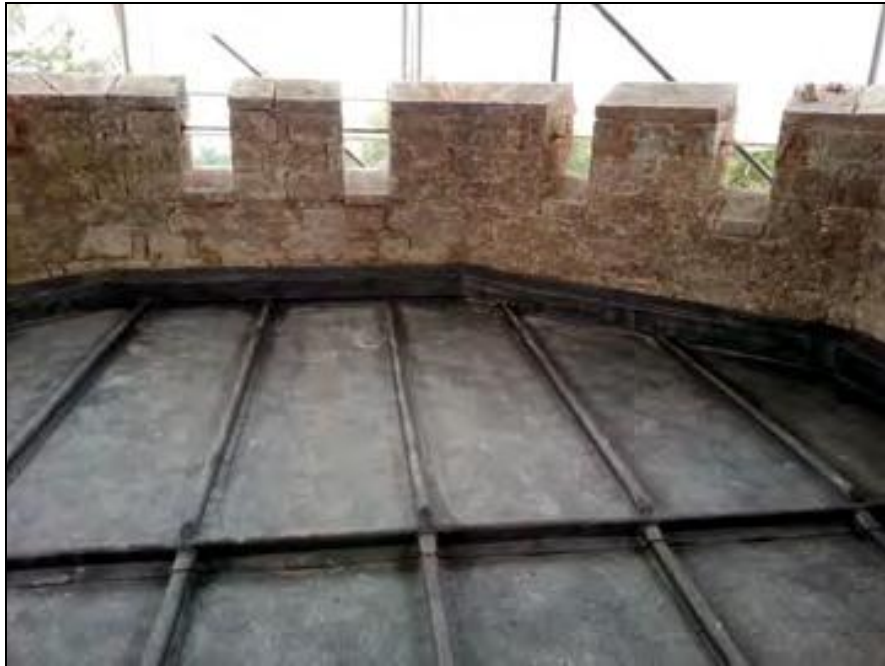
View of roof terrace with embattled parapet which has been stripped of render, exposing dressed stone to the crenellations; this may originally have been pointed, contrasting with the original white render of the building when new, adding to its Gothic-style. The new leaded roof can be seen to have been fitted.
