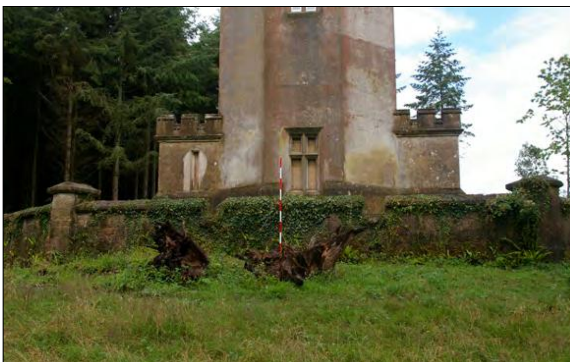
Figure 7: The terrace and tower, showing the blocked ground floor mullion-and-transom window; from the south.
