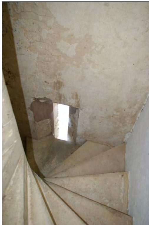
Figure 15 View down the spiral stair, showing the square corners and the stairs cutting across a window; from the south.
