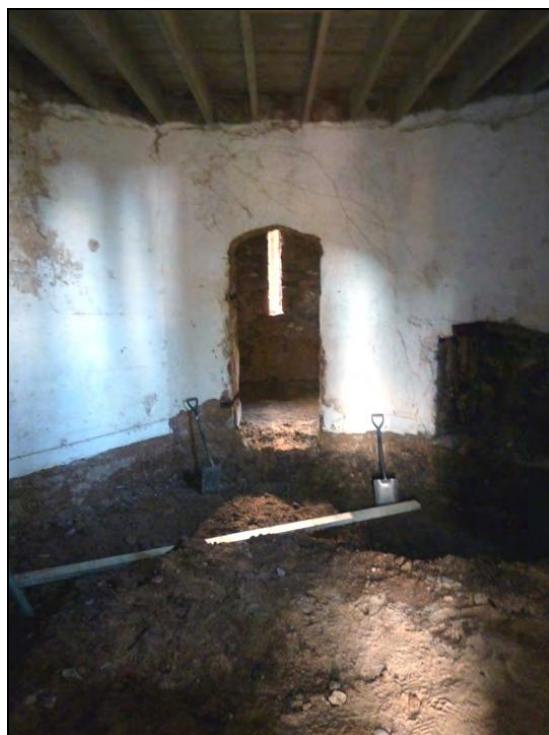
View from the entrance porch across the kitchen to the service room; showing the earth floor which has been removed by hand. The blocked arrow slit window in the service room can be seen to have been opened.
