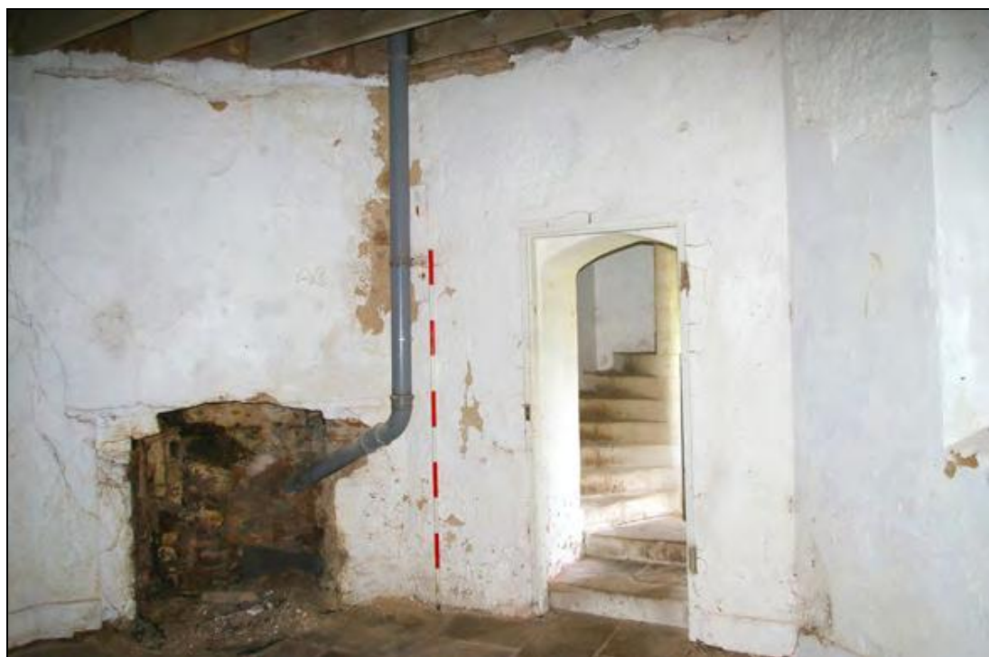
Figure 12 The south-west corner of the ground floor room, showing the fireplace and door to the stair; from the north-east.
