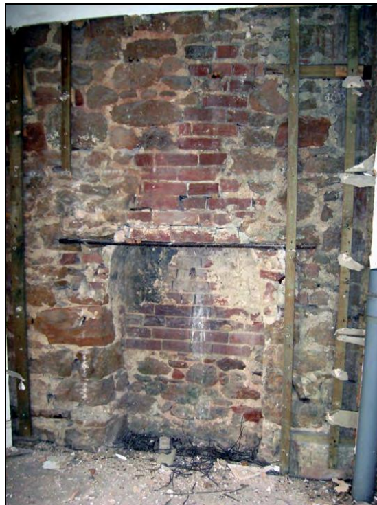
Photograph of the fireplace which serves the third floor room; showing it stripped of plaster. The stone stack and former open stone-built hearth can be seen to be patched with brick, possibly from late 19 th century or a 20 th century grate or stove.
