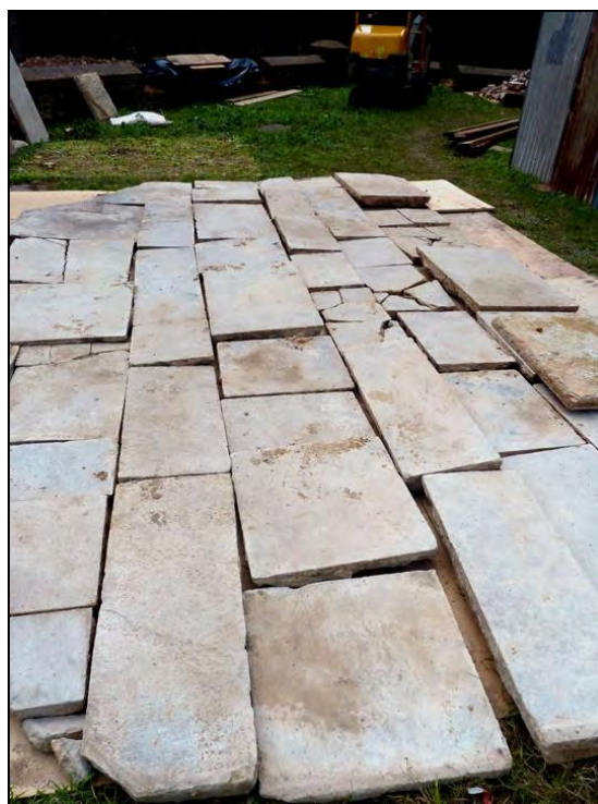
Photograph of the stone flagged floor from the kitchen, removed by hand, showing the cleaned and recorded stones.
