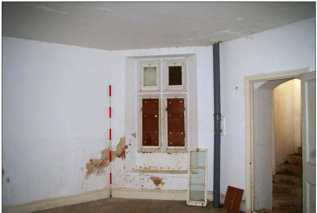
Figure 14: The south-west side of the first floor room showing the blocked mullion-and-transom window, from the north-east.
