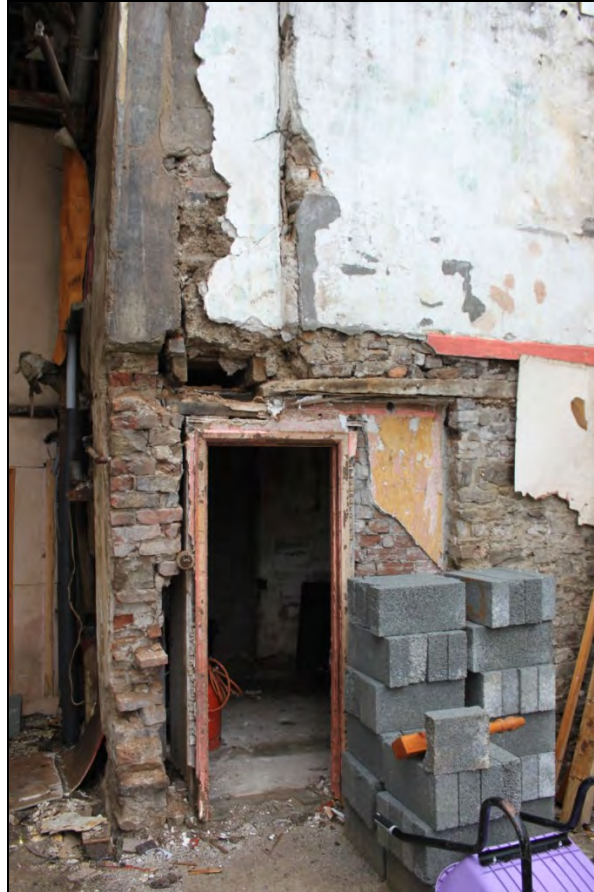
Figure 28: Door to Kitchen of Building 7 in north elevation of north-west outbuilding, viewed from the north.
