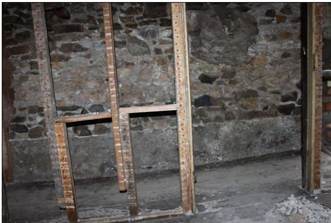
Figure 33: East elevation of second floor of the Building 7, viewed from the east.
