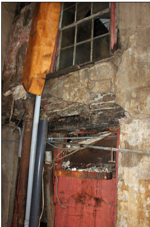
Figure 29: Hornless sash window above blocked doorway in east wall of north-west outbuilding, of Building 7, viewed from the north-east.
