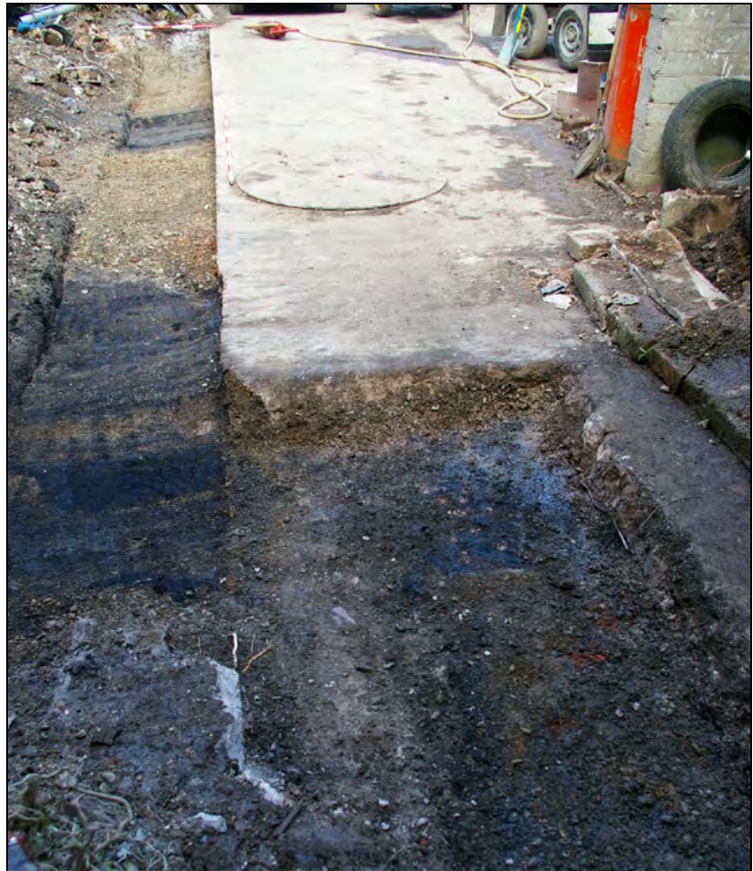
Figure 3: Trench #1, viewed from the south, looking north (scale 1&2m). Note the dark bands in the natural shillet bedrock.
