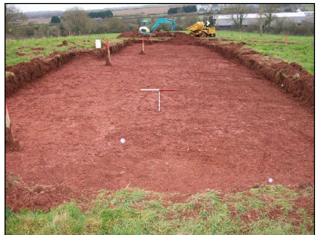
Photo 6: Excavated area in south-east portion of the site, posts denote corners of proposed buildings, looking West (scales 1 & 2m).
