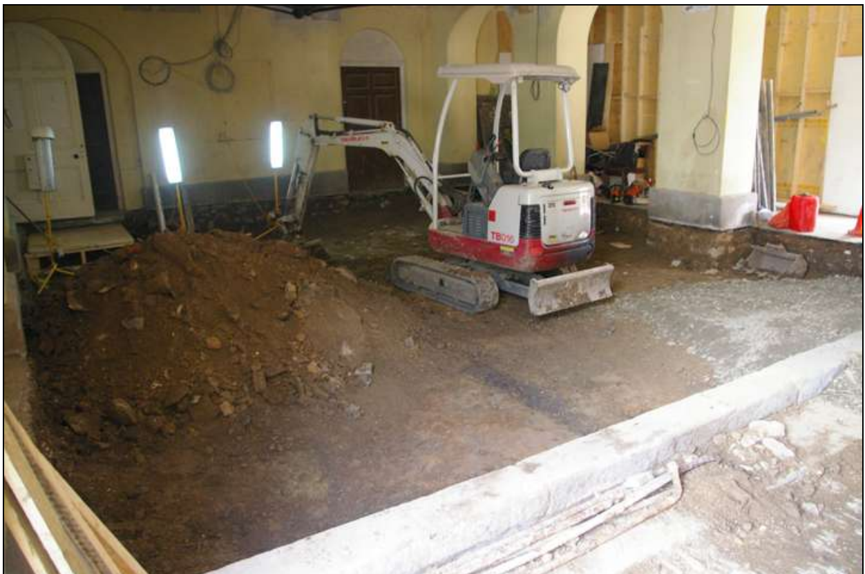
Site shot post-excavation/floor reduction, viewed from the north-west corner, looking south; viewed from the north-west (no scale).
