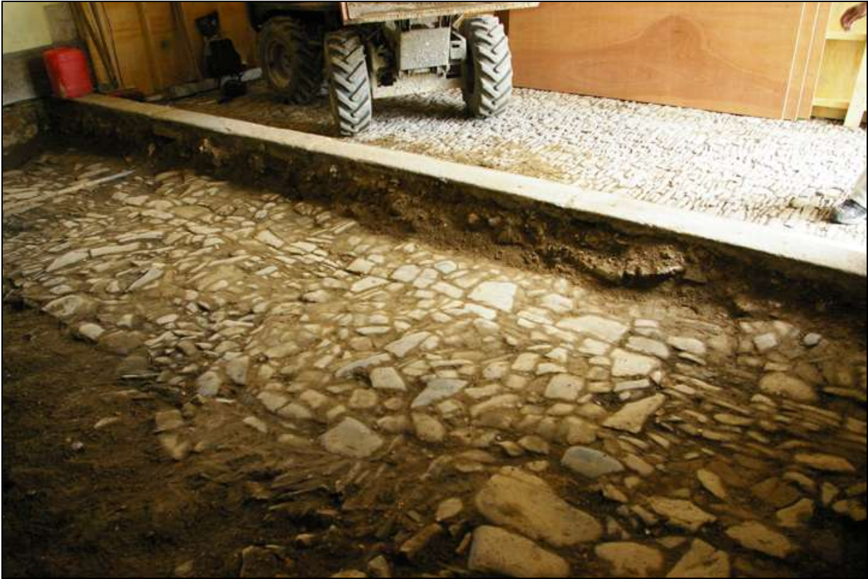
Site shot mid-excavation showing Cobbled Floors (108) and (105); viewed from the south-east (no scale).
