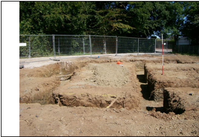
Figure 1: Post-ex footings trench for plots 1 and 2, viewed from the south (2m scale).
