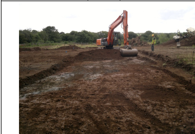
Figure 3: Excavation of access road showing cut of fuel pipe, viewed from the north-west, (no scale).
