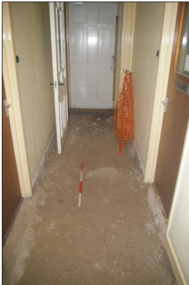
Figure 3: Shot of the finished level in the hall, from the northwest with flash (1m scale).
