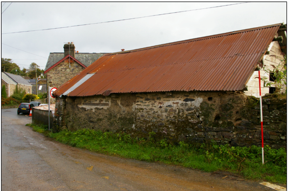
Figure 9: The exterior west wall of Building 3 with the rubble stone and lime mortar repairs, viewed from the south-west.
