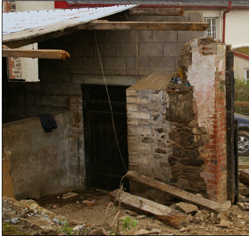
Figure 7: The rubble stone wall between the doors in the east elevation of Building 2 after the demolition of Building 3, viewed from the south-west.
