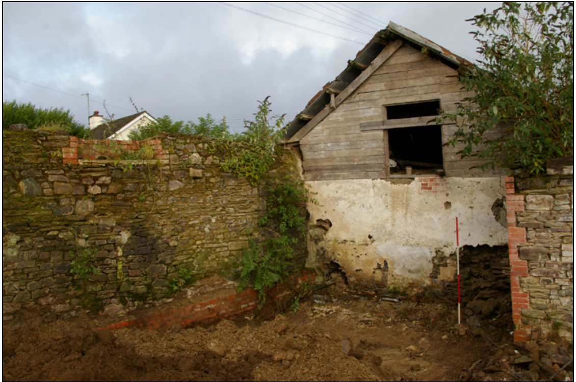
Figure 12: The interior north-west corner of Building 4 and south wall of Building 3, viewed from the south-east.
