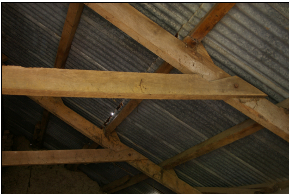
Figure 11: The roof structure on the eastern pitch of Building 3, viewed from the south-west.
