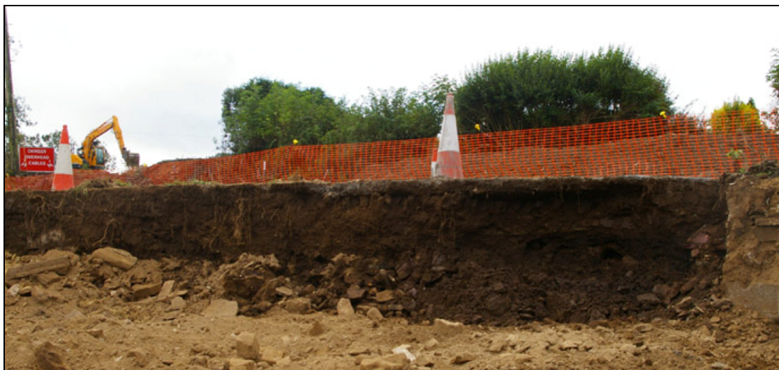
Figure 14: The south-western boundary of the site after removal of the former west wall of Building 4, viewed from the north-east.
