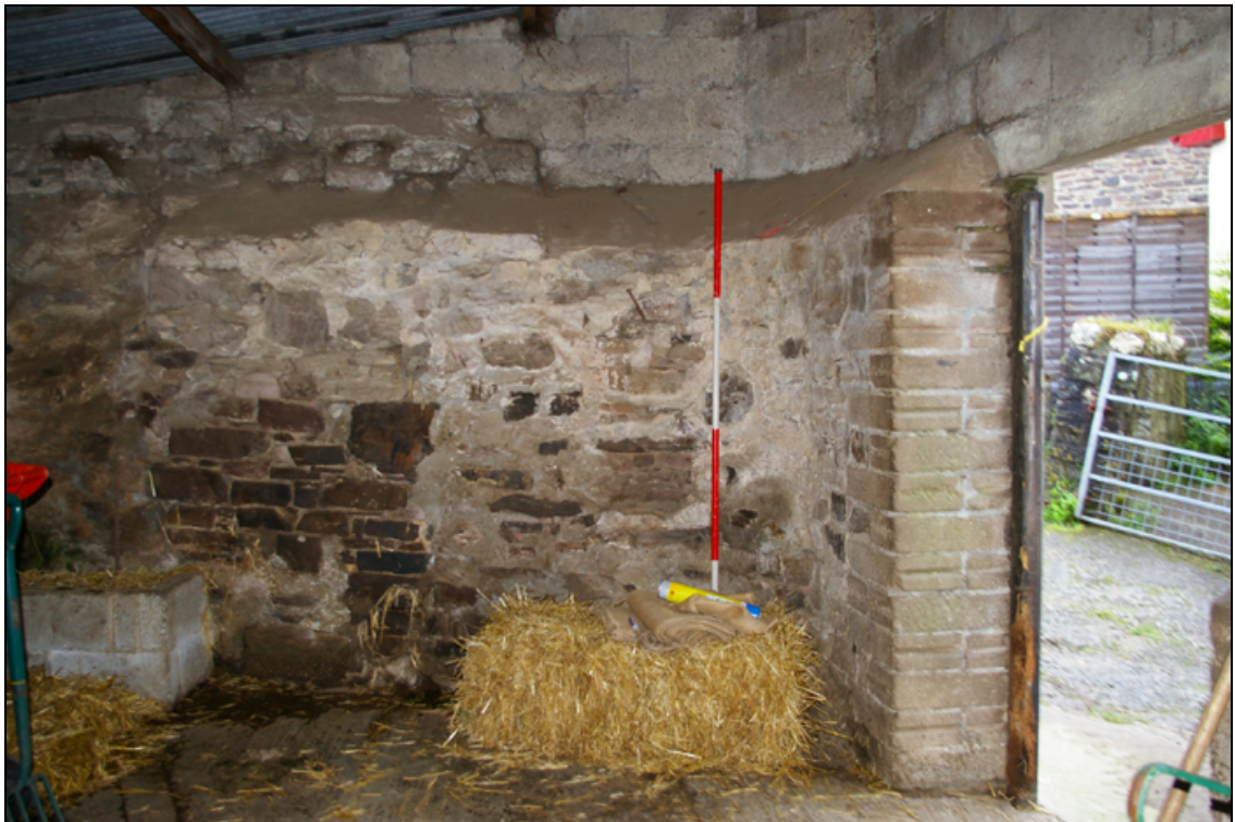
Figure 6: The interior rounded north-east corner of Building 2, showing the earlier rubble stone construction below, the concrete block upper and door jamb, viewed from the south.
