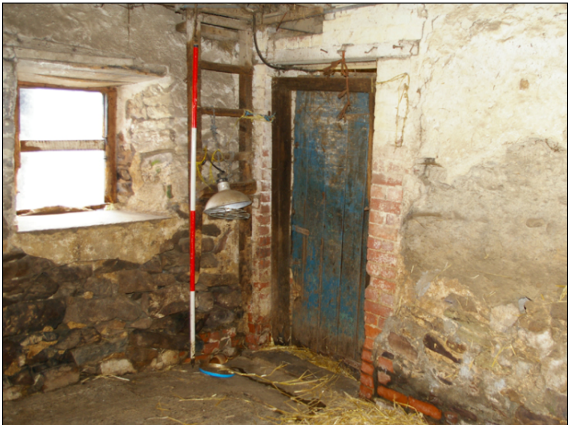
Figure 10: The interior south-east corner of the northern portion of Building 3, showing the forced door opening and the earlier window, viewed from the north-west.
