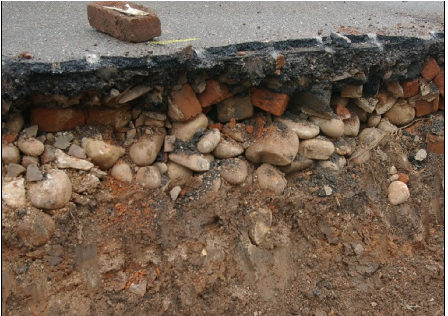
Figure 4: The area of pebbles with possible herringbone brickwork above in the northern retaining wall trench, viewed from the southwest.
