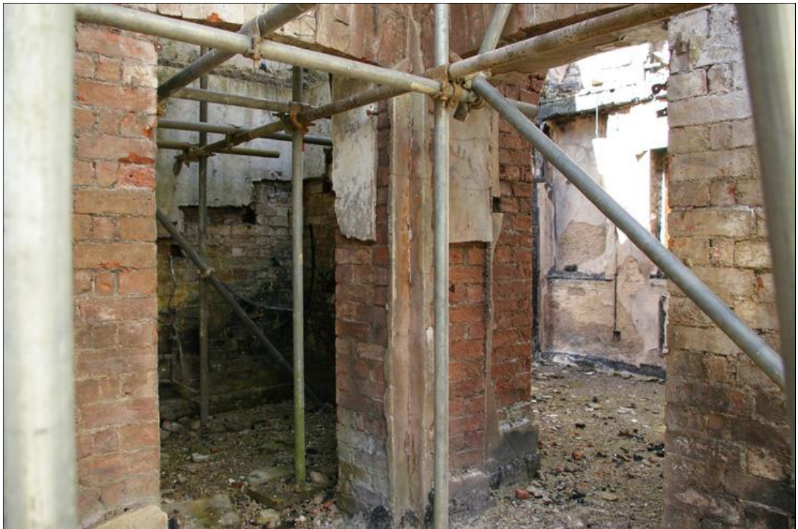
Figure 9: The door opening (D4) into the stair lobby (R4) and the opening (D2) into kitchen (R4) in the north-east.
