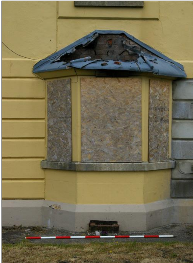
Figure 8: The bay window on the exterior south elevation of the Lodge, viewed from the south (2m scale).
