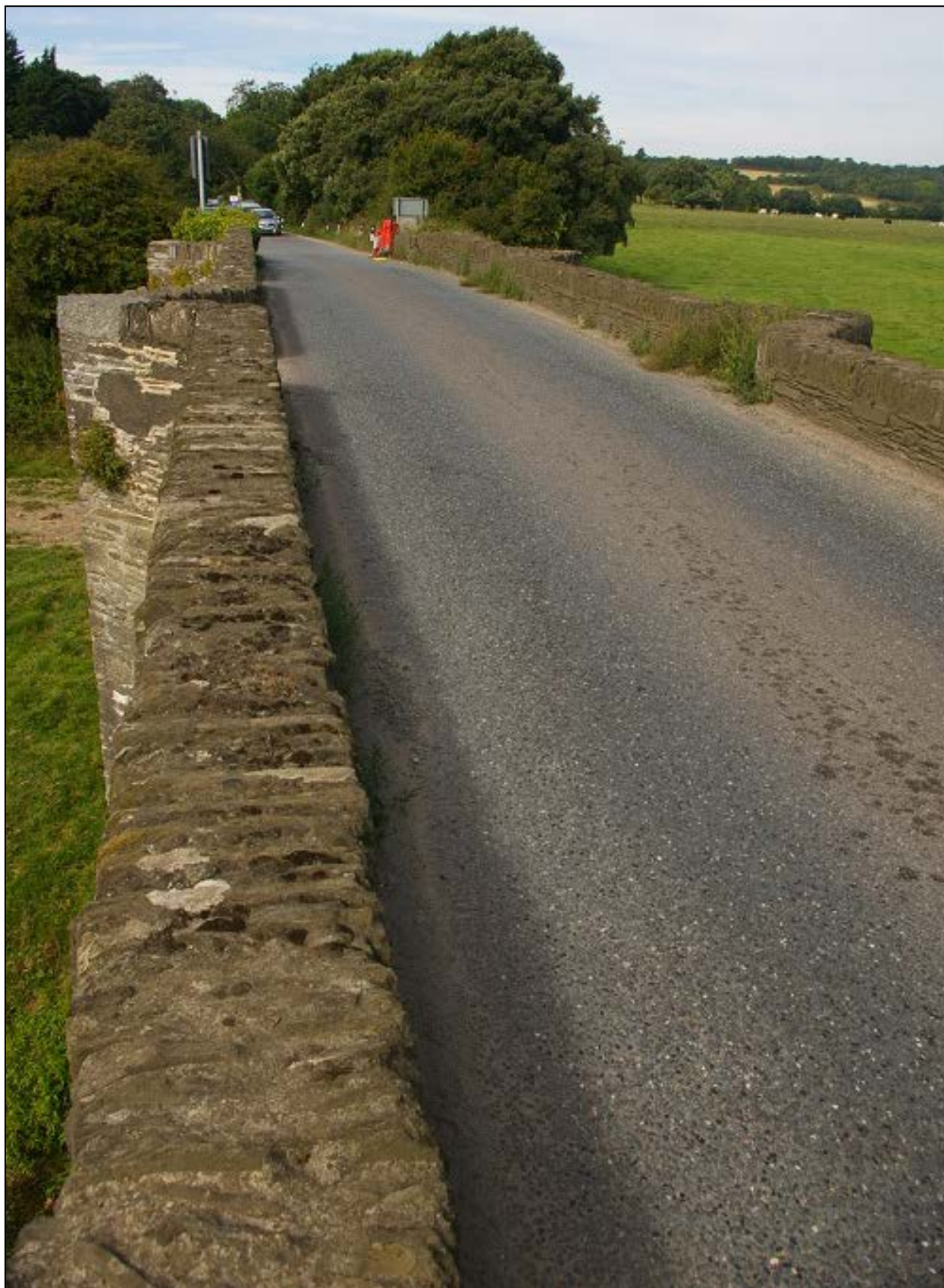
View along Trewornan Bridge towards Trewornan Farm, set in the trees; from the east.
