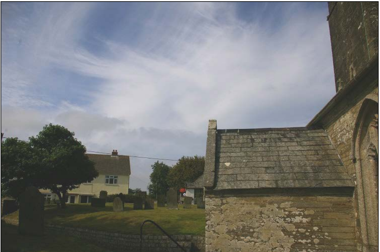
The view south-west and west from St Mabena's in St Maybn, with the houses surrounding the church, but the church raised within its compound on high ground; from the east.
