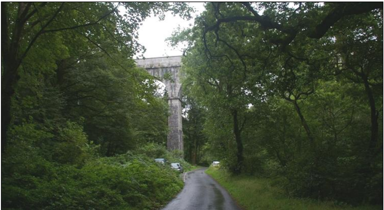
The Treffry Aqueduct within the Luxulyan valley, surrounded by the trees of the valley; from the north.
