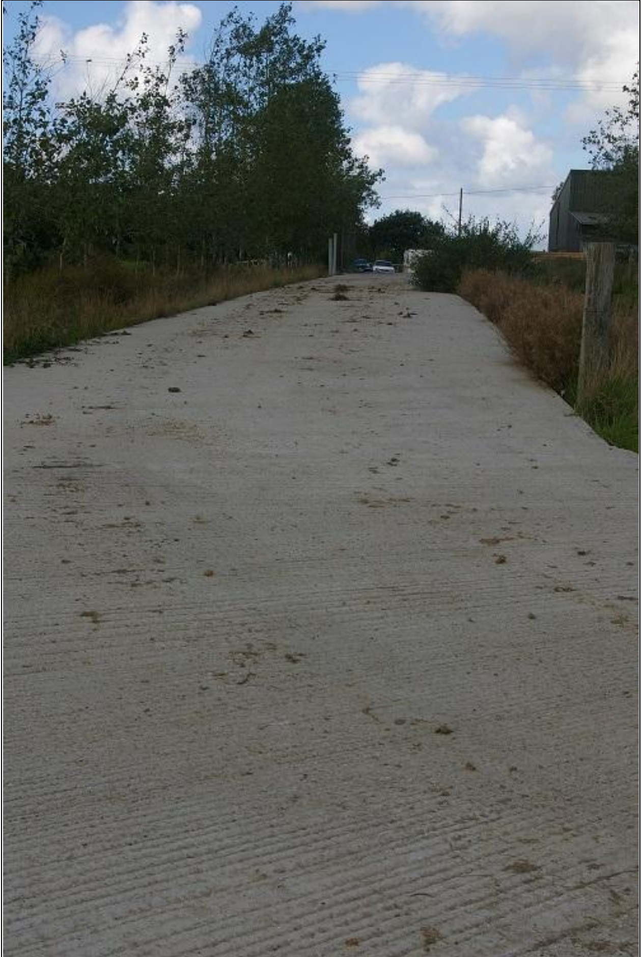
The concrete track/path which provides access to the field; from the south.
