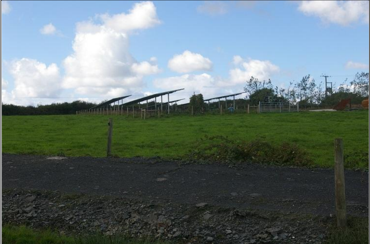
The photovoltaic units which are already installed to the north-west corner of the field; from the south-east.
