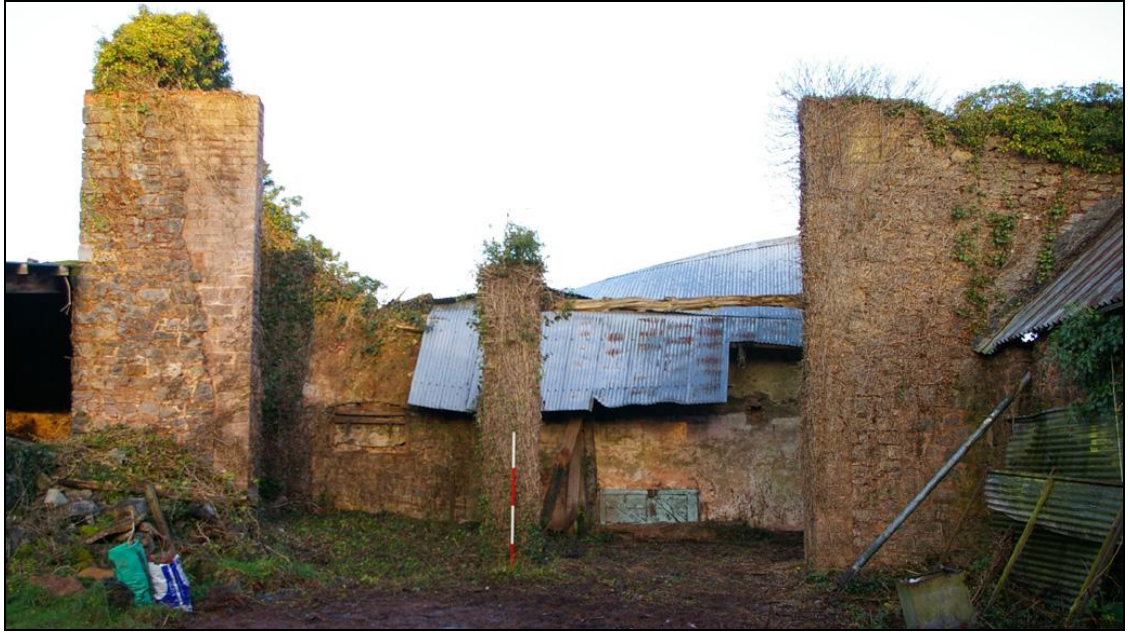
Figure 11: The open west elevation of Building 5, showing the central partition wall, viewed from the west (2m scale).
