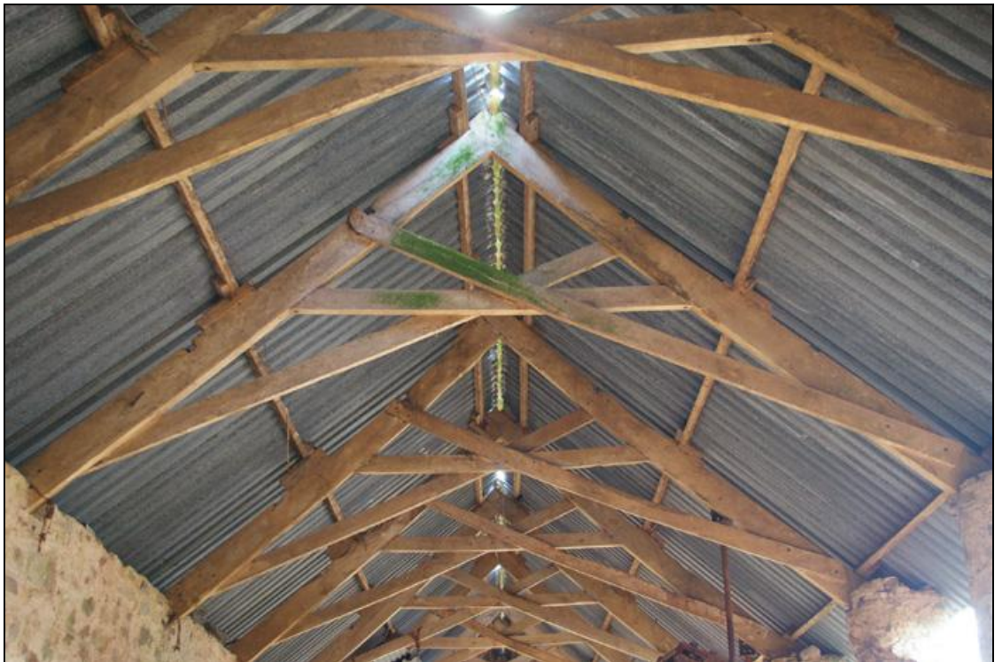
Figure 18: The roof structure of Building 6, showing the scissor brace trusses, viewed from the east.
