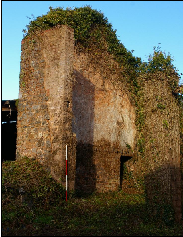
Figure 13: The three storey north gable of building 5, viewed from the south-west (2m scale).
