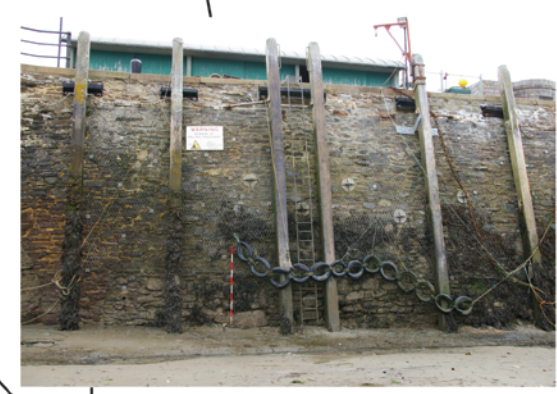
Note the numerous patches of remortared masonry. This probably represent numerous phases of hasty reconstruction, during occasions of urgent need of repair to the inner wall.
