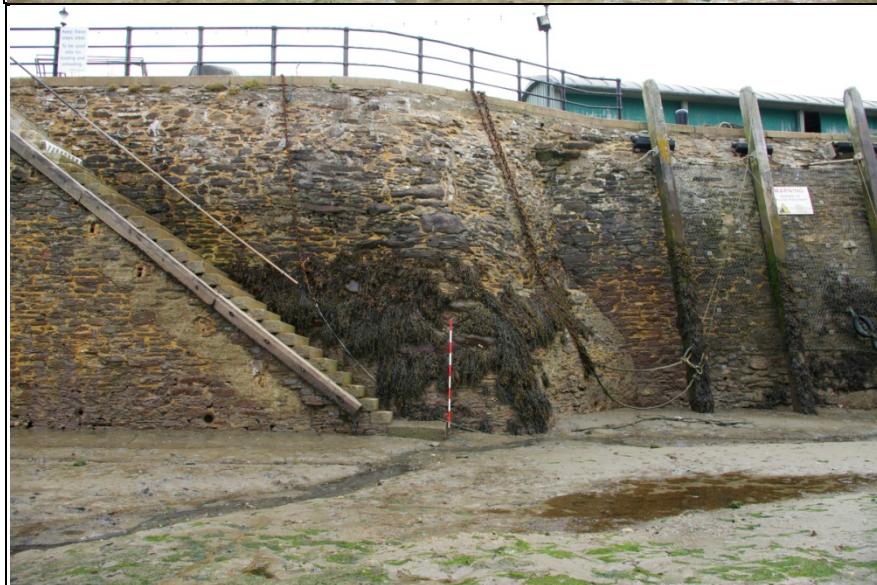
Top: The western side, northern portion, from the south-west (2m scale). Middle: The west side, to the north of the steps, from the west (2m scale). Bottom: The west side, to the south of the steps, from the west (2m scale).
