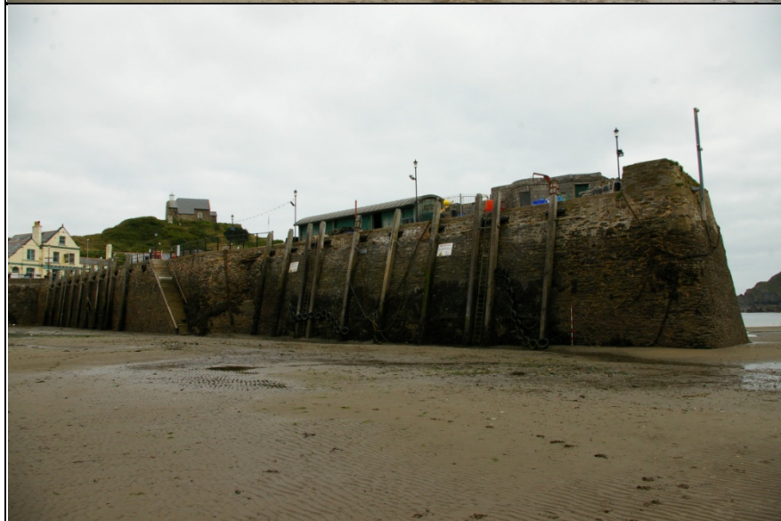
Top: The western side, southern portion, from the north-west (2m scale). Middle: The west side, southern end, from the west (2m scale). Bottom: The whole western side of the pier, from the south-west (2m scale).
