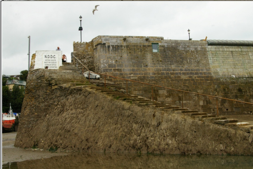
Top: The western side, south end, from the south-west (2m scale). Middle: The south end, from the south (2m scale); Bottom: The steps & slip-way at the southern end of the east face, from the east (no scale).
