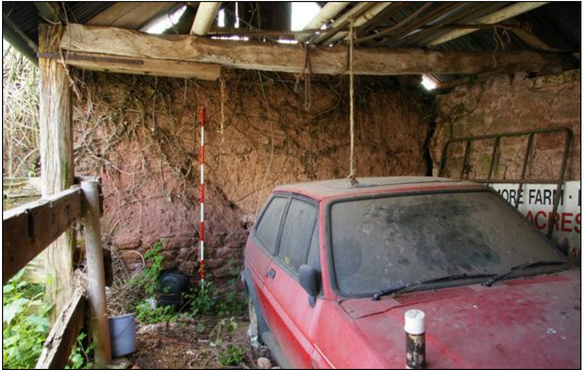
Figure 18: The south-east end of B4 abutting the wall of B5, viewed from the north-west (2m scale).
