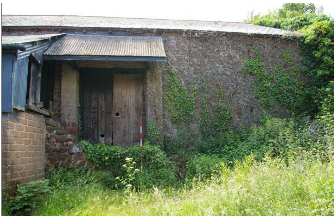
Figure 11: The west end of the north elevation of Building 3 (B3), viewed from the north (2m scale).
