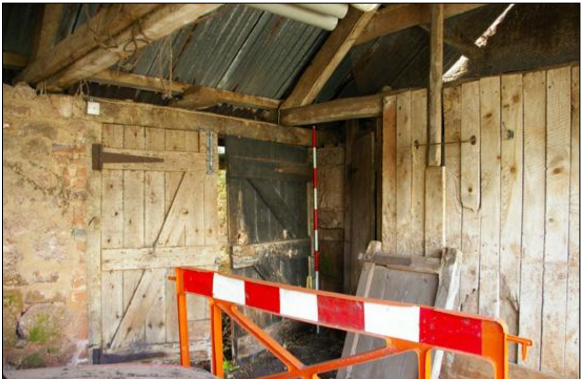
Figure 19: The door openings to the exterior and into the compartment at the north-west end of B4, viewed from the south-east (2m scale).
