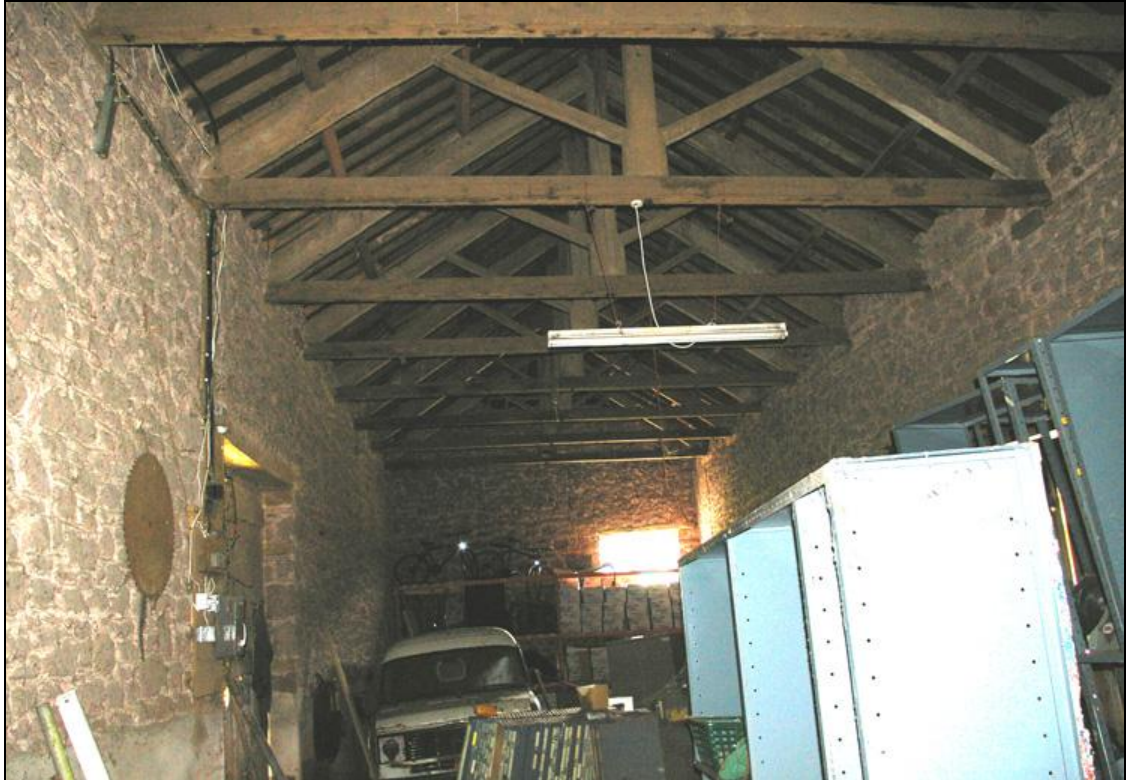
Figure 13: The interior south-east end of B3, showing king post roof structure, north doors and window opening in the east gable, viewed from the north-west.
