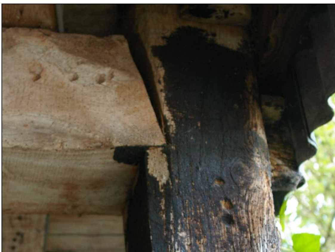
Figure 17: Detail of the carpenter's marks on the posts and joists within B3a, viewed from the south east.
