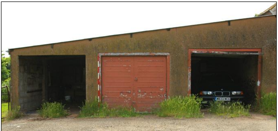
Figure 24: The exterior north elevation of B6, viewed from the north (2m scale).
