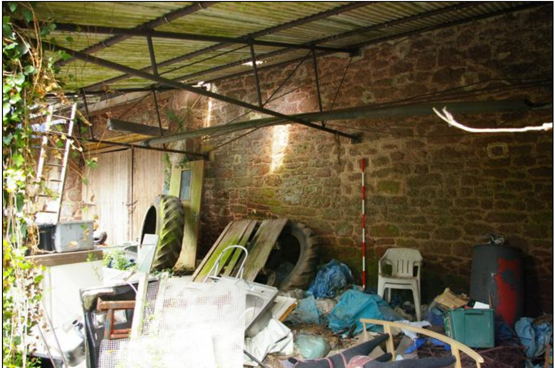
Figure 12: The exterior south wall of B3, within a mid to late 20 th century lean-to, with south doors to the left, viewed from the east (2m scale).
