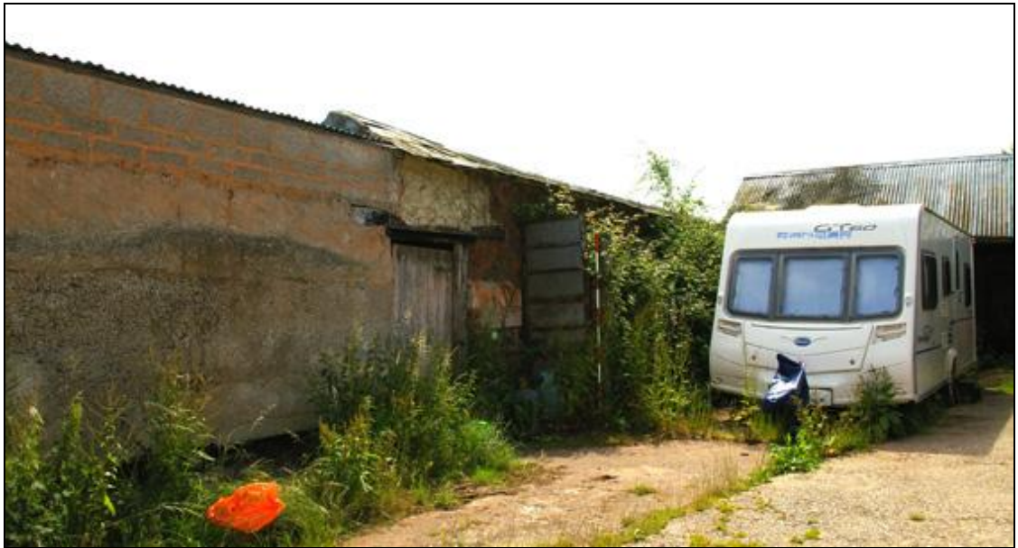
Figure 20: The exterior west wall of Buildings 5 and 6, viewed from the north (2m scale).
