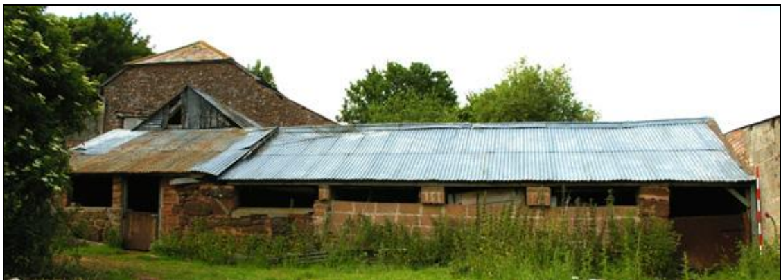
Figure 21: The entire east elevation of the Piggery (B5), viewed from the east (2m scale).
