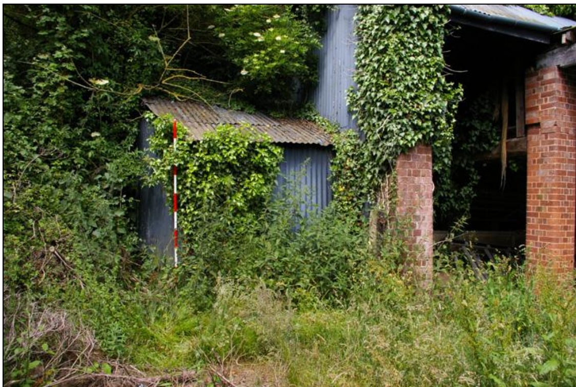
Figure 10: The single storey lean-to at the south-west end of B1, viewed from the south (2m scale).
