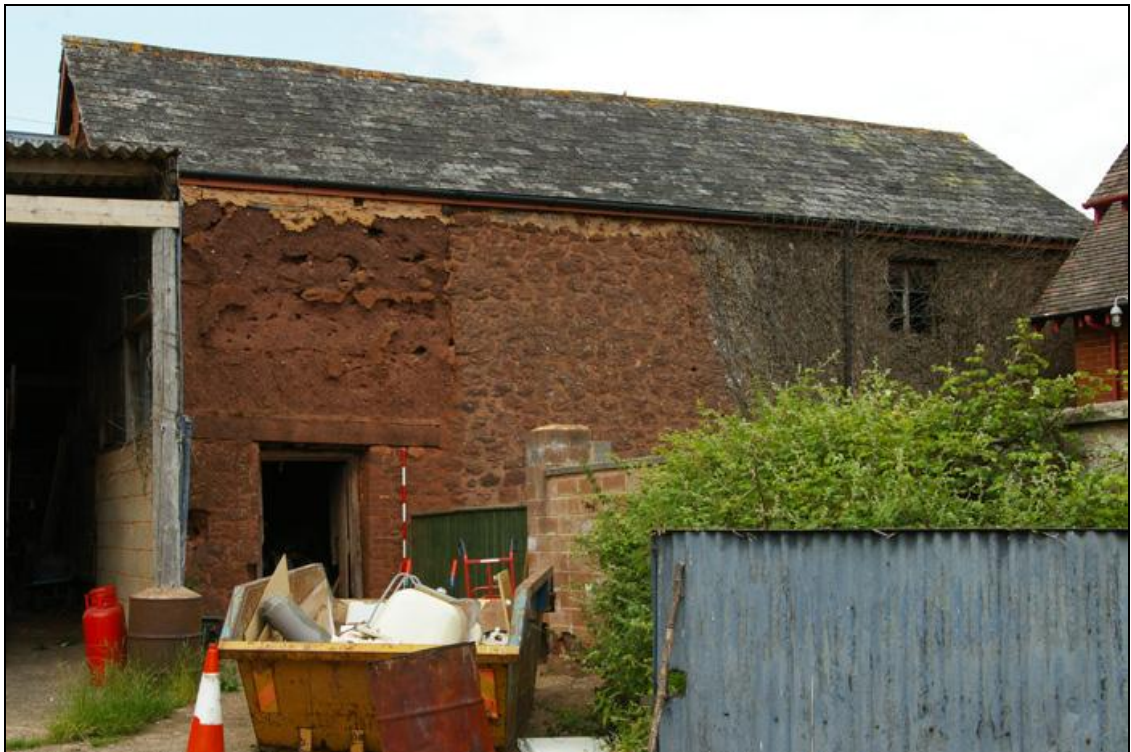
Figure 6: The south-east elevation of Building 1 (B1), viewed from the south (2m scale).
