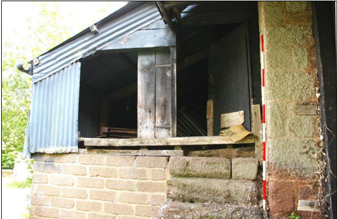
Figure 15: Exterior first floor north elevation of B3a, viewed from the west (2m scale).
