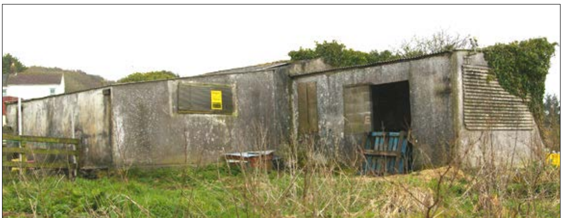
Figure 12: The buildings in the south-west corner of the northern portion of the eastern field, viewed from the north-east.
