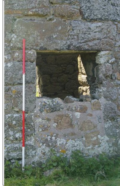
Figure 3: The partially blocked north door opening, viewed from the north (2m scale).
