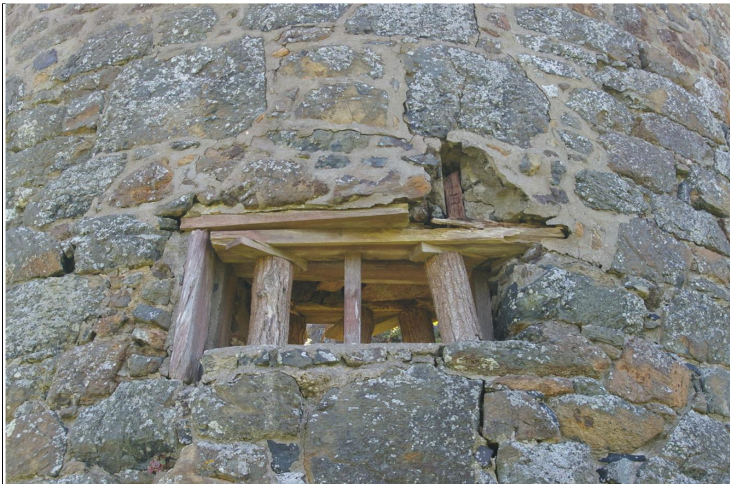
Figure 4: The forced WWII window opening to the north, with modern cement repairs above and to the upper wall, viewed from the north.
