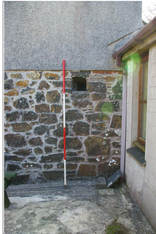
Figure 8: The squint window in the west wall of Windmill Farmhouse, viewed from the west (2m scale).
