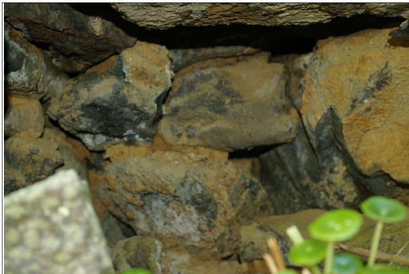
Figure 9: The interior of the cavity within the north-east section of wall, viewed from the south-west. Note the orange earth bonding.
