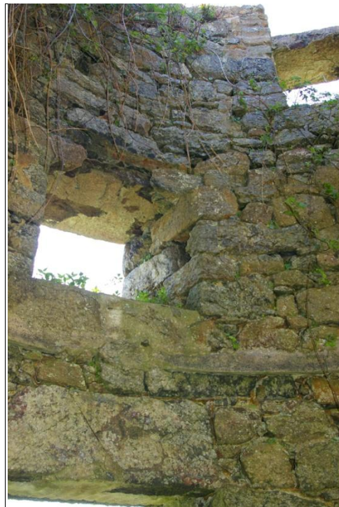
Figure 6: The south window, with cement to the lintel and sill, with cement former floor level below and the west window with (reset?) lintel above.
