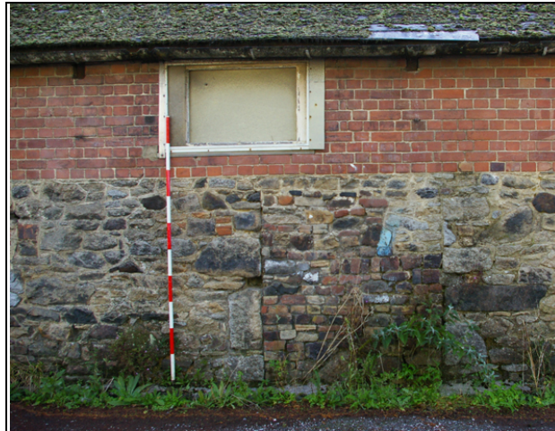
Figure 13: Detail of the blocked door opening, roughly central in the west elevation of the southern part of B1, viewed from the west.
