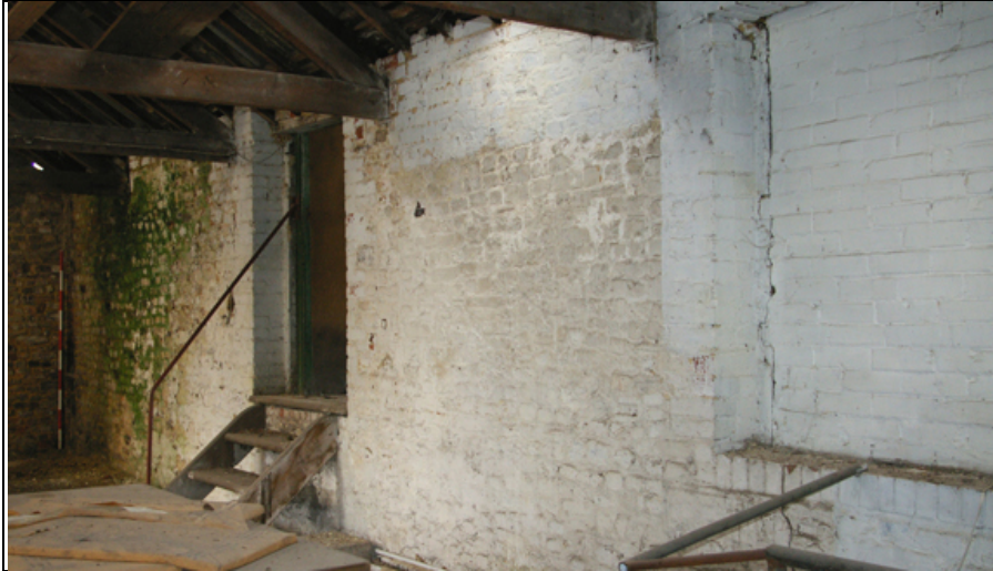
Figure 35: First floor north wall of the southern element of B2, viewed from the east.
