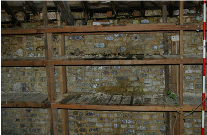
Figure 41: The west end of the interior first floor dividing wall between B2 south & north, viewed from the north.
