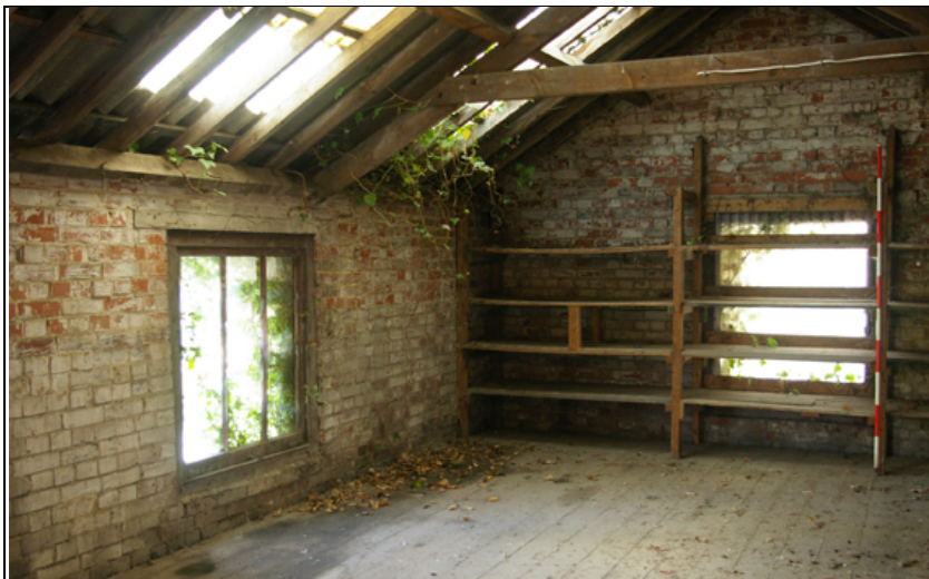
Figure 40: The interior first floor north-east corner of B2 (north), viewed from the west.
