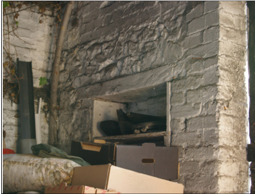
Figure 45: Blocked opening to the east of the door in the south elevation of B1, viewed from the west.
