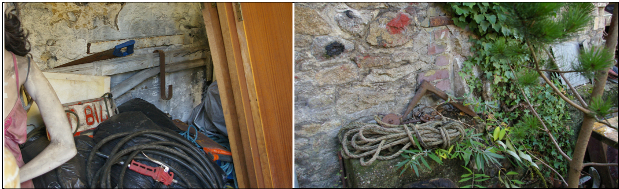
Figure 46: (left) Disturbance and blocked opening in the west end of the north gable wall of B1, viewed from the (interior) SW. Figure 47: (right) As above, exterior, viewed from the north-east.
