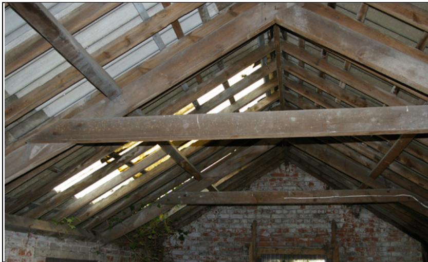
Figure 42: Roof structure over the north element of B2, viewed from the west.
