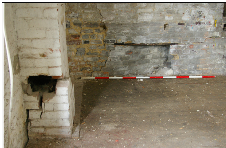
Figure 54: Feature in the first floor east end of the south wall of B2, and internal chimney to the east, viewed from the north.
