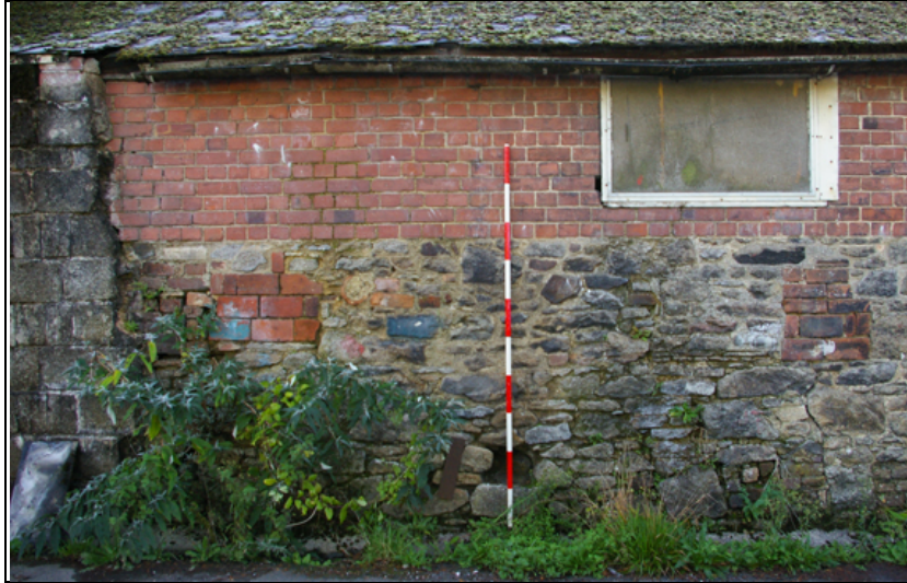
Figure 15: Masonry and blocked openings at the northern end of the southern portion of B1, viewed from the west.
