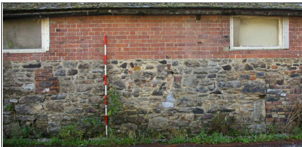
Figure 14: Detail of the blocked openings, in the northern portion of the west elevation of the southern part of B1, viewed from the west.
