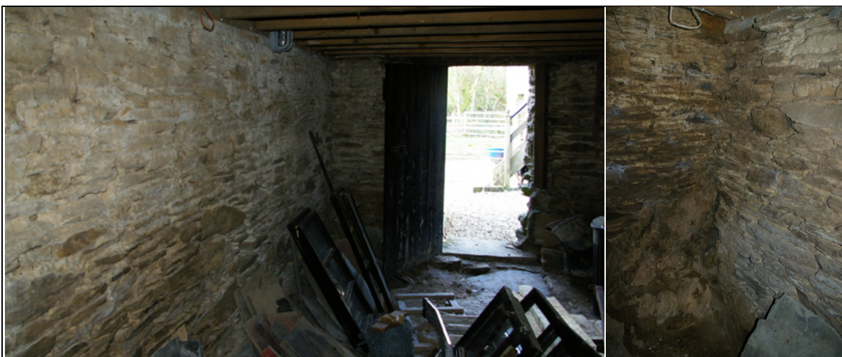
Figure 33: The interior ground-floor south wall of B1, from the east. Figure 34: The interior ground-floor south-east corner of B1 built into the bedrock, from the north-west.
