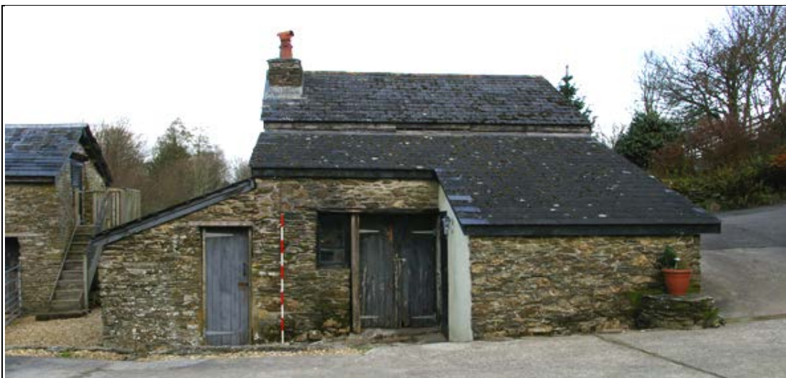
Figure 16: The south elevation of the mill (B1) with lean-tos B1a, B1b & B1c in the foreground, from the south (scale 2m).
