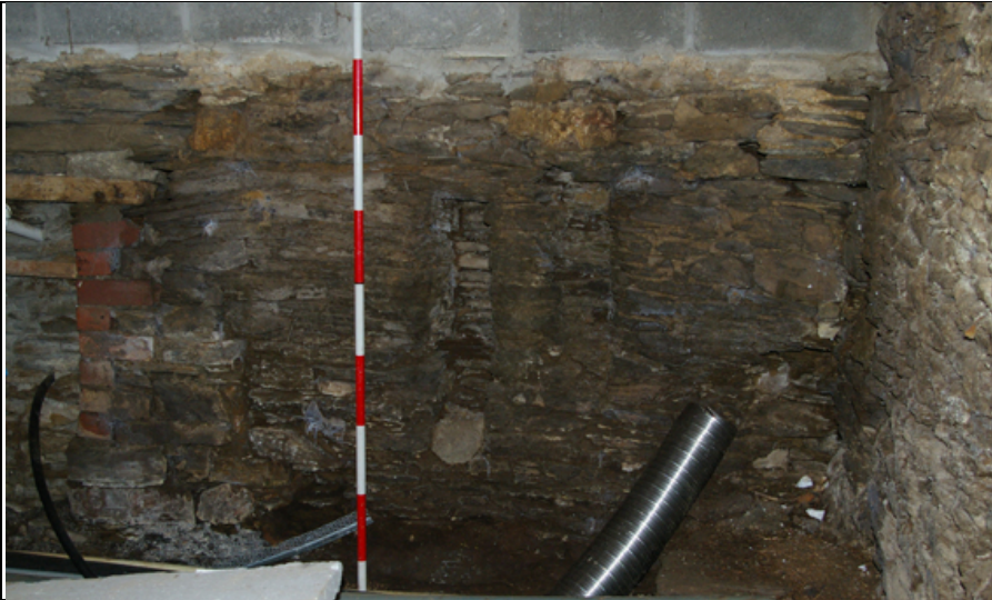
Figure 36: Ground-floor interior north-east corner of B1, with blocked openings; from the south (scale 2m).
