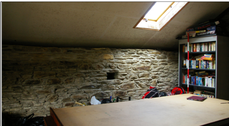
Figure 43: The first-floor interior north wall, with small opening, blocked to the exterior, from the south (scale 2m).
