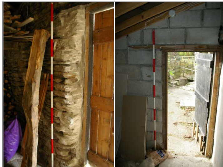
Figure 48: The ragged eastern jamb of the door opening in the south elevation of B1a, from the north-west (scale 2m).
