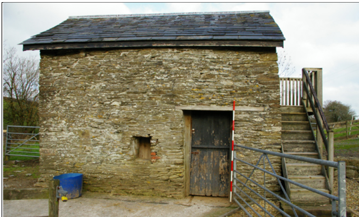
Figure 3: The south elevation of the granary (B2), from the south (scale 2m).
