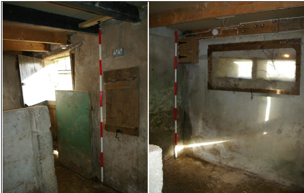
Figure 52: The ground-floor interior south-east corner of B2, from the north-west (scale 2m).
