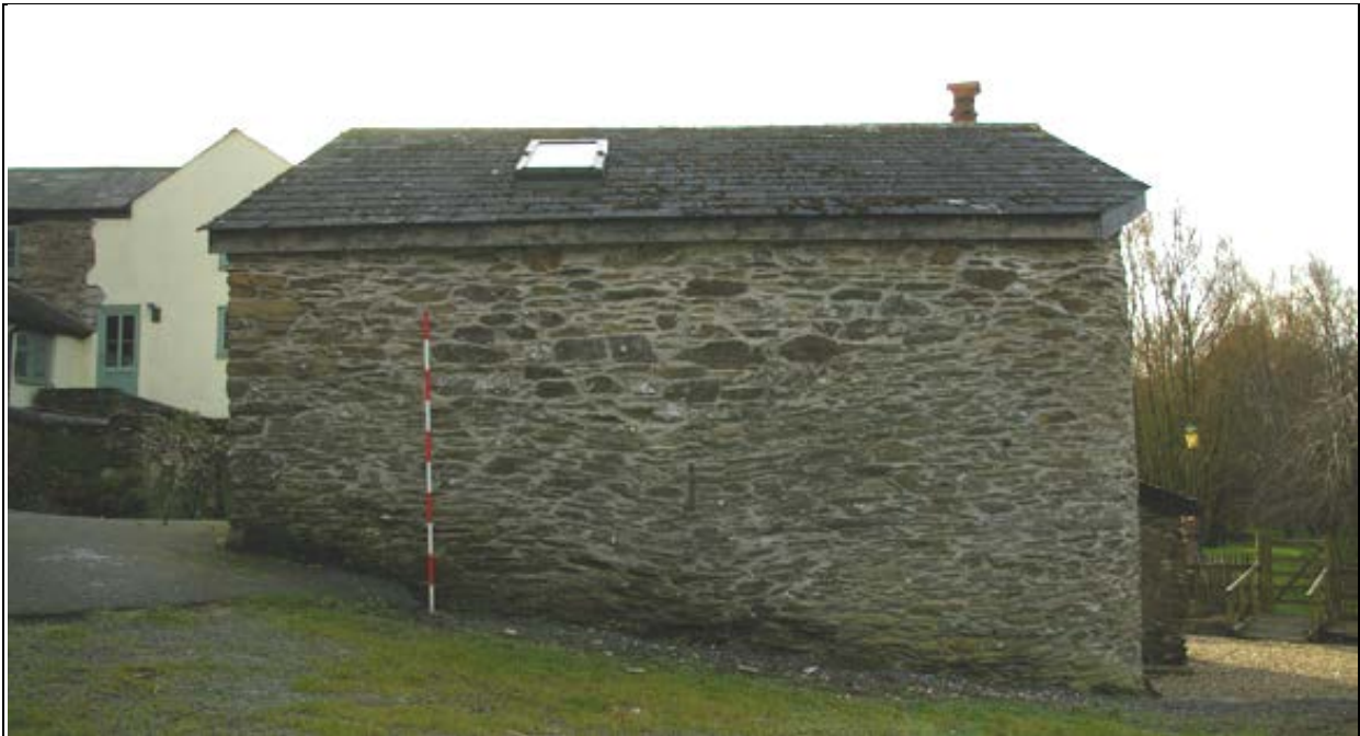
Figure 23: The north elevation of the mill (B1), from the north (scale 2m).
