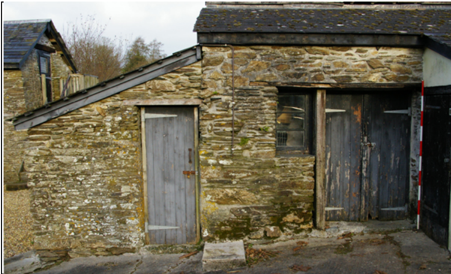
Figure 18: The south elevations of B1a and B1c, from the south (scale 2m).
