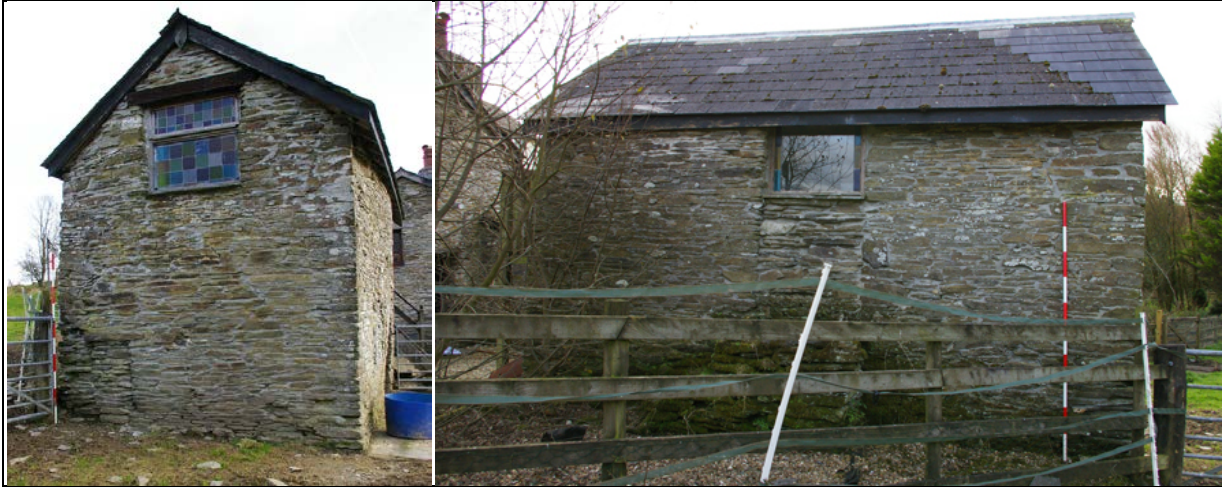
Figure 29: The west elevation of B2, with blocked opening bottom left, from the west (scale 2m). Figure 30: The north elevation of B2, with partly-blocked loading door, from the north (scale 2m).
