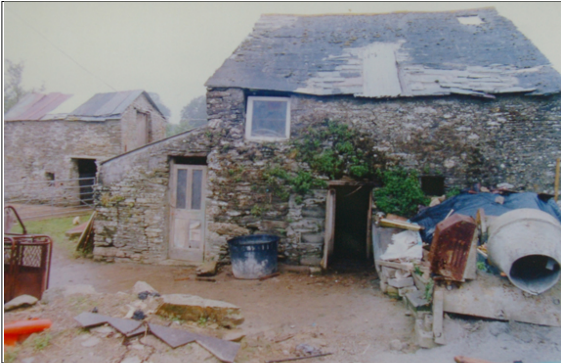
Figure 9: The south elevation of the mill, during the 1990s, with the granary visible on the left.
