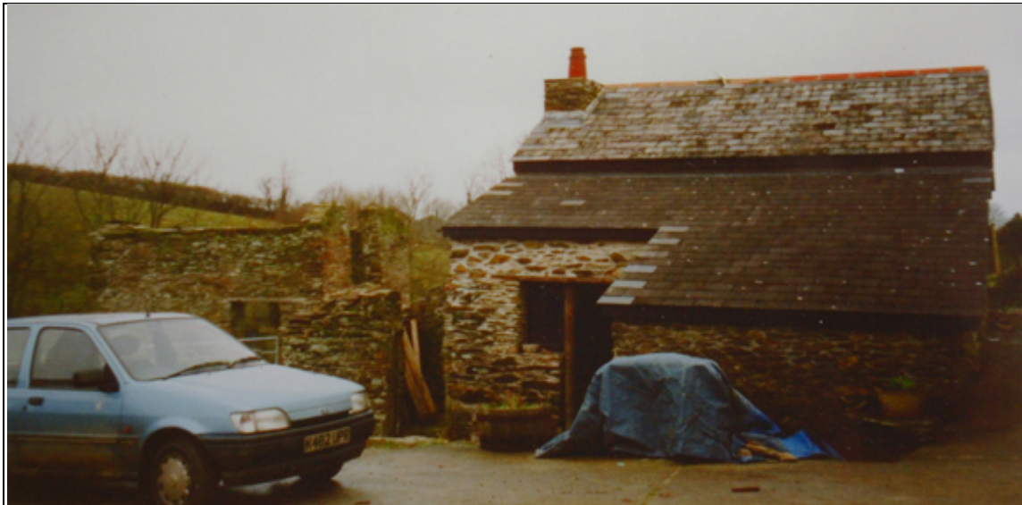
Figure 11: Photograph of the south elevation of the mill dating to 2002, with the roofless granary in the background to the west.
