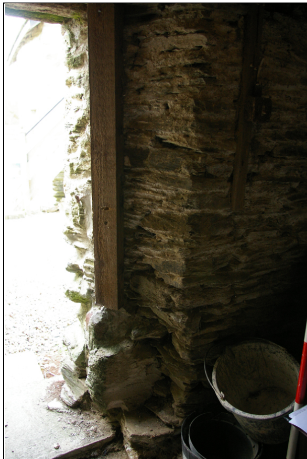
Figure 40: The ragged northern jamb of the ground-floor door opening in the west elevation of B1, from the south-east.
