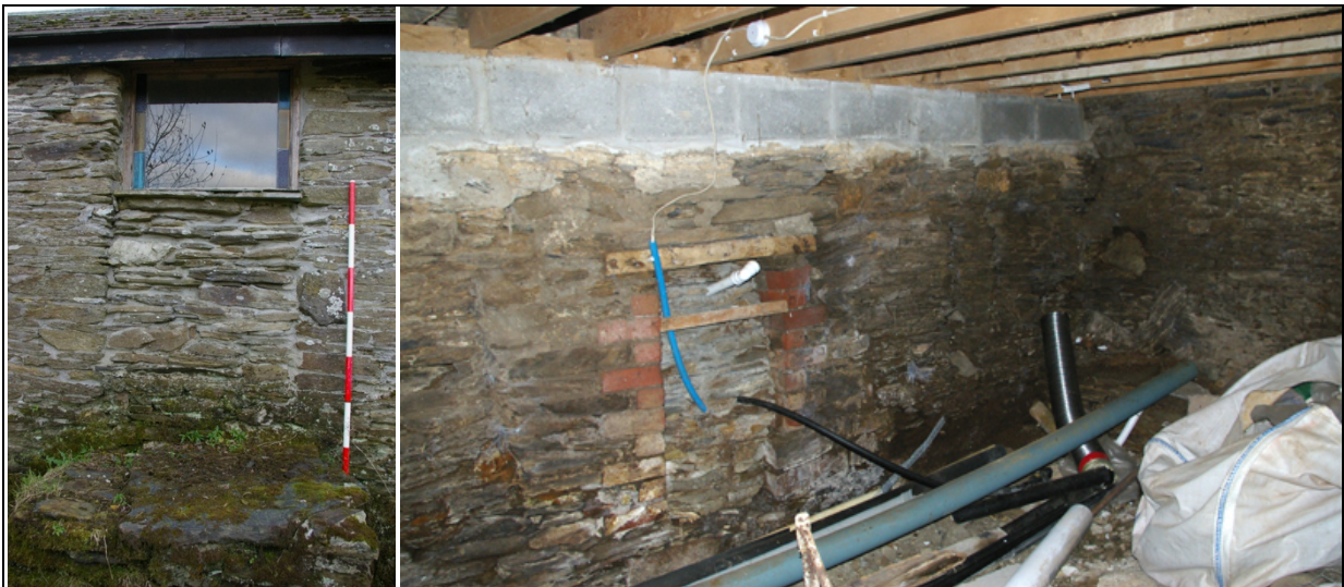
Figure 31: Detail of the blocked opening in the north wall of B2, from the north (scale 2m). Figure 32: The interior ground-floor north wall of B1, with blocked opening, from the south-west.
