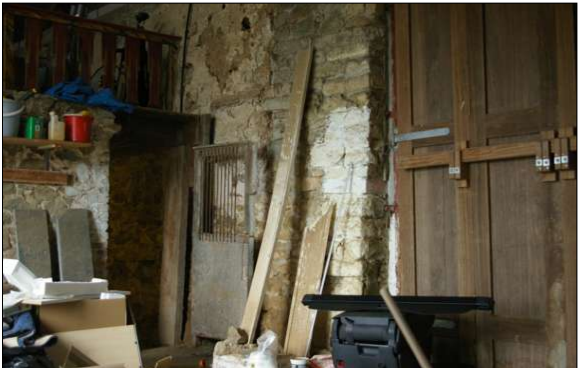
Figure 21: The cob portion of the north wall of the barn and north end of the single storey internal wall, viewed from the south-east.
