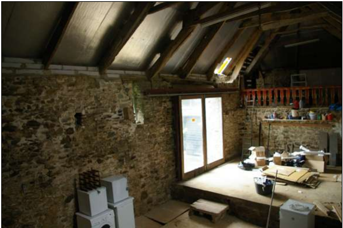
Figure 23: The south wall of the barn and western single story partition, viewed from the north-east.
