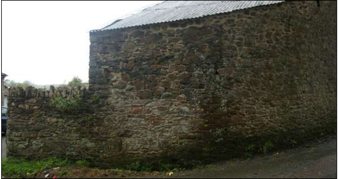
Figure 14: The polygonal north/east wall of the lean-to, the lower portion of the wall is of a continuous build to the gate pier, viewed from the north-east.
