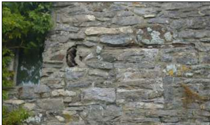
Figure 8: Detail of the blocked opening in the south wall.
