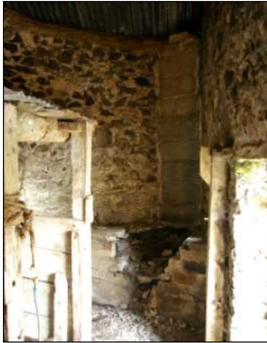
Figure 16: The copper in the south-east corner of the lean-to, viewed from the west.
