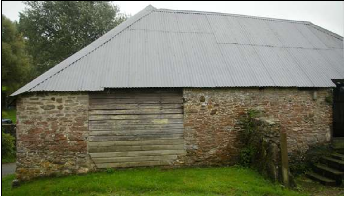
Figure 11: The north end of the west elevation of the barn and linhay, viewed from the south-west.
