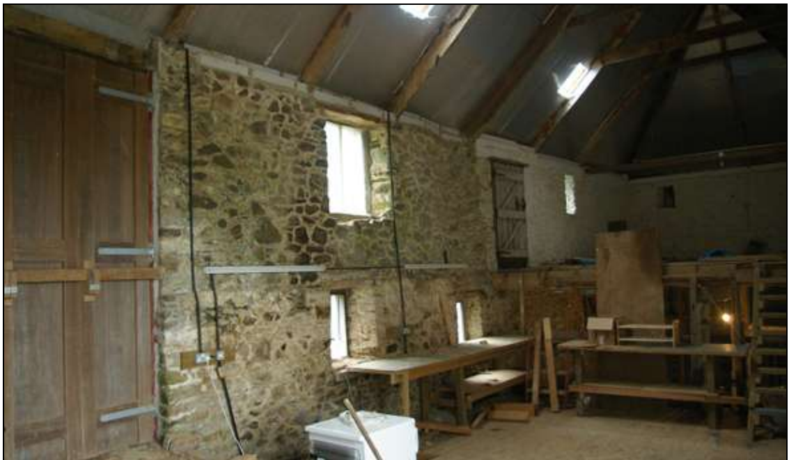
Figure 19: The eastern portion of the north wall of the barn, viewed from the south-west.
