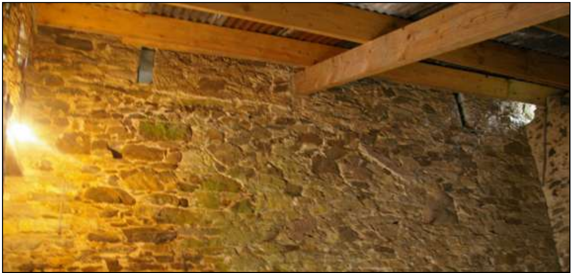
Figure 15: The west wall of the lean-to, with scars of a former roof line, viewed from the east.
