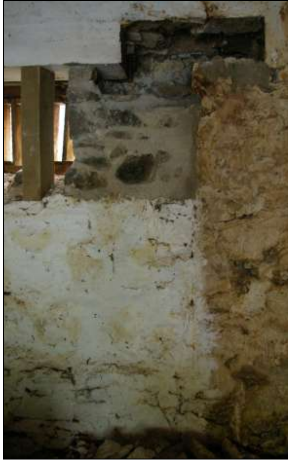
Figure 25: The partially blocked opening in the west wall of the Linhay, viewed from the east.
