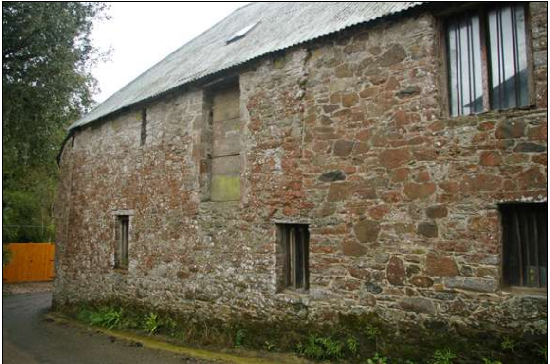
Figure 13: The east end of the north elevation of the barn, showing the clear joint in the masonry, viewed from the north-west.
