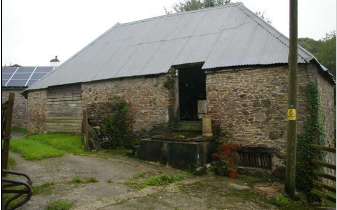
Figure 10: The west elevation of the linhay at the west end of the barn, viewed from the south-west.
