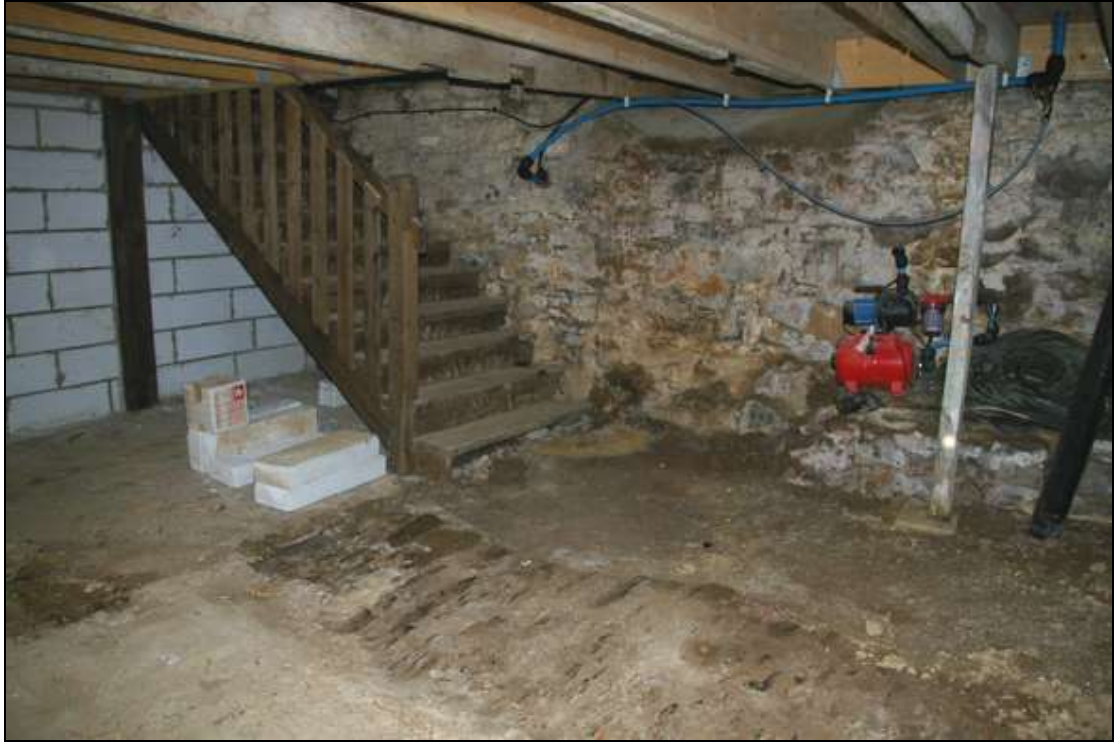
Figure 22: The west wall and north-west corner of the ground floor western element of the barn, viewed from the north-east.
