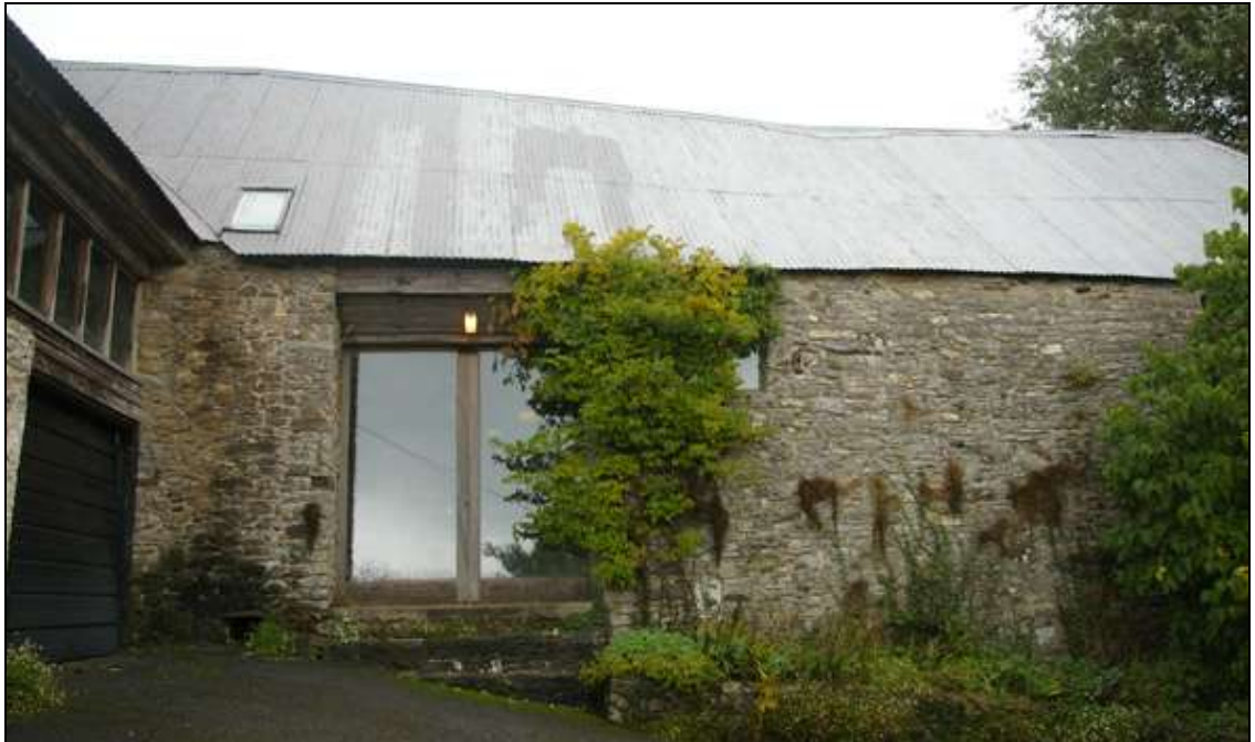
Figure 7: The central western portion of the barn with the southern threshing doors, viewed from the south.
