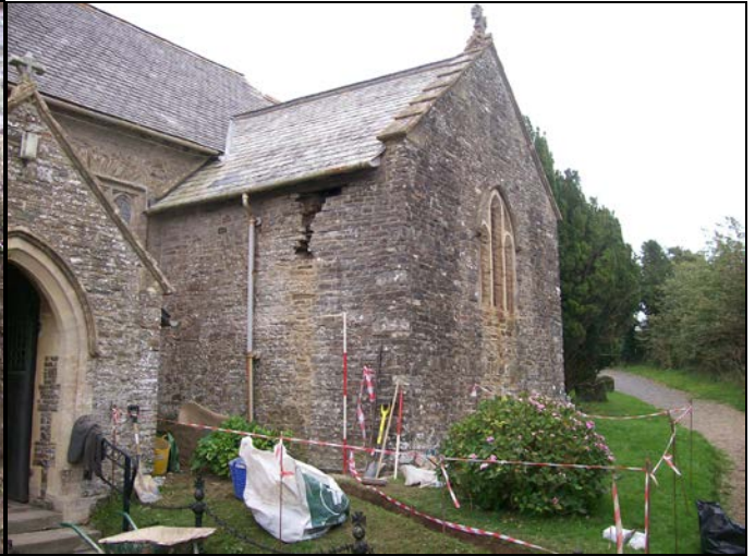
Figure 2: South transept; showing crack, repair and pipe trench, viewed from the south-west (2m scale)
