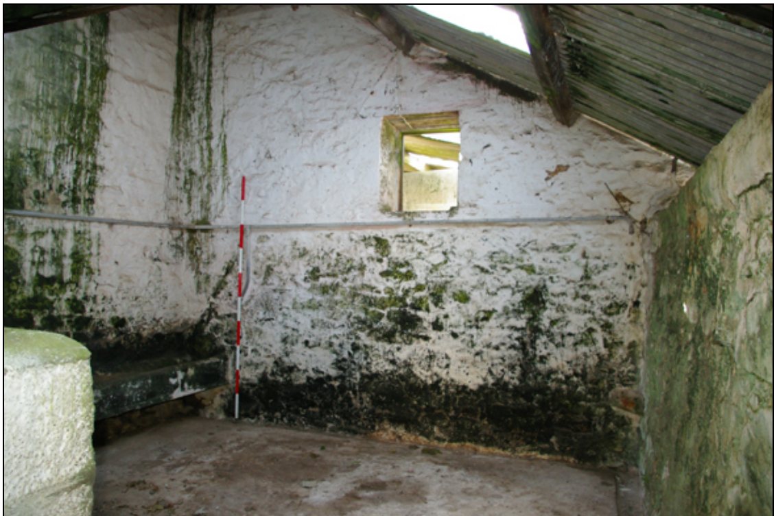
Figure 17: The interior of the south wall of B1b, viewed from the north.
