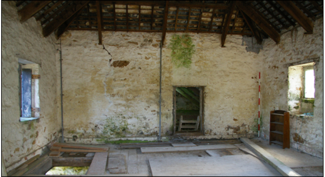
Figure 12: The eastern end of the first floor of B1, viewed from the west.
