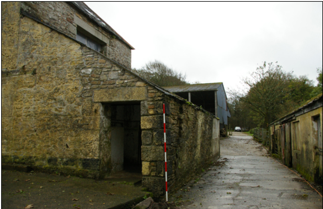
Figure 16: Lean-to (B1b) against the west wall of the chall barn (B1), viewed from the north.
