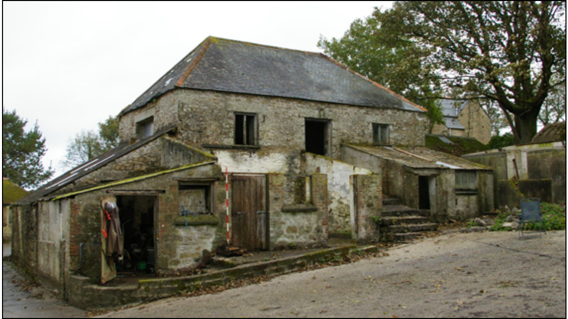
Figure 8: The south (rear) elevation of the main chall barn (B1), with later associated structures (and the former farmhouse in the background), viewed from the south-west.
