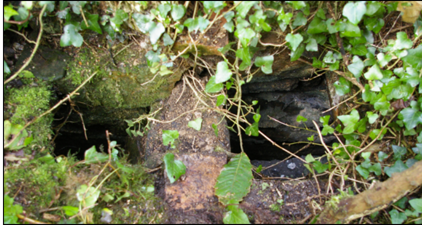
Figure 22: The flue from the fireplace in the east wall of B2a, showing smaller flue leading up from the south, now blocked, viewed from the east.
