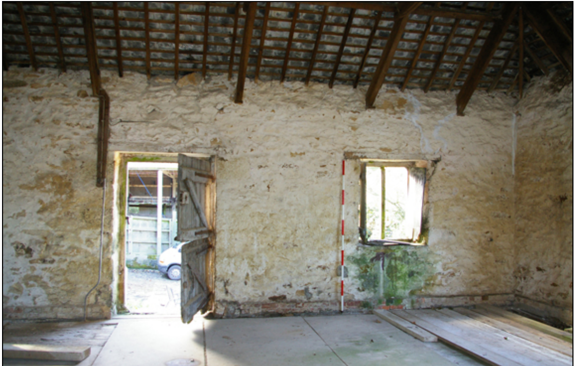
Figure 11: The western portion of the first floor south elevation of B1, viewed from the north.
