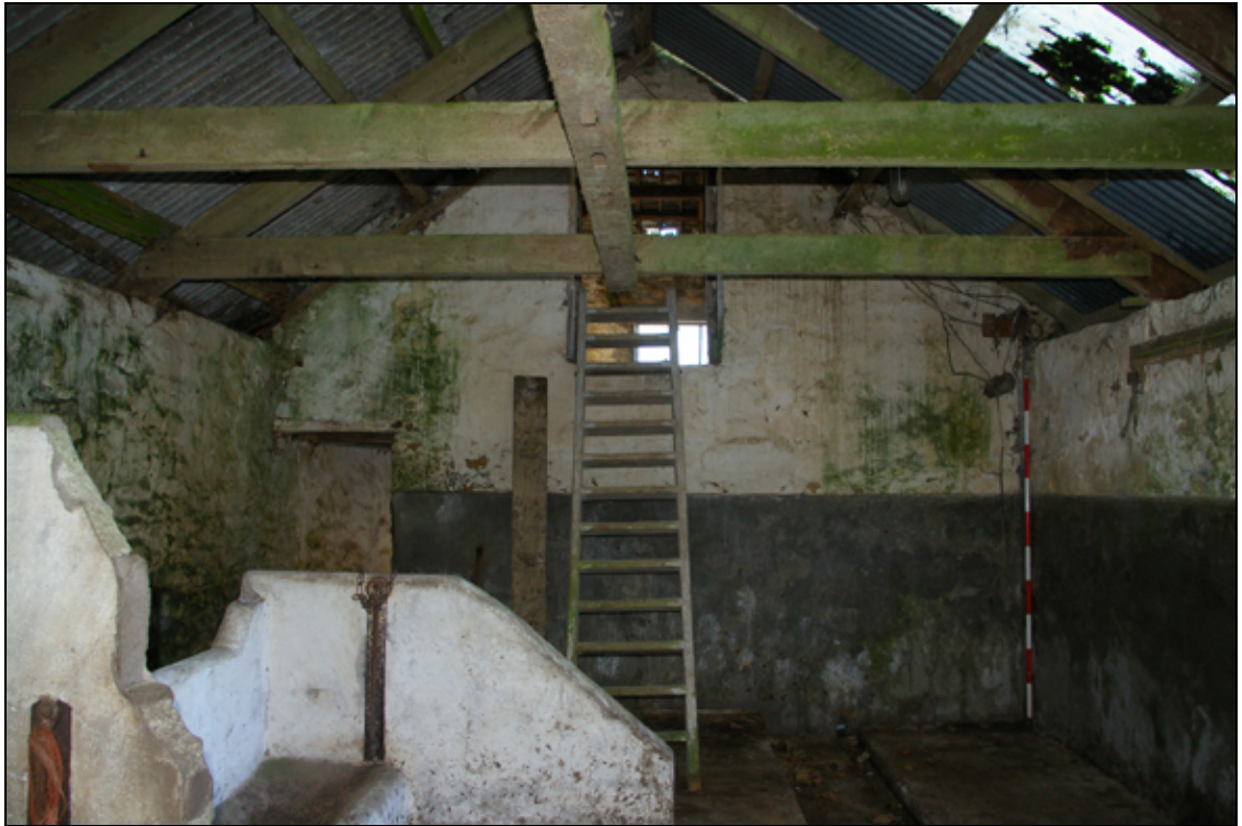
Figure 15: The west wall of B1a (east wall of B1), with original loading door and forced door opening in the south-west corner, viewed from the east.
