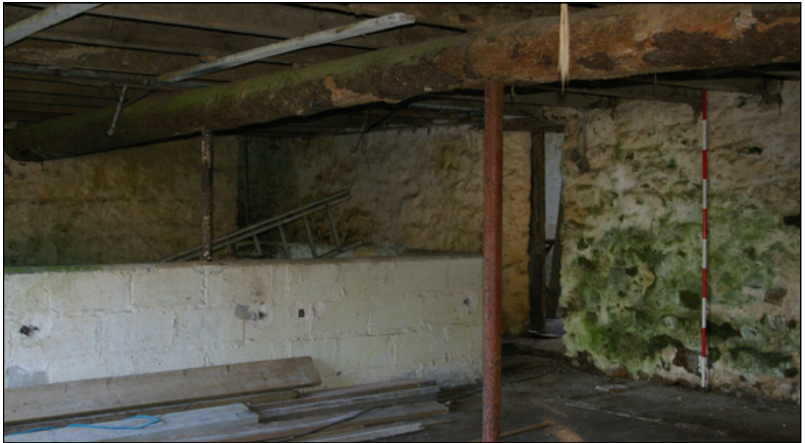
Figure 9: The south-east corner of the ground floor of B1, viewed from the north-west.
