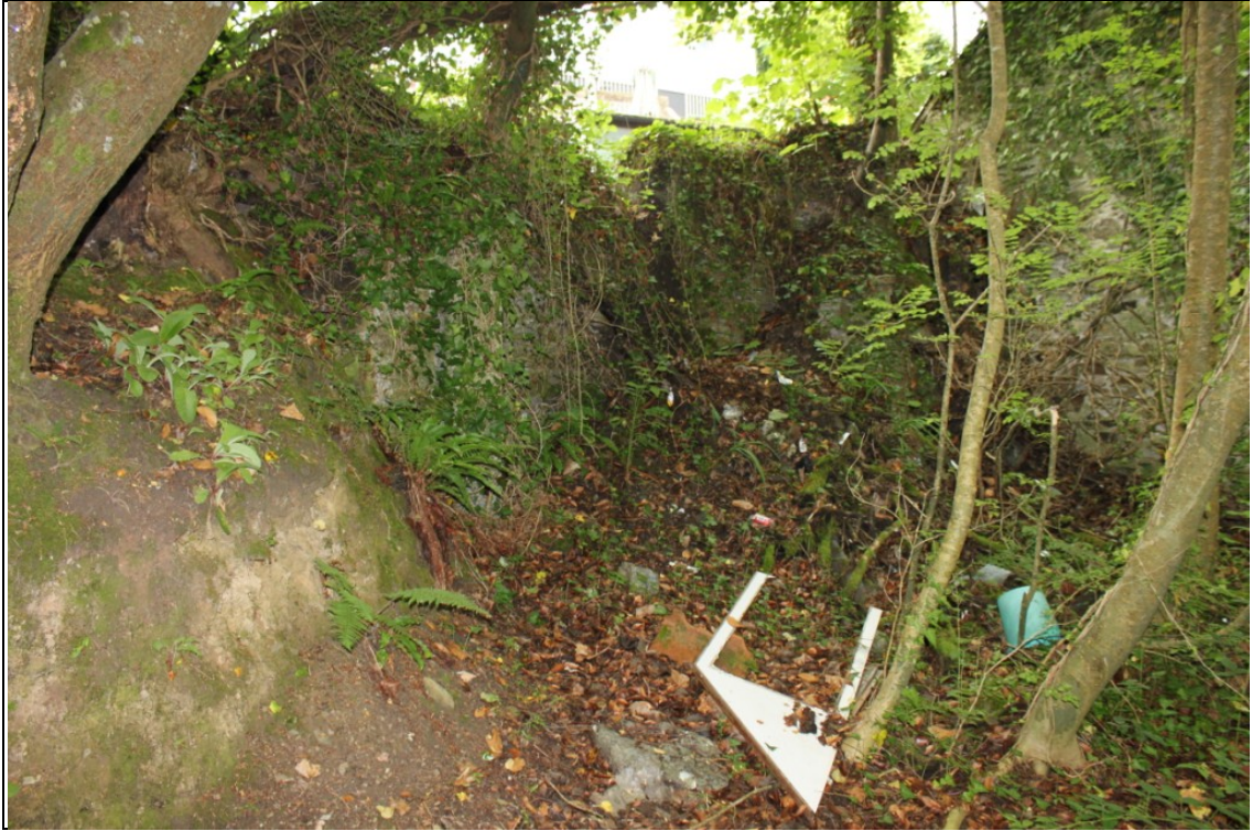
Figure 21: Blocked former opening to the east of the garage, viewed from the northeast.
