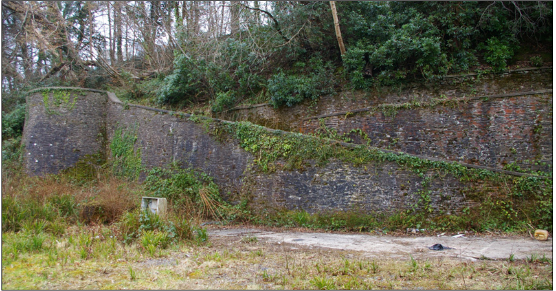
Figure 24: The tiered retaining walls and viewing platform tower to the east of the house, viewed from the north-west.
