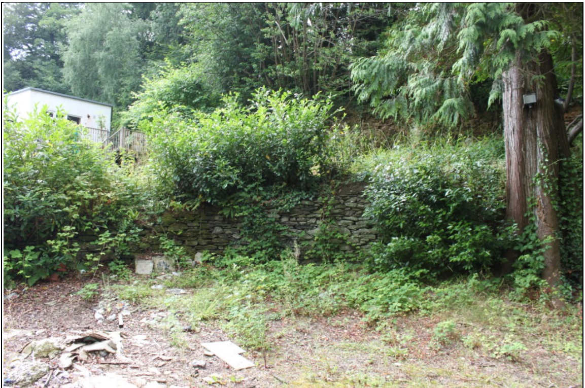
Figure 14: Stone retaining wall along the eastern edge of the southern edge of the oval platform to the west of the house, viewed from the north.
