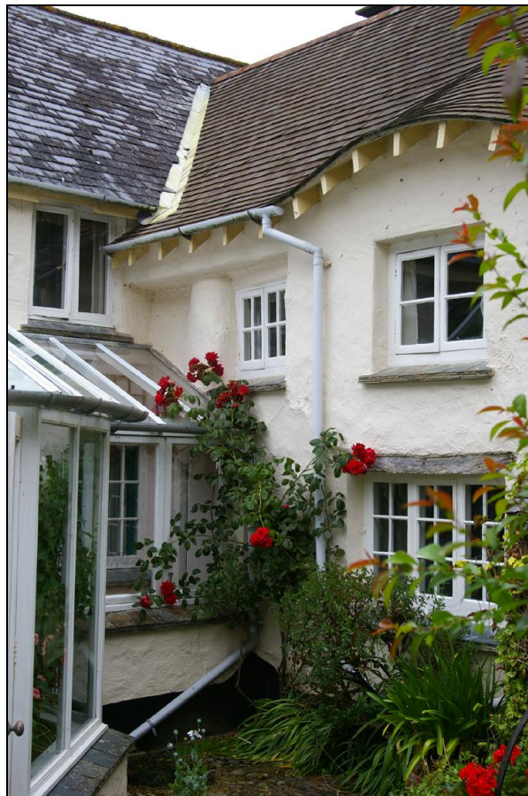
Figure 13: The angle between the front range and the rear north-east wing showing the possible position of the stair turret; viewed from the rear yard (the south-east).
