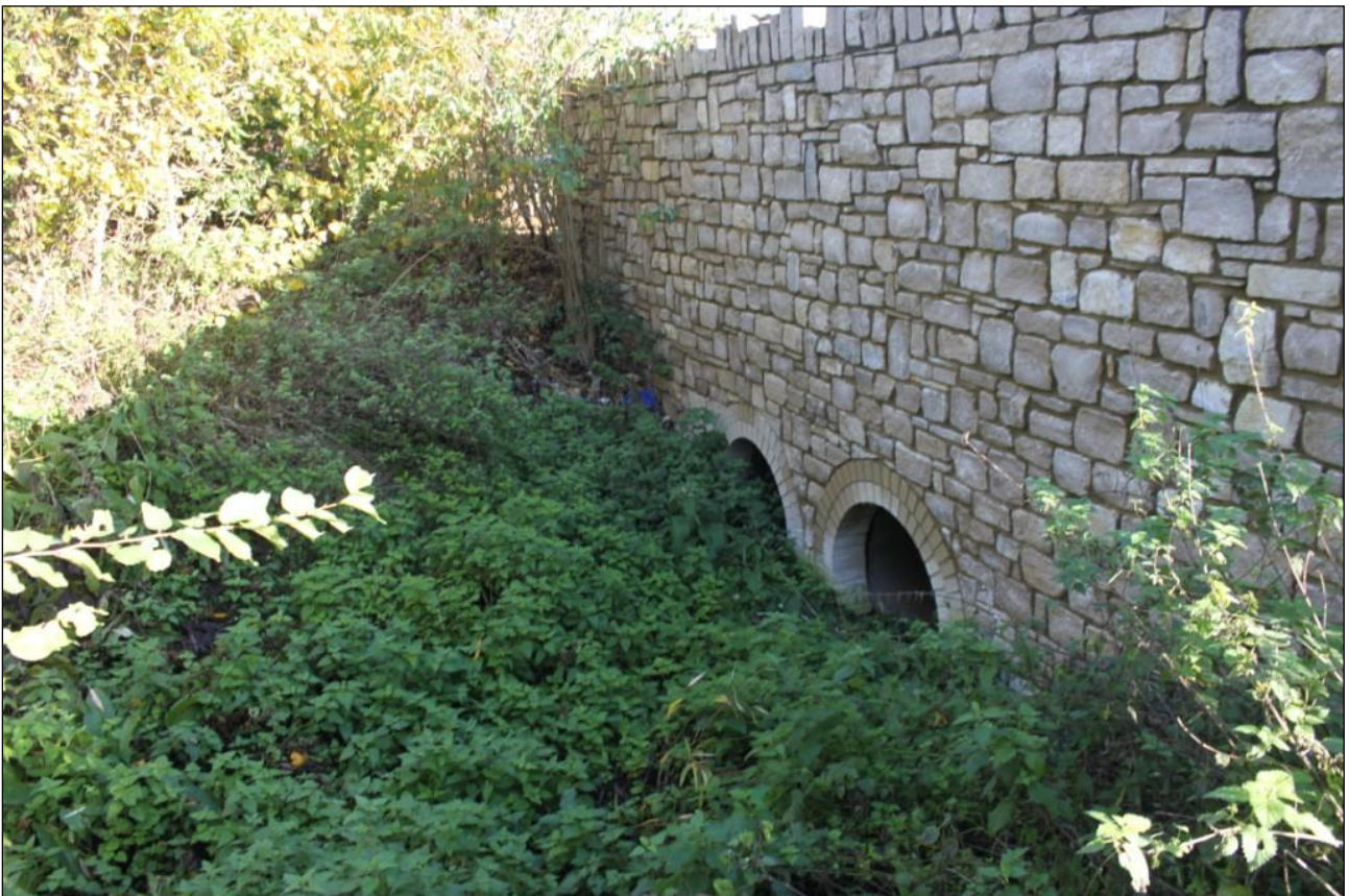
Shot of the 'new' culvert accessing the site from the Park and Ride- viewed from the south-south-east.
