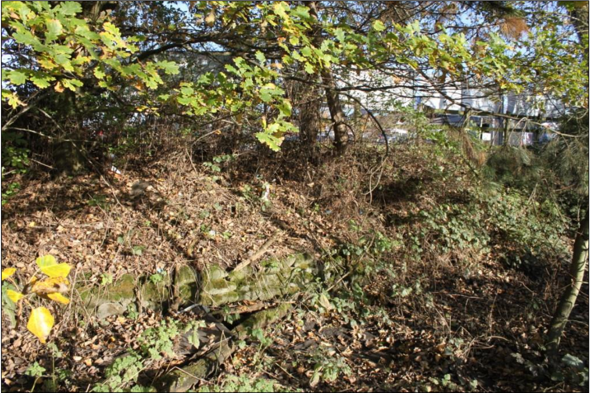
Figure 15: Shot from the drainage ditch showing the short length of stone facing to the embankment along the northern edge.
