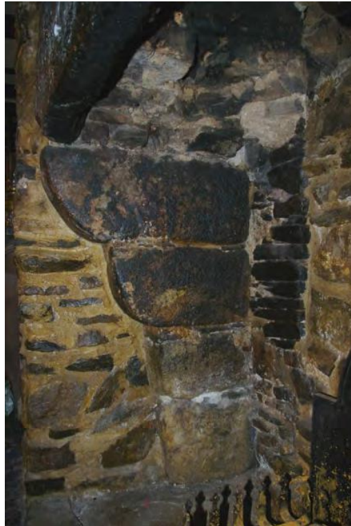
Figure 9: Detail of the corbels to the west of the opening within the fireplace in room G2, from the west.
