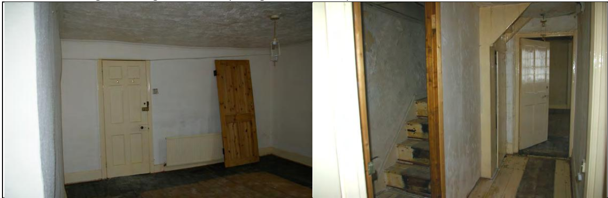
Figure 51: The interior W wall of bedroom F2 with sloping timber at wall top, from S-E.
