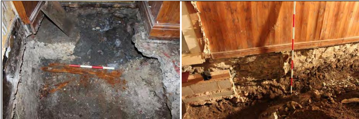
Figure 73: Remnant of timber against threshold of opening into G3, from S. Figure 74: Change of build in west elevation of the G4, from E.
