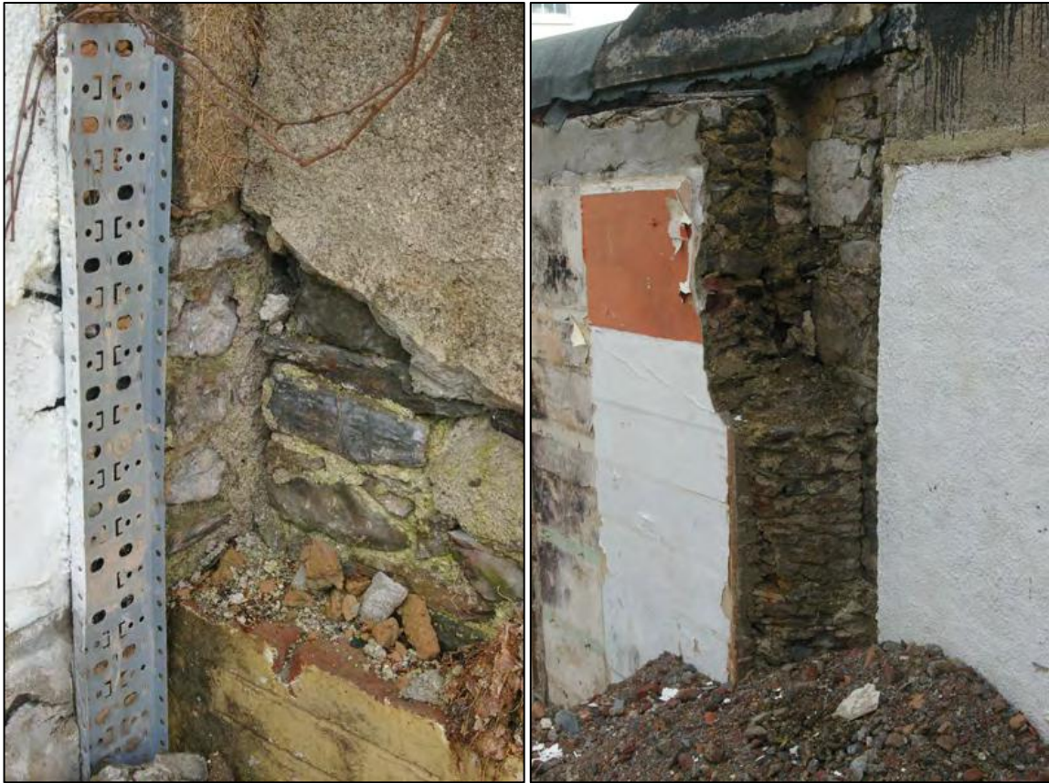
Figure 28: Build of east wall of kitchen/hall (G8/G1) abutting east wall of G7, viewed from south-west. Figure 29: Kink in wall of south elevation, in south-west corner of G7), viewed from the north-east.
