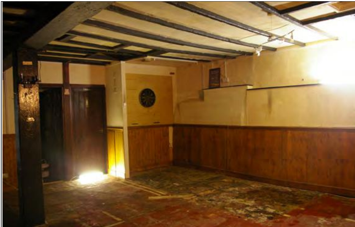
Figure 12: The south-west corner of room G4, with irregular west wall and toilet block to the west, from the north-east.
