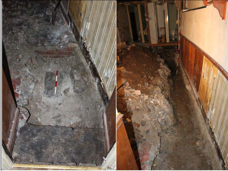
Figure 71: Dwarf wall noted in sewer trench in G4, from N. Figure 72: Fully excavated sewer trench as above.
