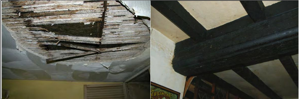
Figure 63: Left: Lathe and plaster ceiling in S-E corner of S5, from the N-W.
