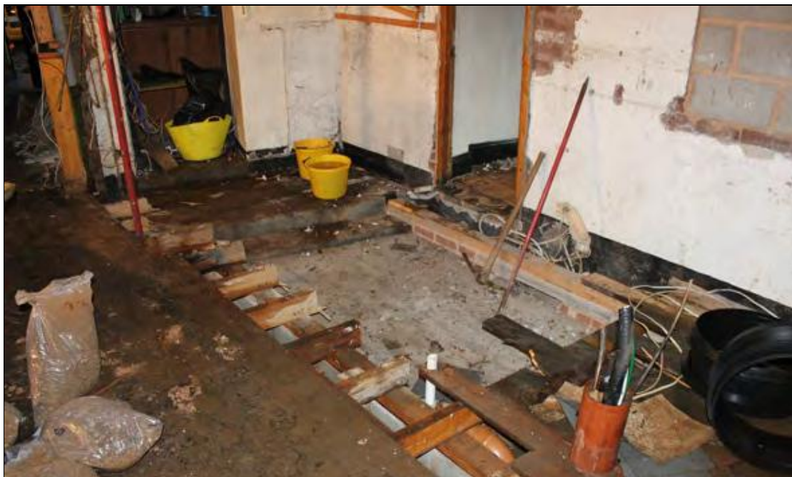
Figure 18: The removed bar area in the north-west corner of G4, from the south-west.
