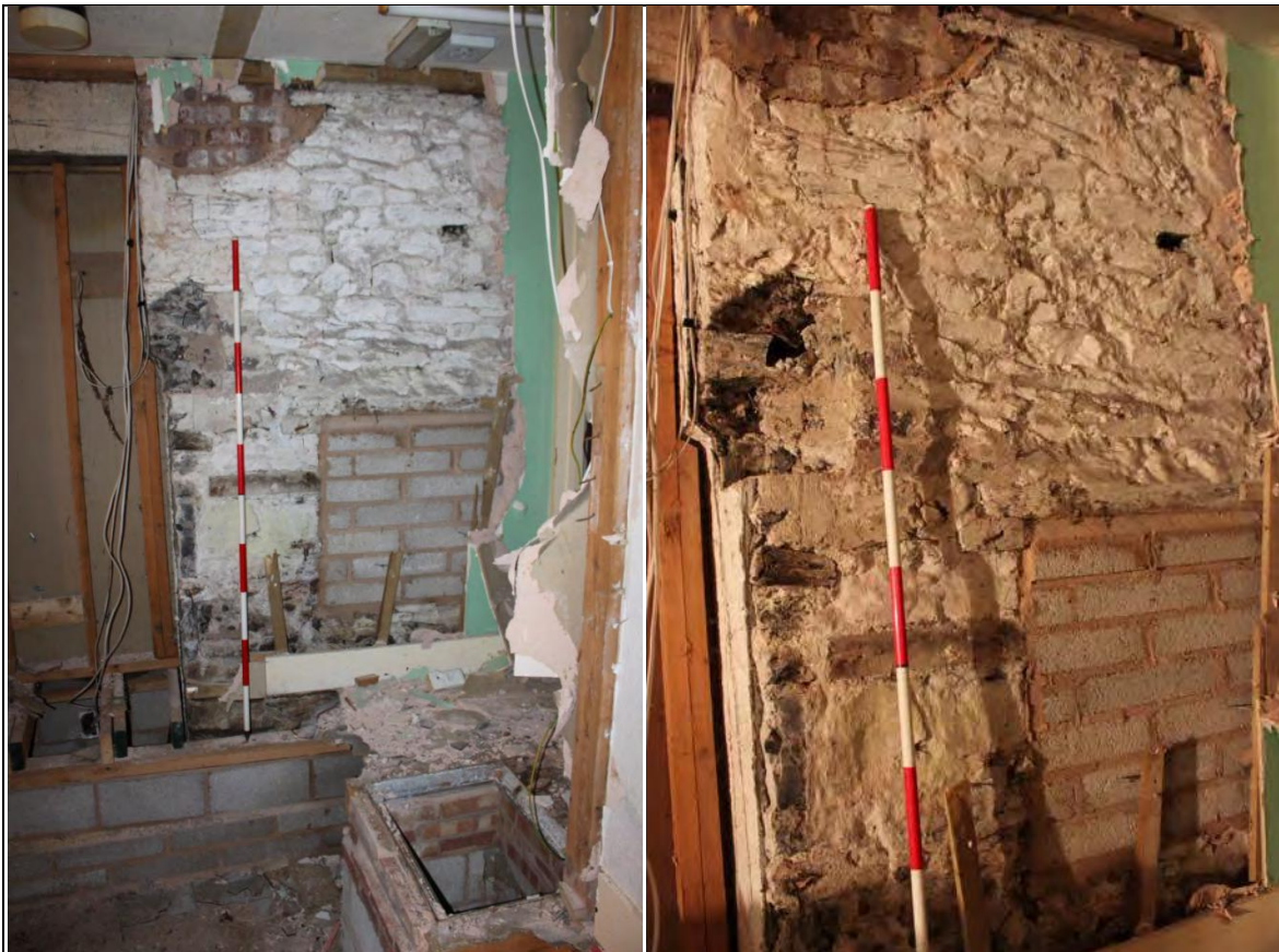
Figure 77: Left: E wall of toilet block G5, from N-W. Figure 78: Right: close up of above.
