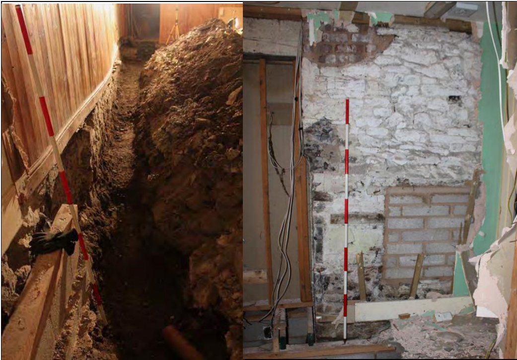
Figure 16: Sewer trench in G4, showing change in the build of the west wall, from the south.
