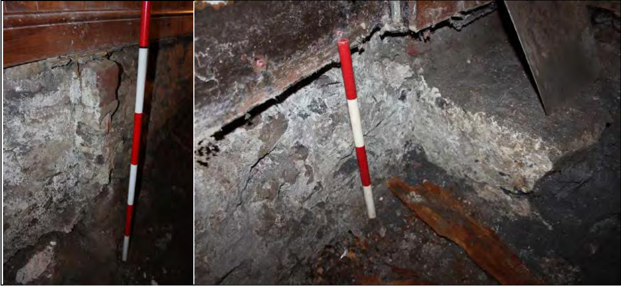
Figure 75: Left: close up of change of build in W wall of G4, from S-W. Figure 76: Right: W wall of G4 abutting G3 N-W corner, from S-E.
