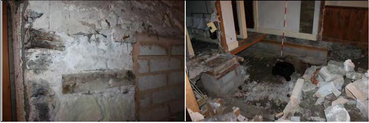
Figure 79: Detail of timber lacing in W wall of former toilet block G5, from N-W.
