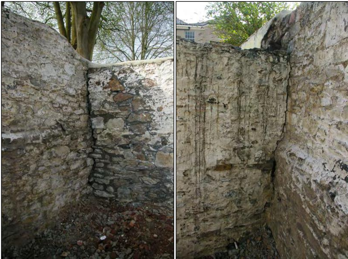
Figure 26: Abutting wall in south-west corner of toilet block (G5), viewed from the north-east.
