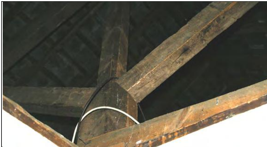
Figure 65: Kingpost roof truss located above and between rooms S3 & S4, from the W.
