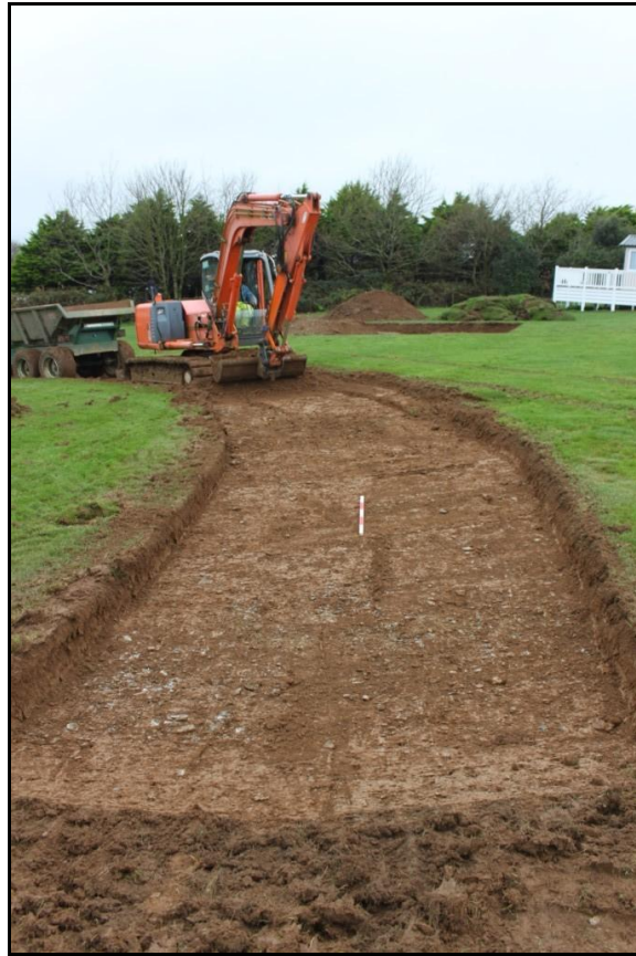
35. THE WESTERN PART OF THE ACCESS ROAD; VIEWED FROM THE EAST (1M SCALE).
