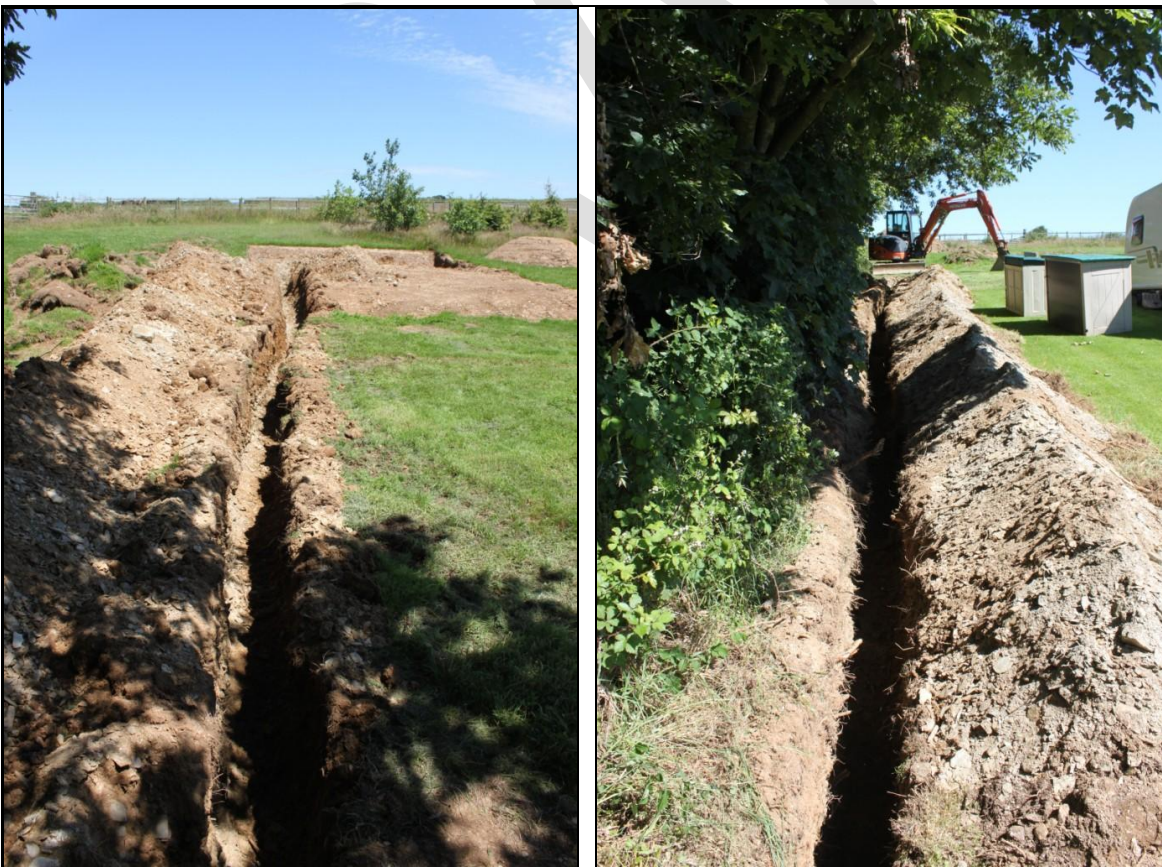
14. LEFT: POST-EX OF NORTHERN END OF SERVICE TRENCH FOR PLOT A; VIEWED FROM THE SOUTH-WEST (NO SCALE).
