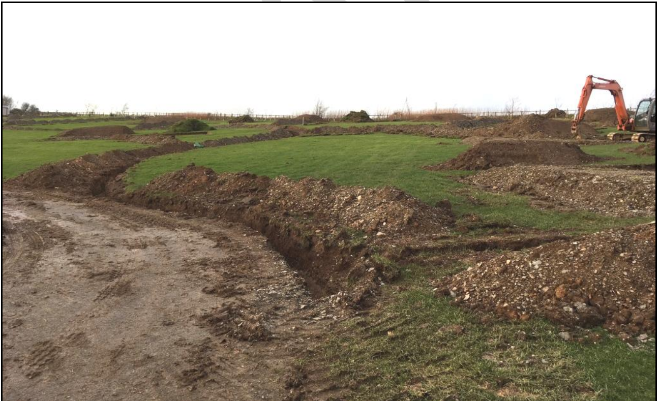
36. THE SITE, POST-SERVICE TRENCHING, FROM SOUTH OF PLOT J; VIEWED FROM THE SOUTH-EAST (NO SCALE).
