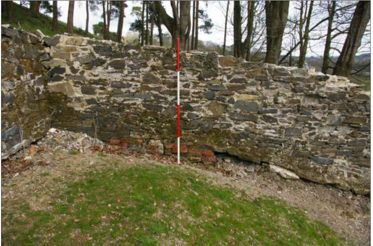
The north-east corner of the yard wall, showing infill brickwork and undermined walling; from the west (scale 2m).
