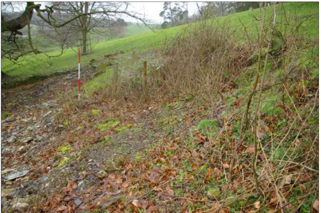
View along the bank where the north elevation has collapsed, from the east.
