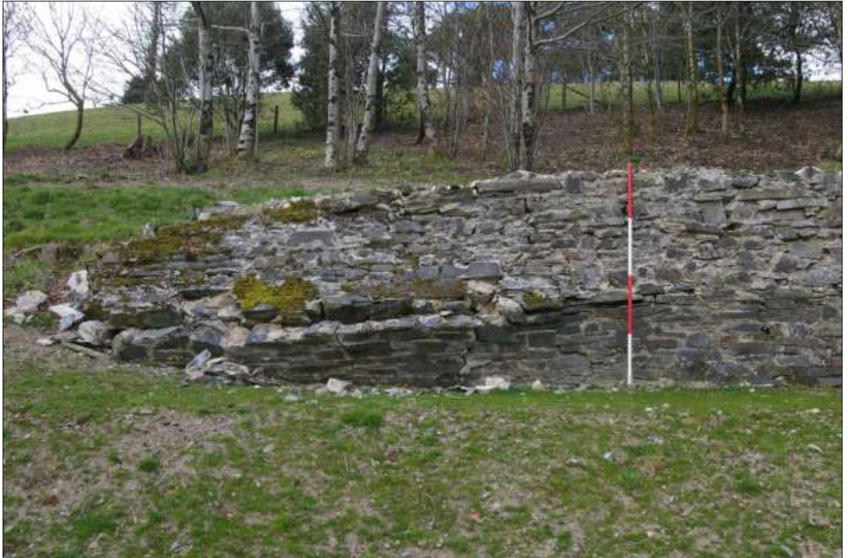
As above, the eastern end, showing the wall collapse; viewed from the south (scale 2m).
