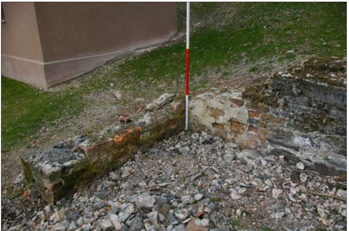
The building in the south-east angle, the internal corner, showing brickwork facing; from the south-east (scale 2m).
