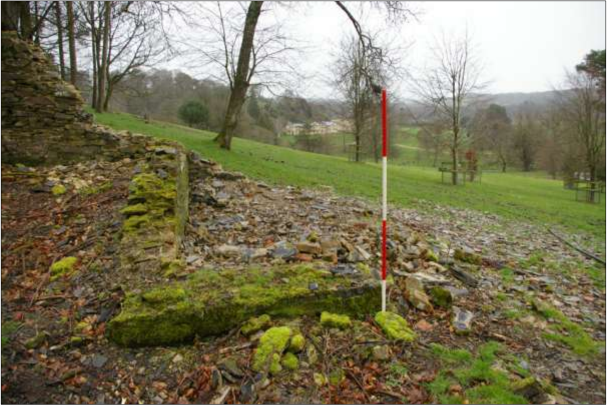
The walls of the small interior room abutting the east and south elevations, from the west.
