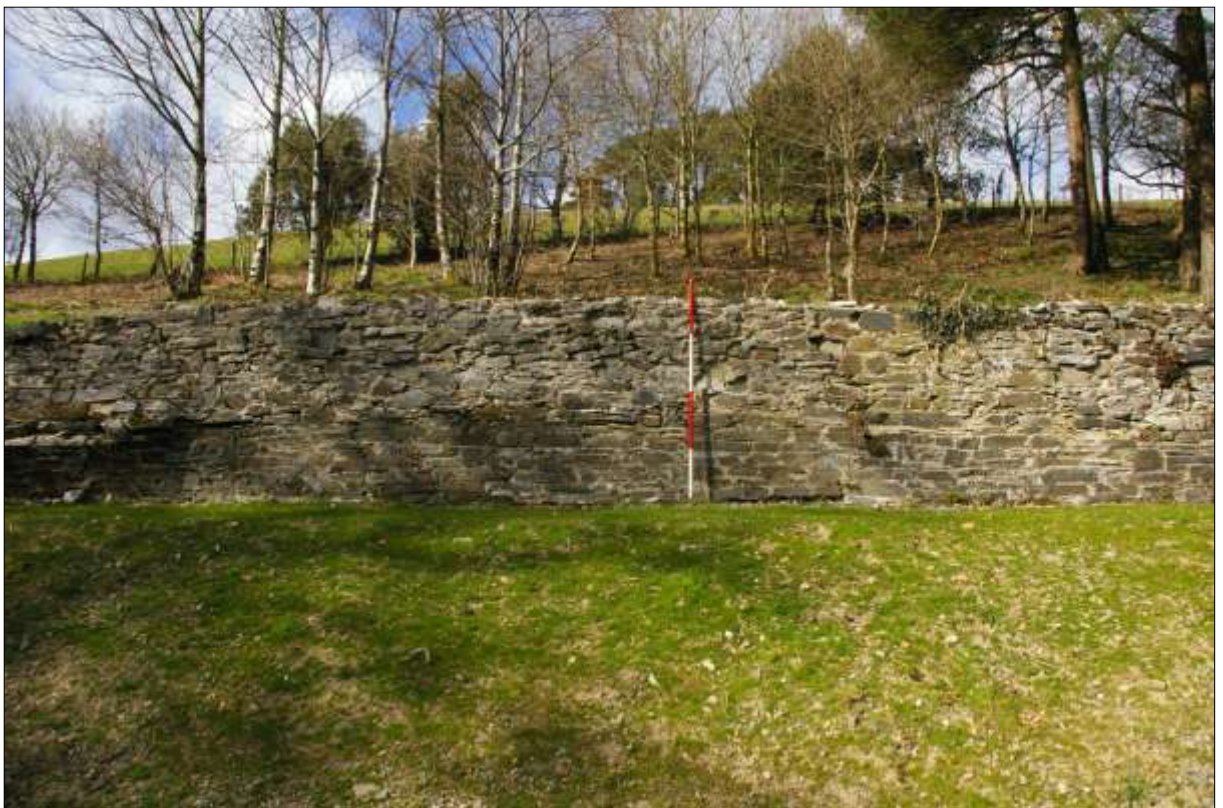
The south-facing elevation of the north wall of the yard; viewed from the south (scale 2m).
