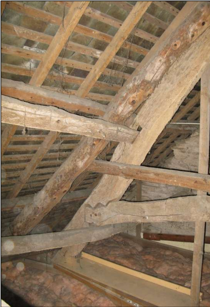
Figure 77: Detail of failing Truss H; viewed from the north-west.
