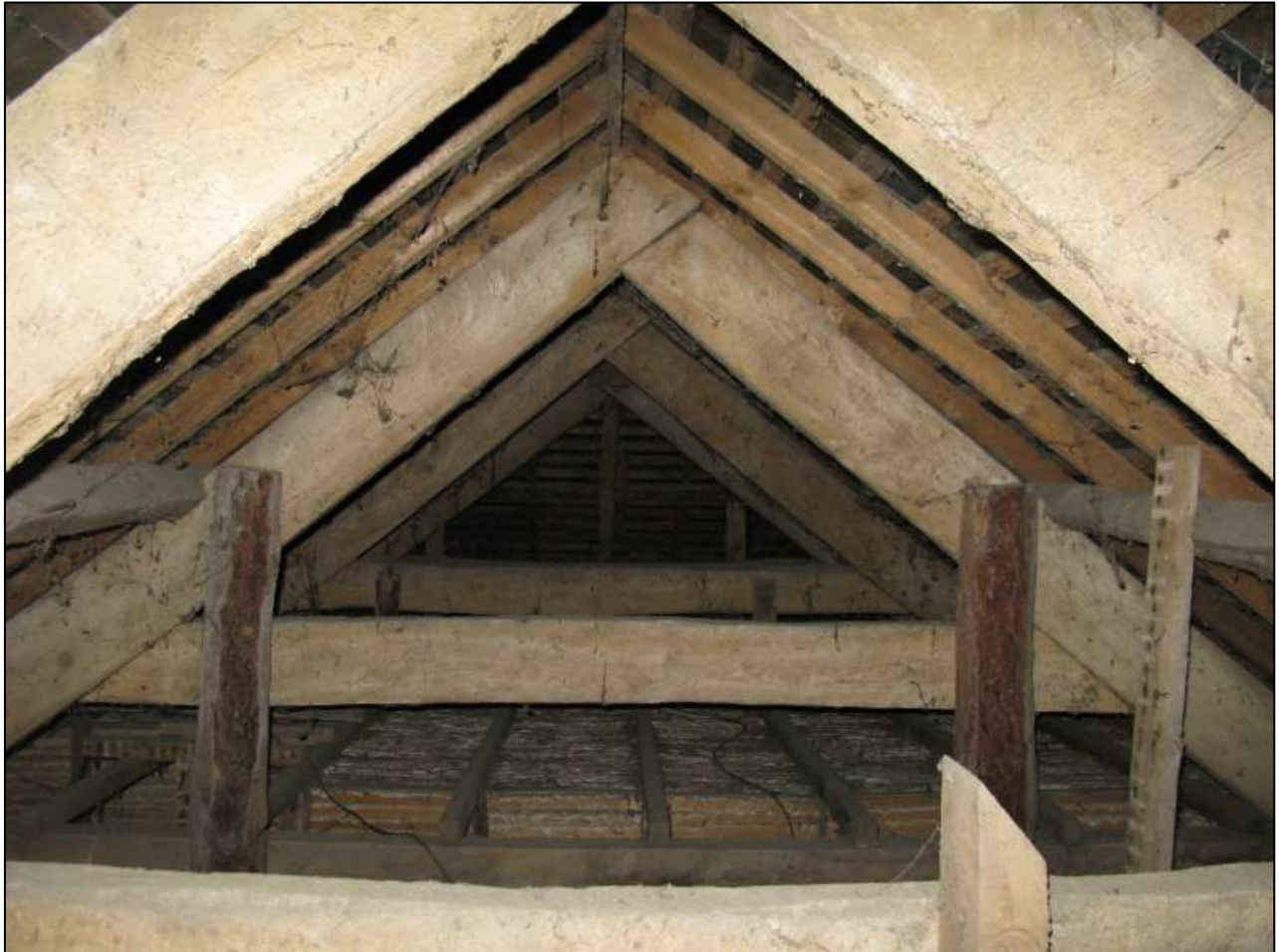
Figure 83: The 19 th century roof trusses in the 19 th century block; viewed from the west.
