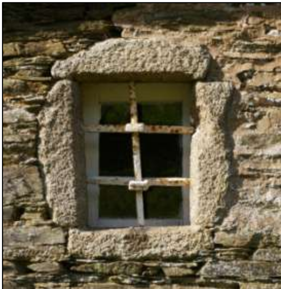
Figure 59: The single surviving original window in the southern elevation. Note the chisel marks on the knuckles of the ferramenta .
