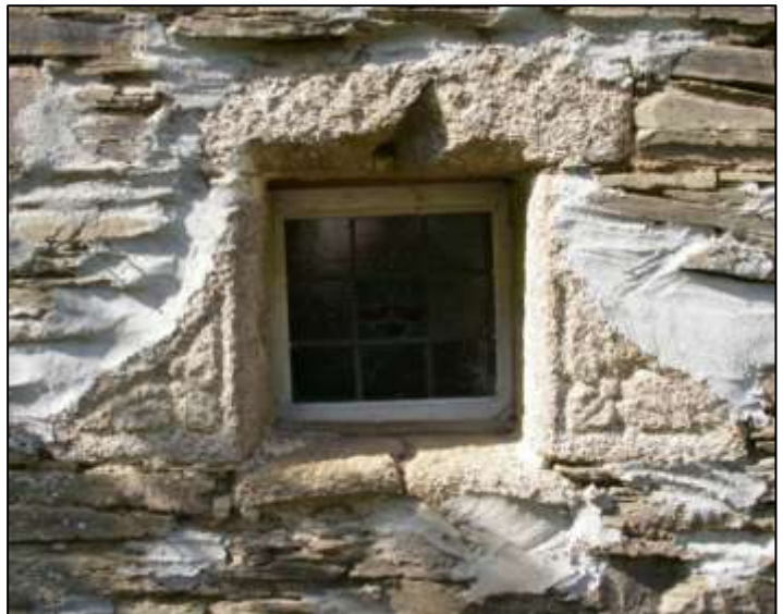
Figure 60: The lower window in the southern elevation, showing the decorative clusped mouldings and floral motif.
