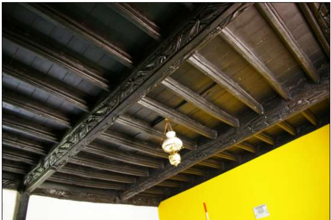
Figure 20: The carved beams in R1; the central beams, viewed from the north-east.
