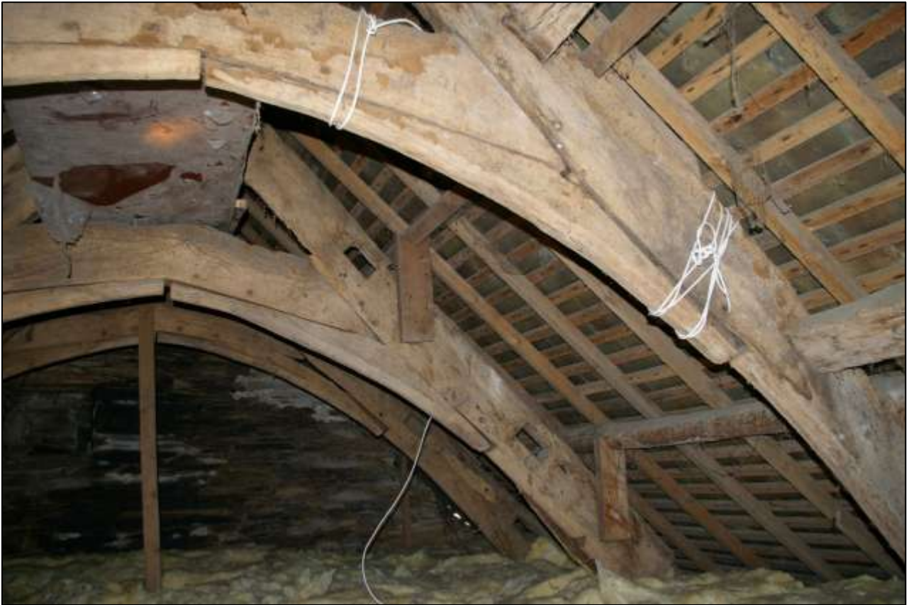
Figure 73: Detail of the roof structure in R 26; viewed from the east, looking west.
