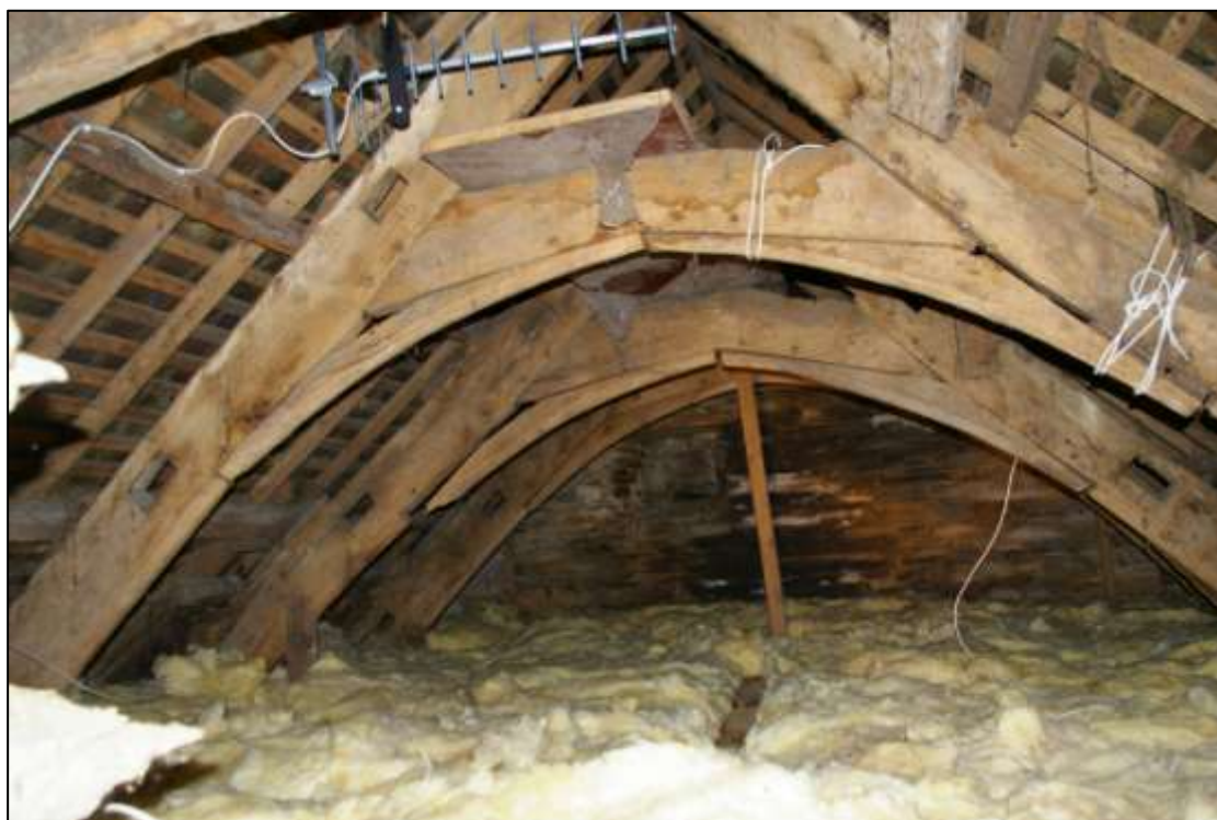
Figure 22: The arch-braced roof in the 15 th century block; viewed from the east, looking west.
