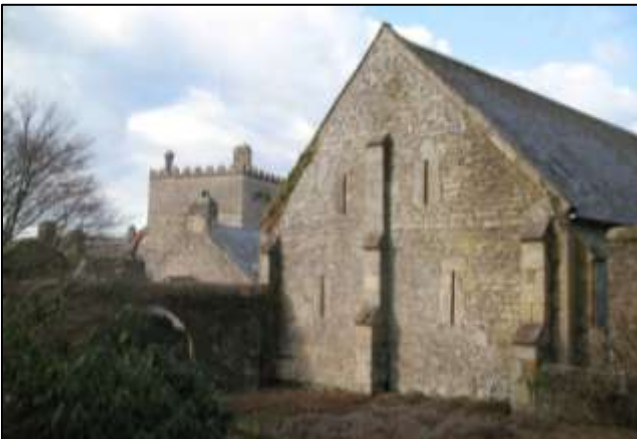
Top: Figure 40: The west elevation of Buckland Abbey barn, viewed from the north-west. Bottom: Figure 42: The south gable of Buckland Abbey barn, viewed from the south.
