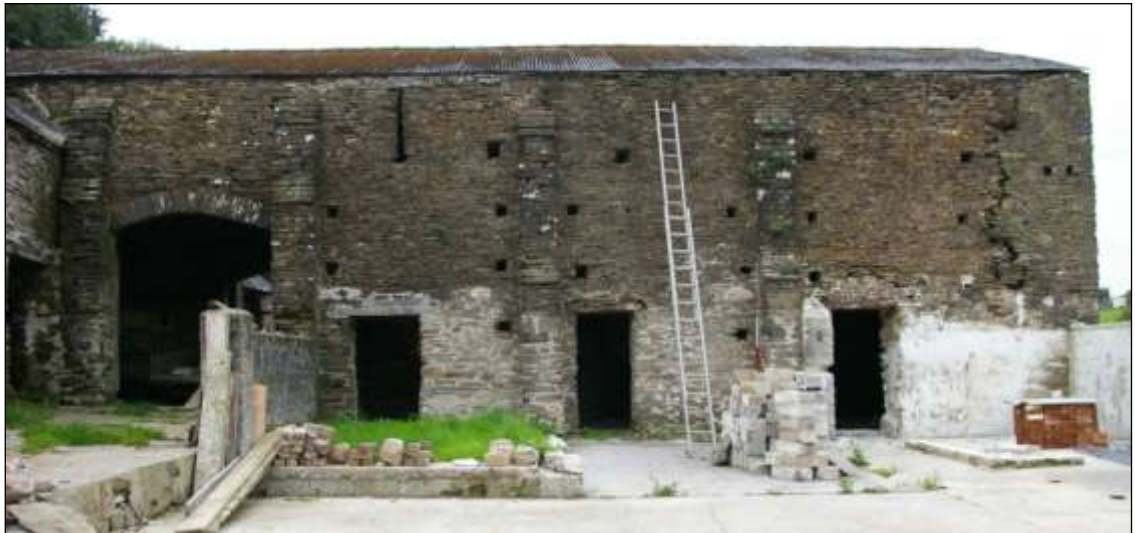
Figure 86: East Elevation of the Great Barn, viewed from the east (scale 2m).
