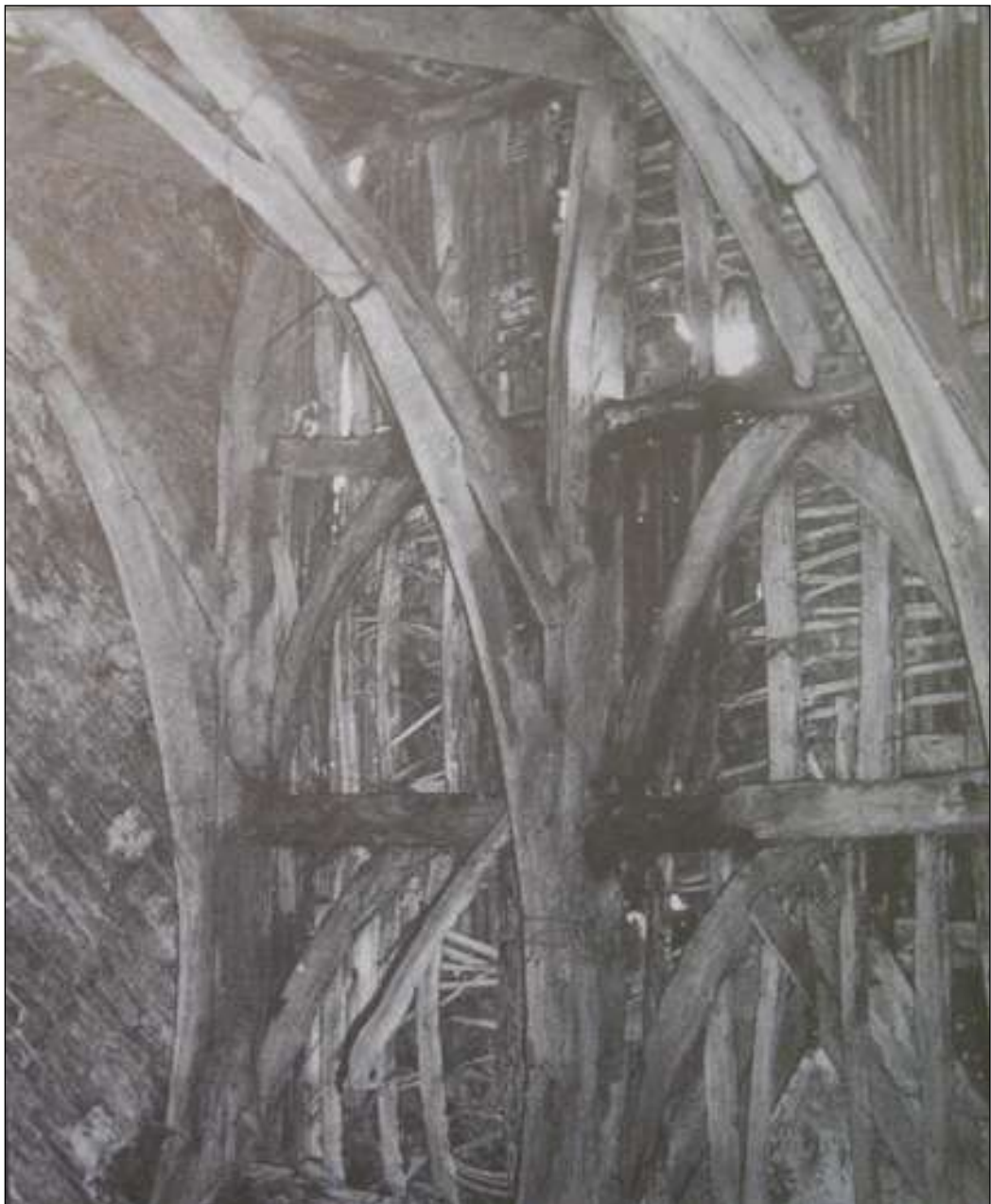
Figure 18: The original roof of the Great Barn, the western truss-blades at the southern end, viewed from below and to the north-east. This photo was published in Langdon (1995), and shows the 15 th century arch-braced roof was in a poor state of repair by the early-mid 20 th century.
