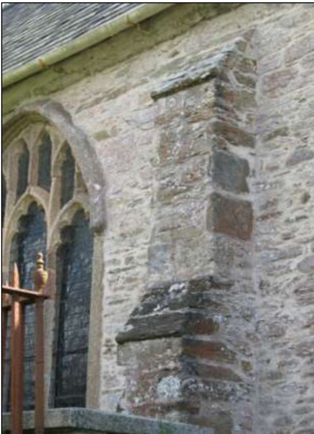
Figure 50: Detail of one of the buttresses on the north aisle. Note also the projecting string course above.
