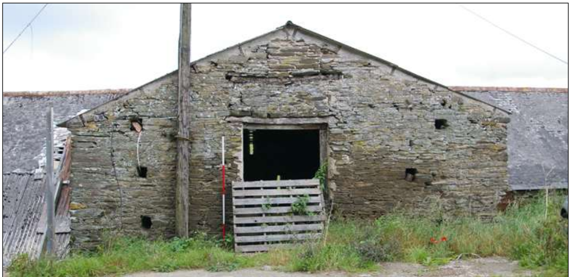
Figure 91: South elevation of the Great Barn, viewed from the south (scale 2m).
