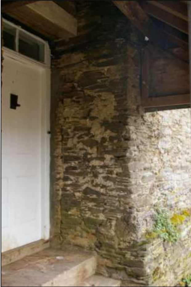
Figure 78: The north-east corner of the northern gable of the 17 th century block, showing the vertical change of build.
