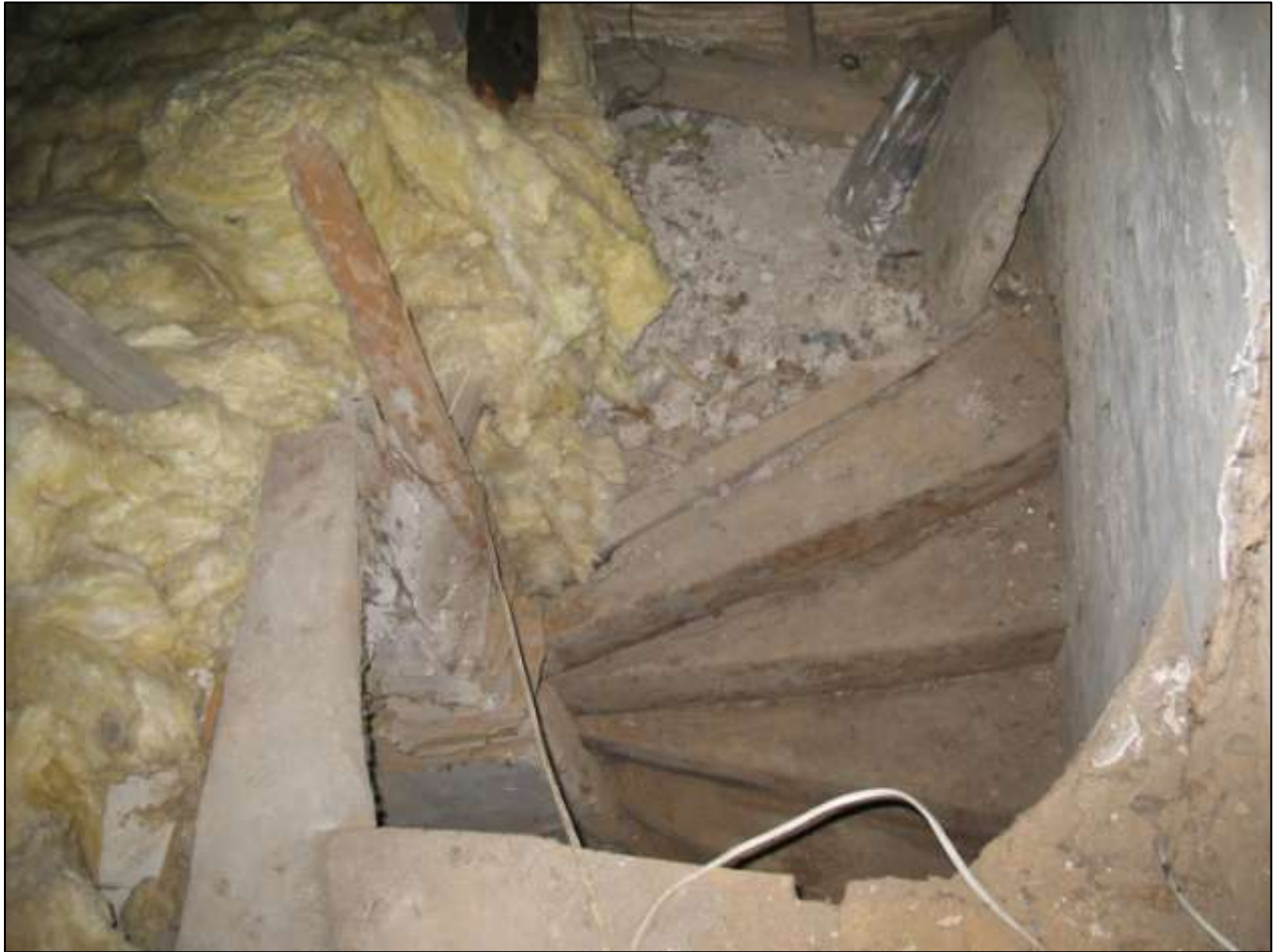
Figure 72: The top of the stairwell; viewed from the west. Note the stairs appear to continue up to the left.
