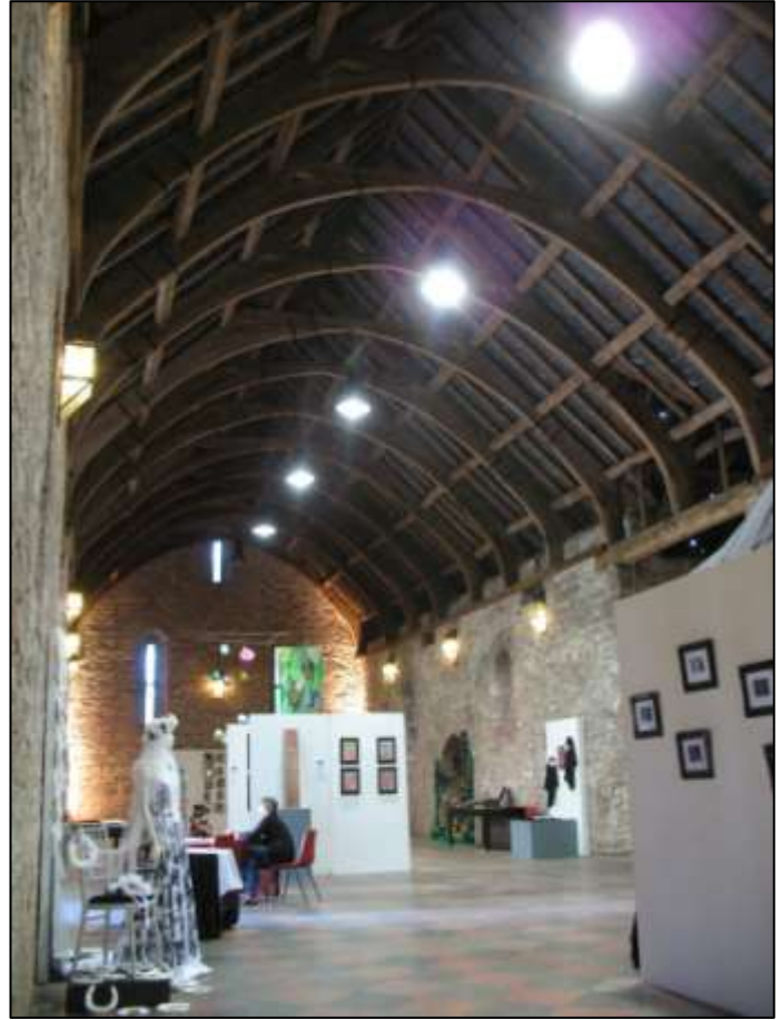
Figure 44: The interior of the barn at Torre Abbey. The barn itself is reputed to date from the late 12 th century, with a (restored) roof structure of the 1450s. Here the arch-braced roof trusses rise from a wall plate set into the upper part of the wall; again, it lacks wind-braces.
