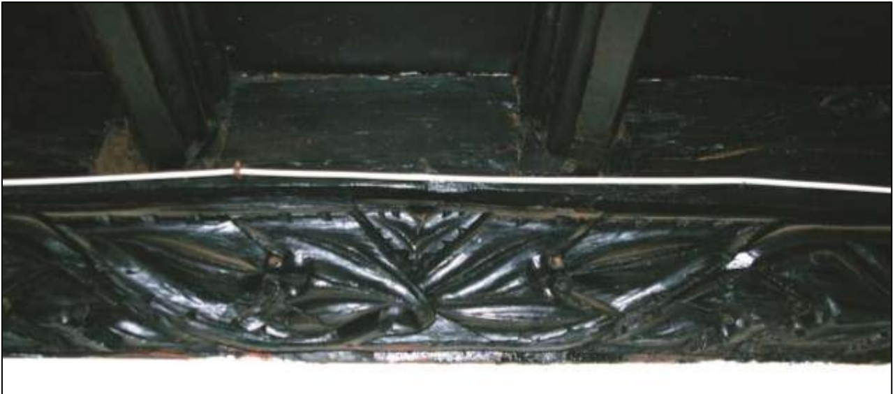
Figure 67: Eastern wallplate, Style 4. Note the holes at the joints of the leaves, and the ill-fitting joists.
