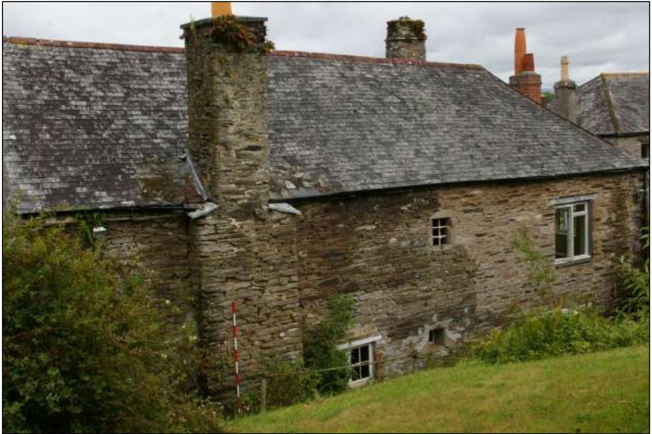
Figure 58: The south-facing elevation of the 15 th century block; viewed from the south-west, looking north-east (scale 2m).
