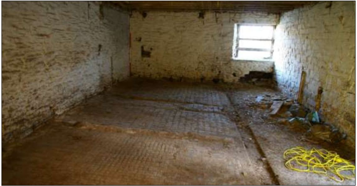
Figure 104: Floor of the stable in the Shippon, viewed from the west. Note the dressed, coursed stonework of the north elevation of the milking parlour (scale 2m).
