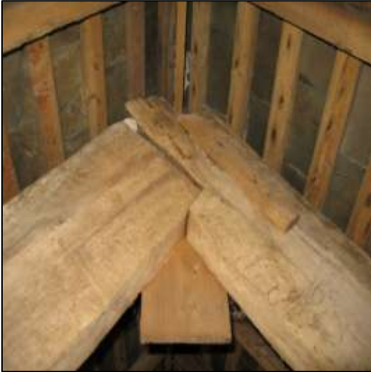
Figure 75: Detail of the joint at the top of the 17 th century trusses.
