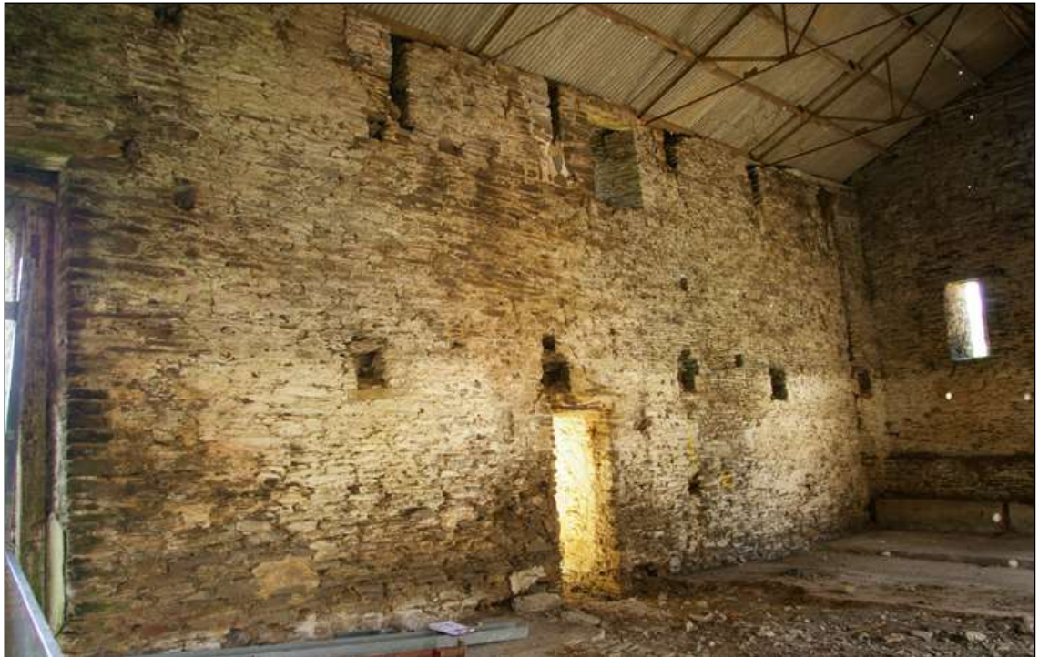
Figure 92: The interior of the Great Barn, the north end of the west wall, viewed from the south-east.
