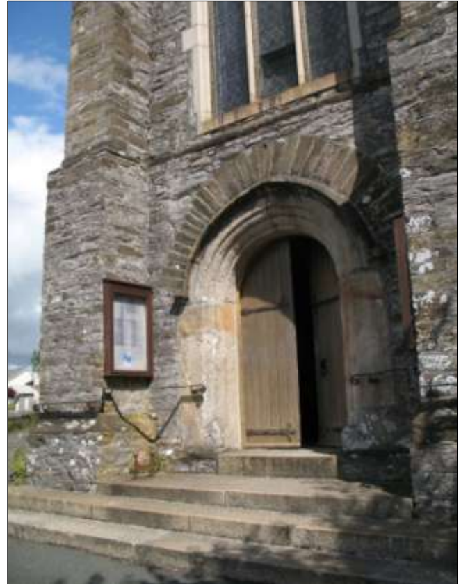
Figure 49: The west face of the tower, viewed from the south-west, looking north-east.
