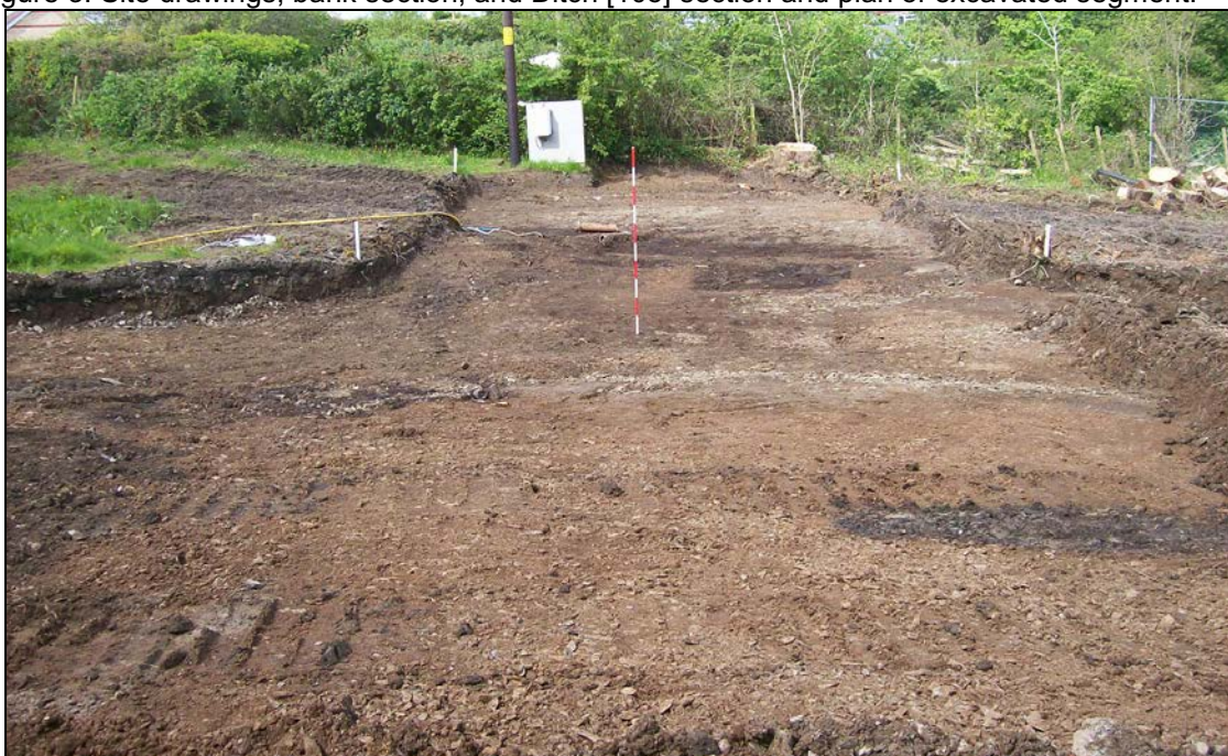
Figure 4: South half of site mid-excavation showing made-ground (103) and services, viewed from the east (2m scale).
