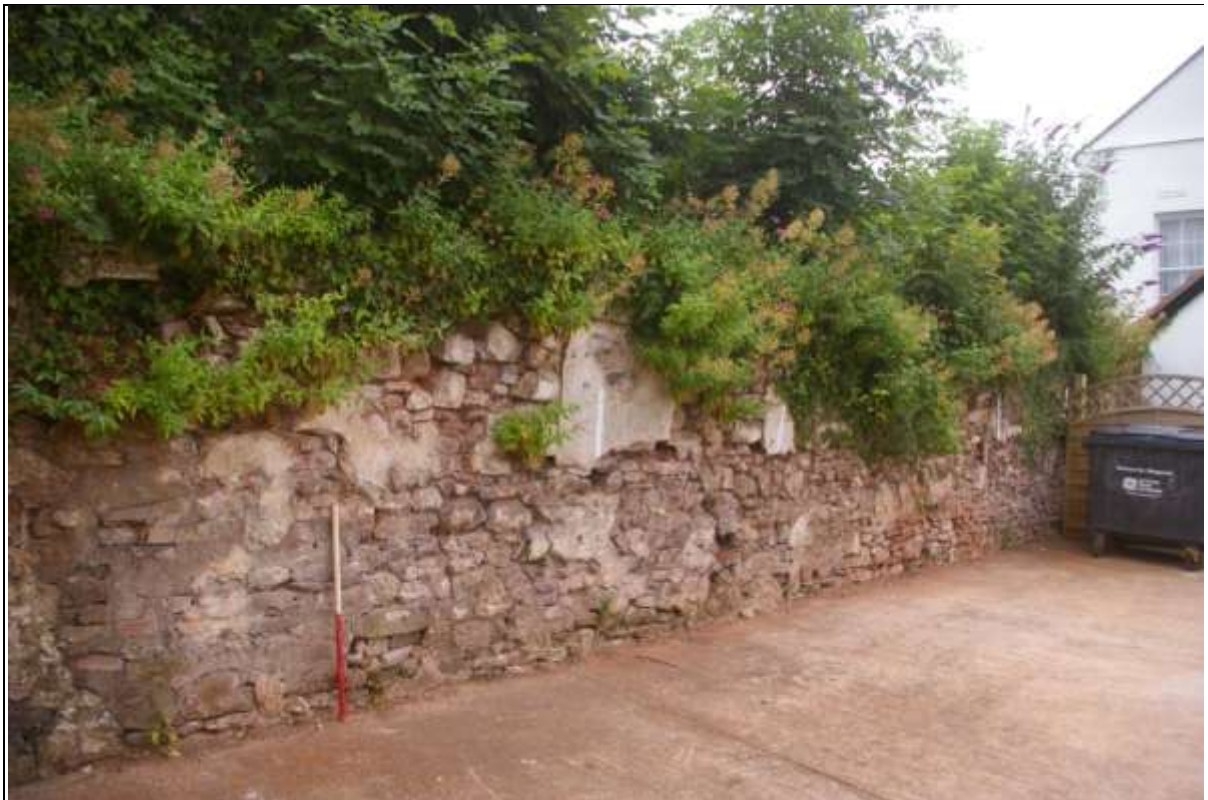
Figure 11: Retaining wall to the yard to the north of the Skittle Alley, viewed from the north (1m scale).
