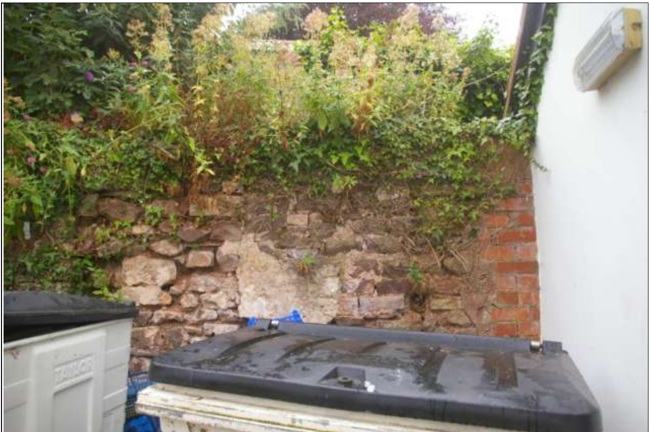
Eastern end of the wall, where it has been abuted/re-built in the 20 th century in brick, at time building to the east was constructed.
