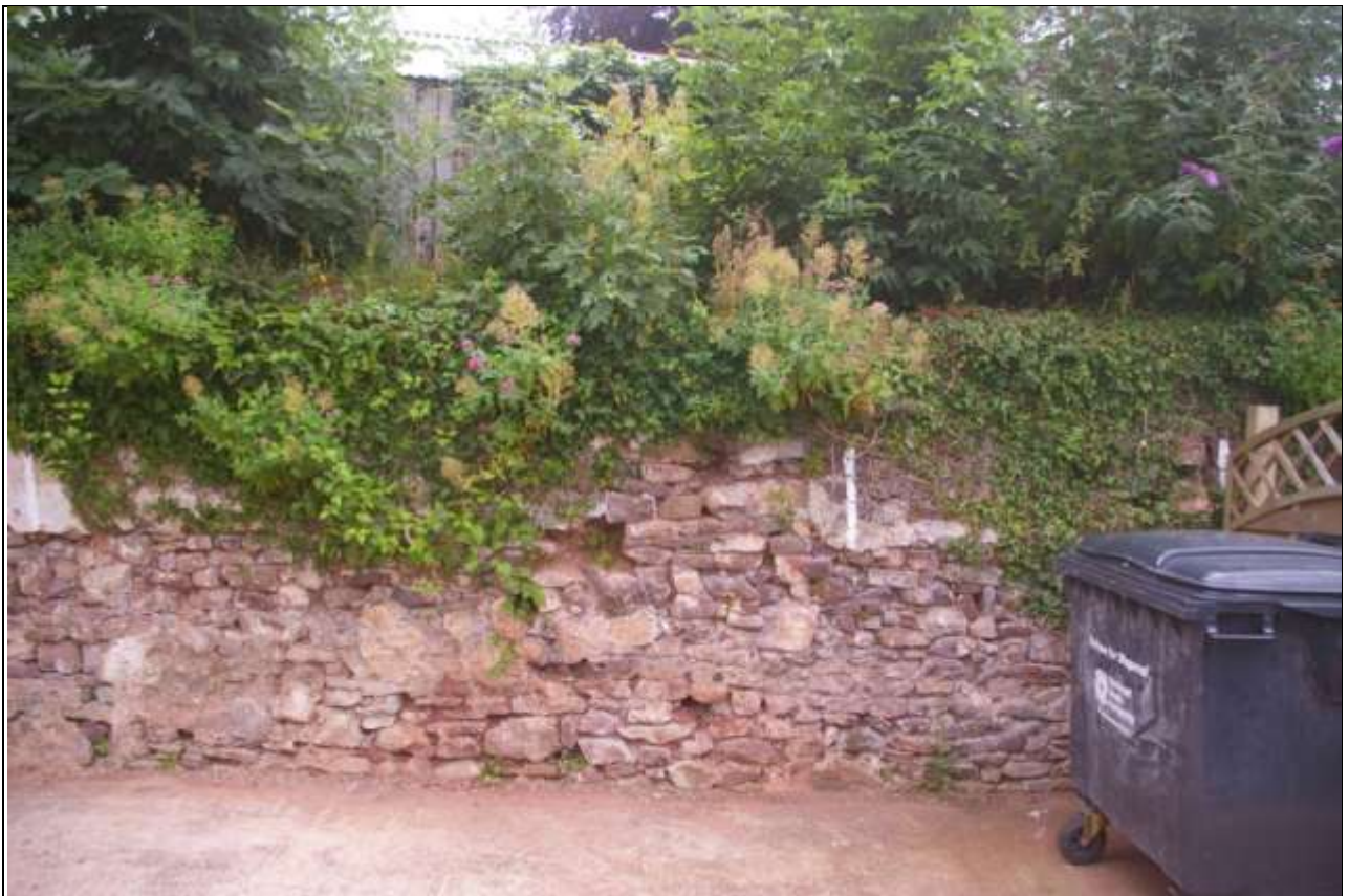
As above, taken slightly to the east, viewed from the north (1m scale).
