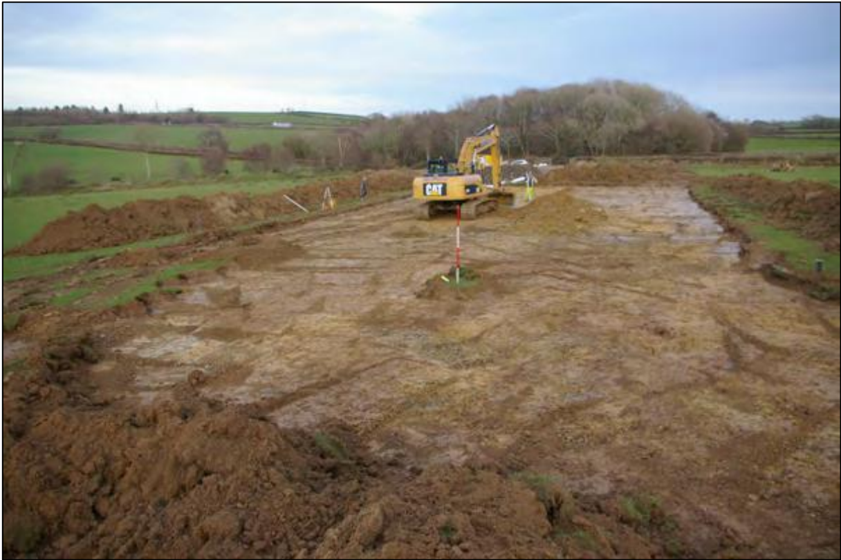
Figure 10: General view of turbine location post excavation, viewed from west (2m scale).
