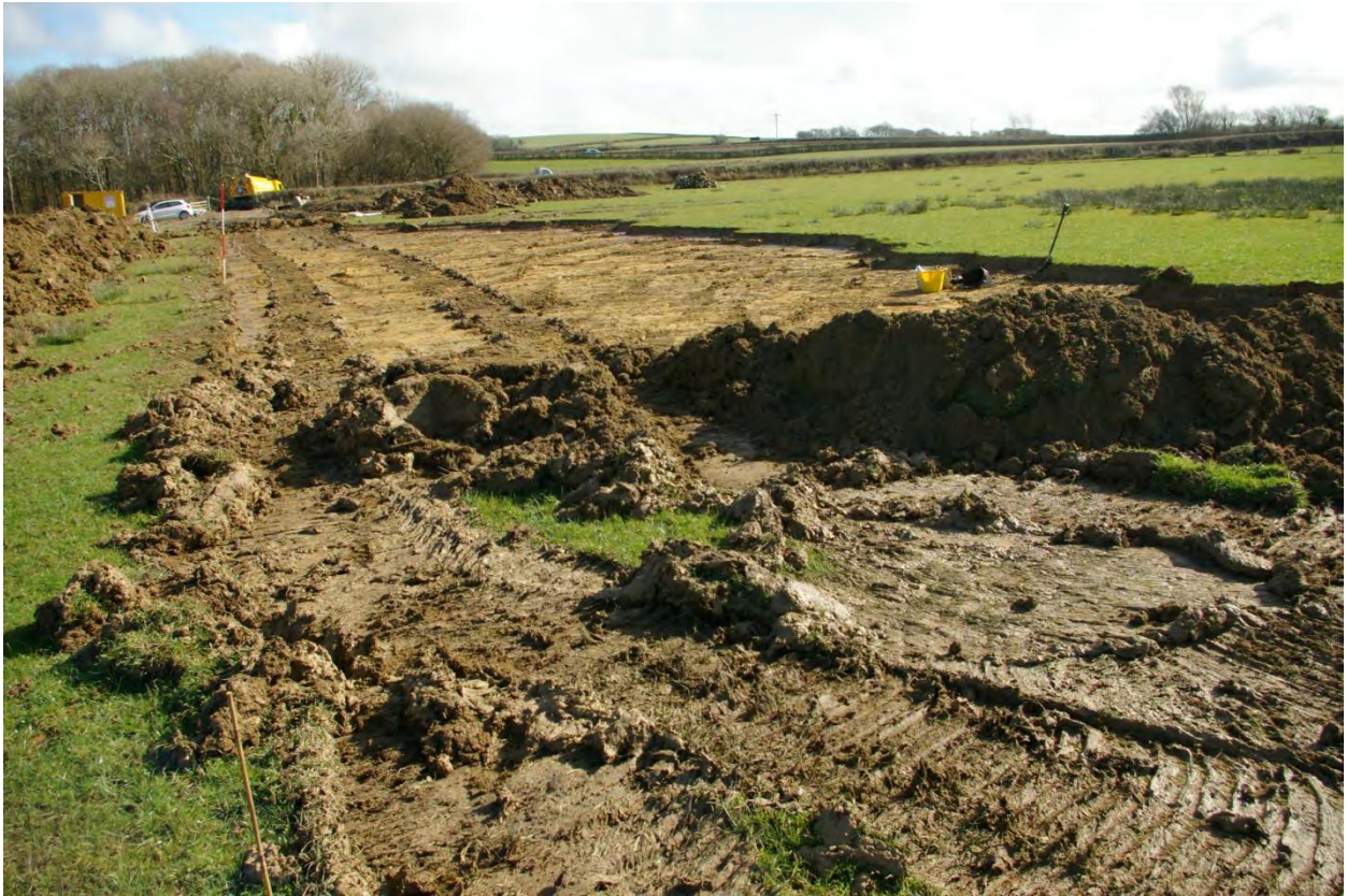
General view of crane base stripped area; from the west, 2m scale.
