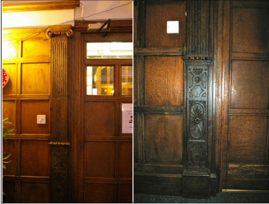
Figure 24: Upper portion of timber pilaster to west of the entrance door in north wall of G17, from the south.
