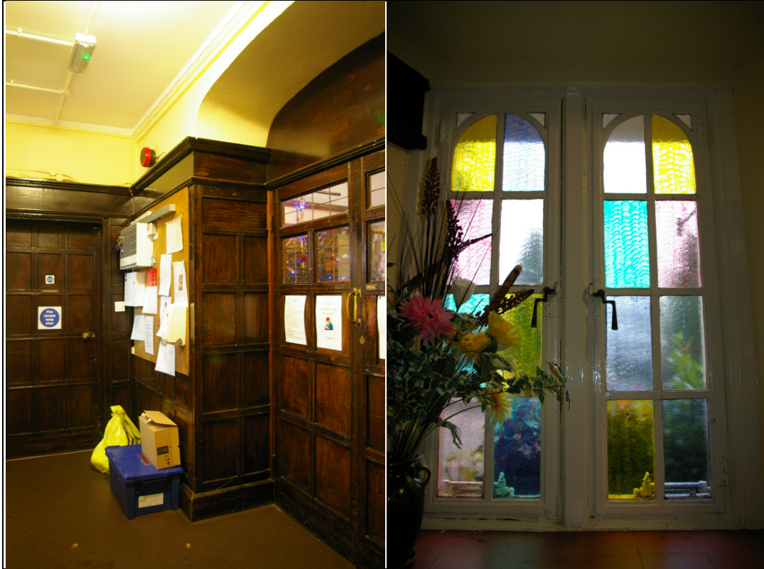
Figure 27: The panelled cupboard, door into lobby G13 and door into G17 from G16, from the south-west. Figure 28: Window to the west of the front door opening in G16, from the south.
