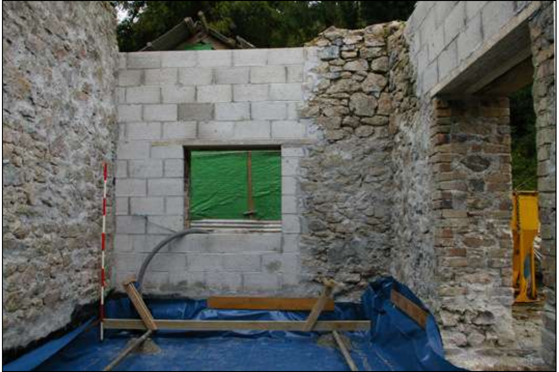
Figure 10: The repaired interior north end of the engine house and northern jamb of the double door opening at the north end of the east elevation; viewed from the south (2m scale).
