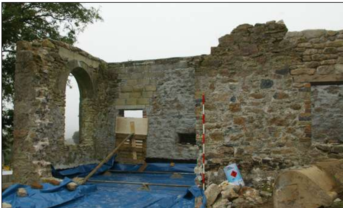
Figure 11: The southern end of the east elevation of the engine house; viewed from the north-east (2m scale).
