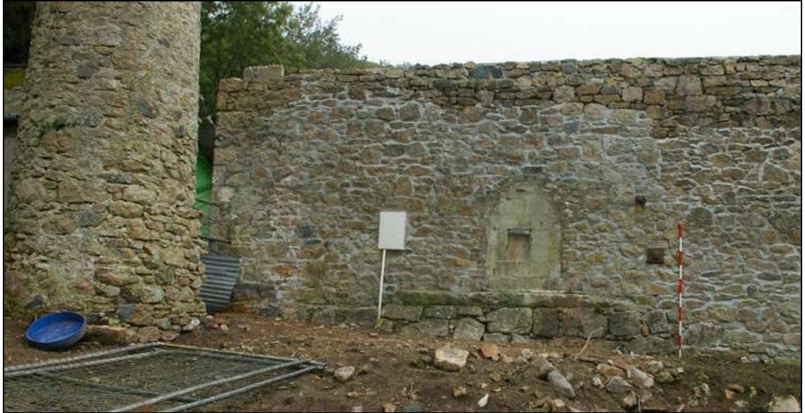
Figure 15: The northern end of the engine house, showing the blocked opening in the west elevation of and truncated masonry at the base of the chimney; viewed from the south-west (2m scale).
