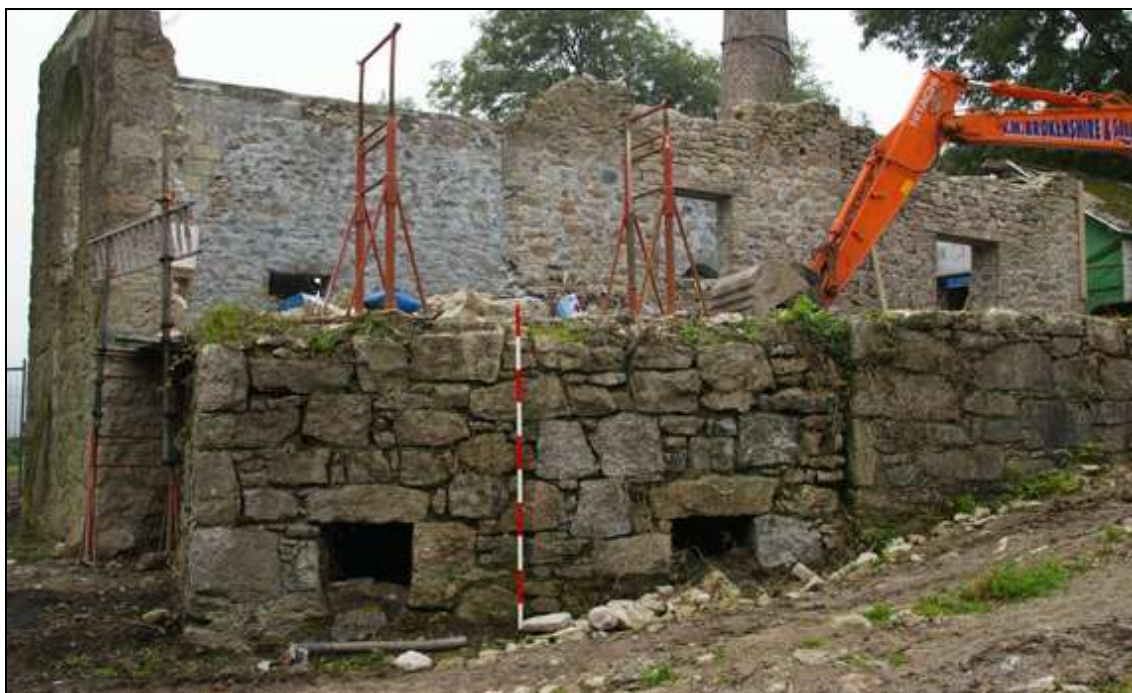
Figure 17: The structures to the south-east of the engine house; viewed from the south-east (2m scale).
