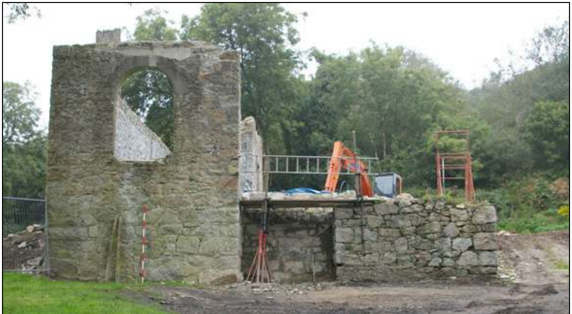
Figure 13: The south elevation of the engine house and associated structures to the east; viewed from the south (2m scale).
