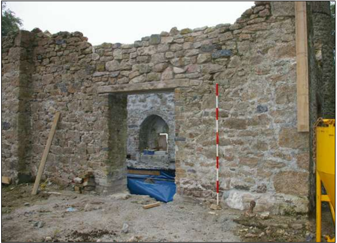
Figure 12: The north end of the east wall of the engine house; viewed from the south-east (2m scale).
