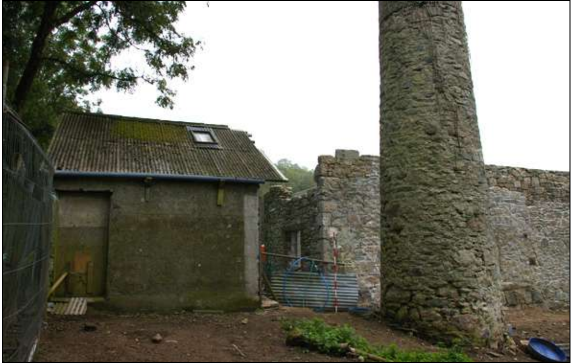
Figure 8: The modern building to the north of the engine house, the north end of the engine house and the base of the chimney, viewed from the north-west (2m scale).
