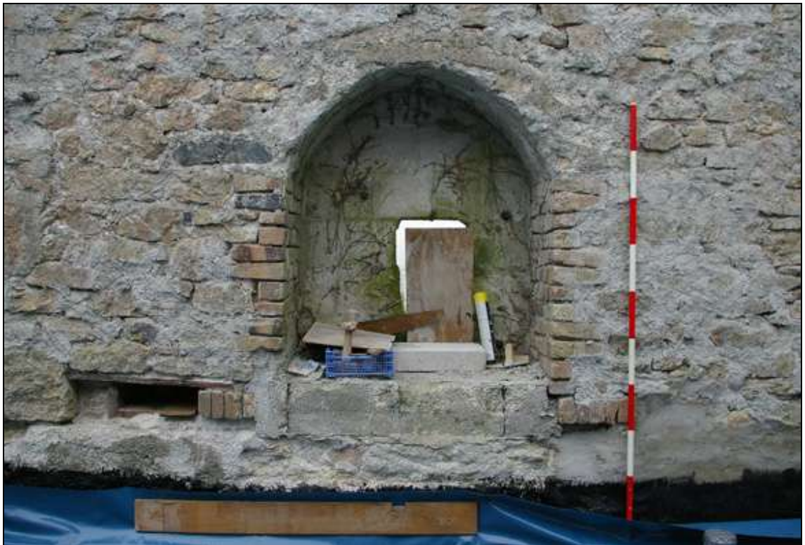
Figure 16: The blocked arched opening in the west wall of the engine house; viewed from the east (2m scale).
