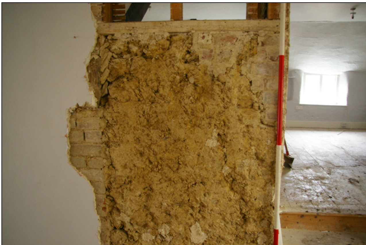
Figure 12: Area of proposed new doorway to Room 5, viewed from north (2m scale).
