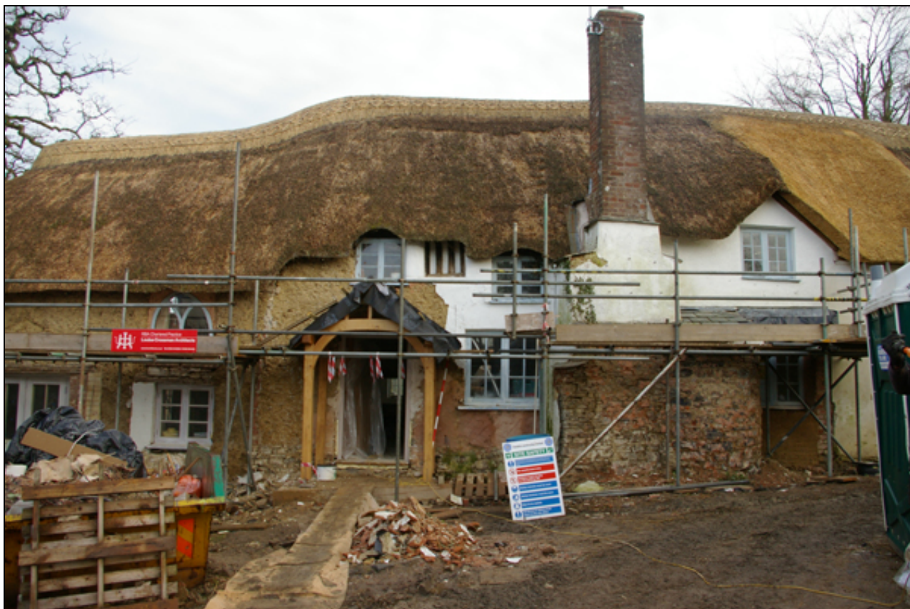
Figure 17: South Elevation of The Longhouse during removal of render, viewed from south (2m scale).
