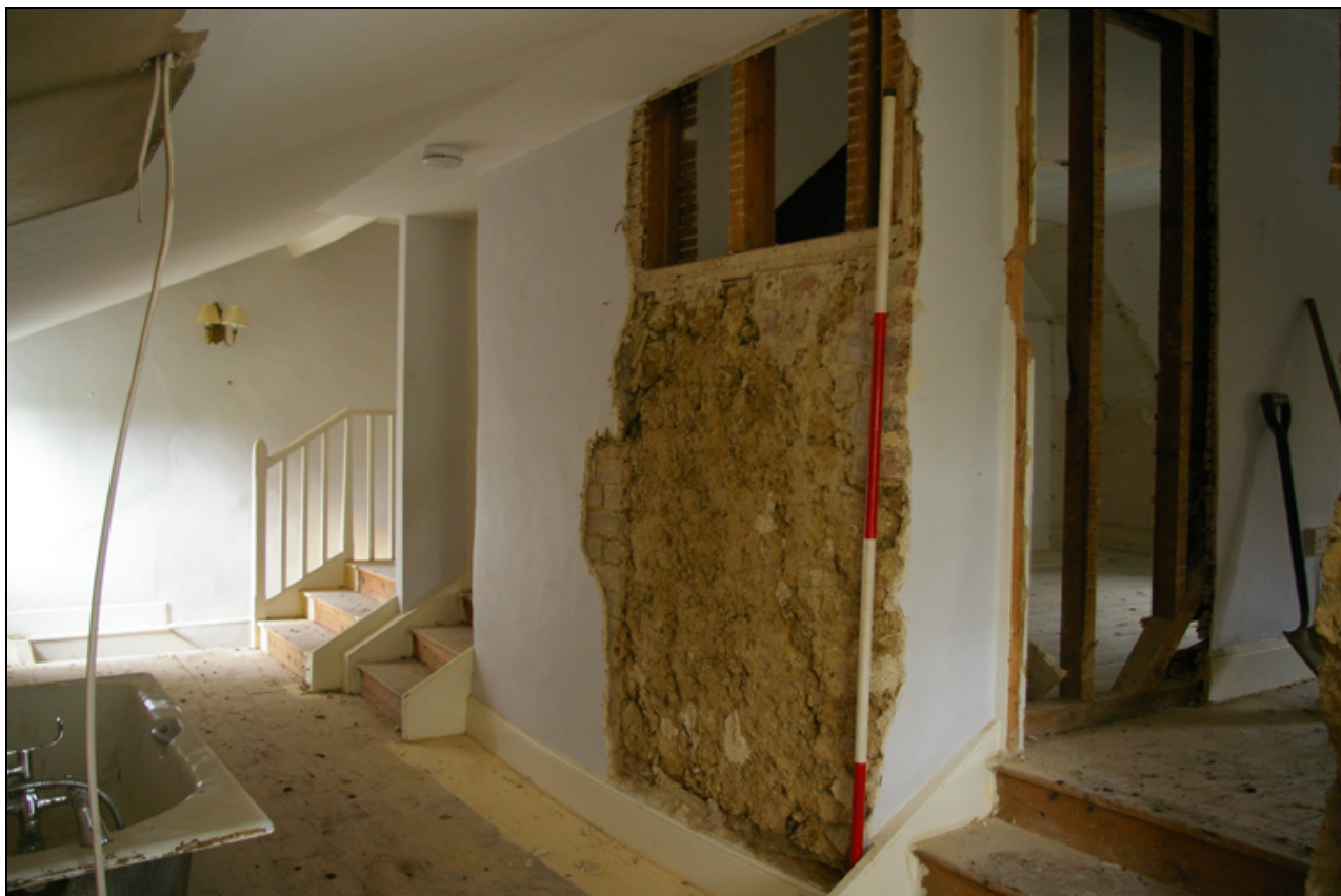
Figure 11: Area of proposed new doorway to Room 5, viewed from north-west (2m scale).
