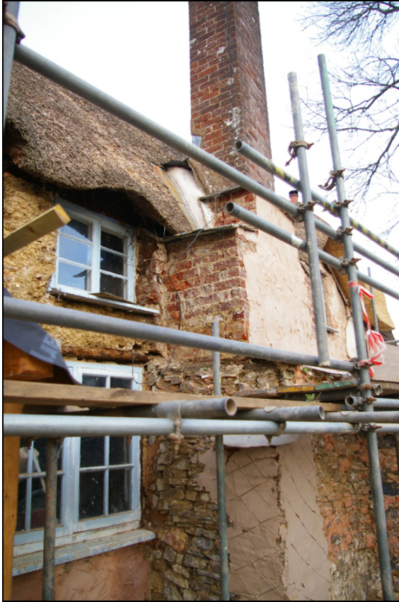
Figure 22: Upper west side of south elevation chimney stack, viewed from south-west (no scale).
