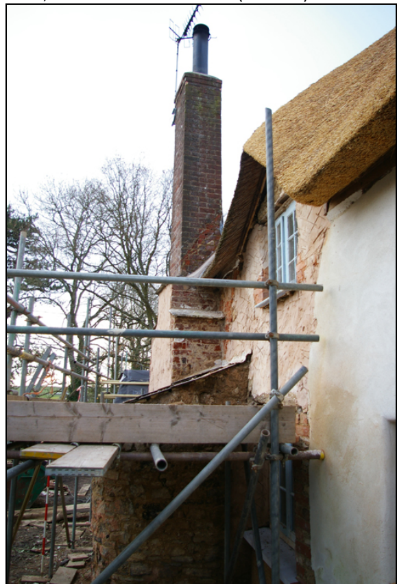
Figure 25: east side of chimney stack and oven, viewed from east (2m scale).
