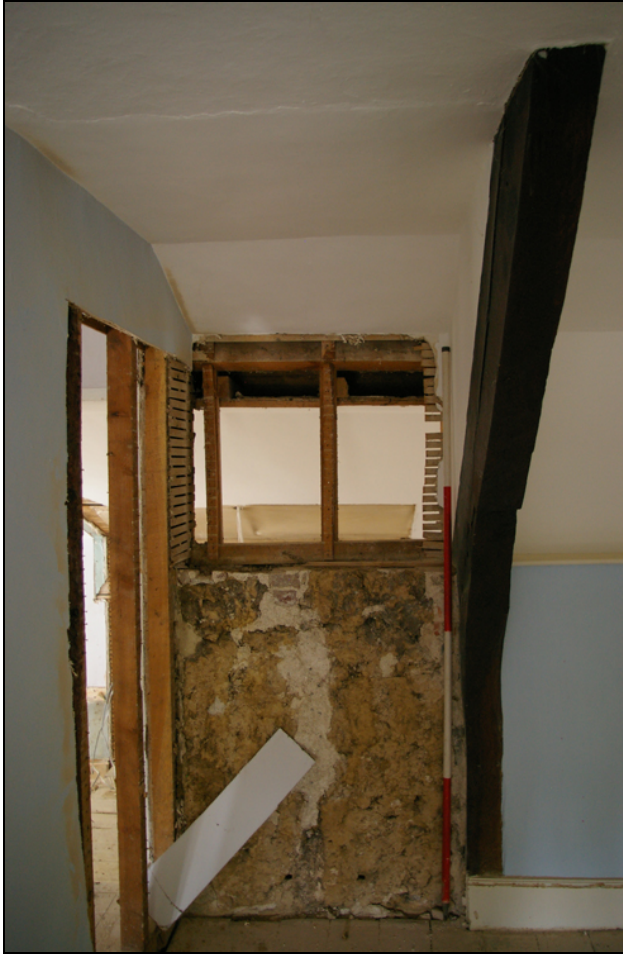
Figure 13: Room 5, wall partition, door to be inserted, roof truss, viewed from south (2m scale).
