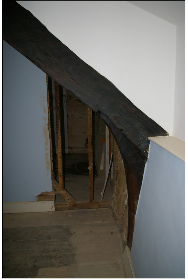
Figure 14: Room 5, wall partition to be removed and roof truss, viewed from east (no scale).
