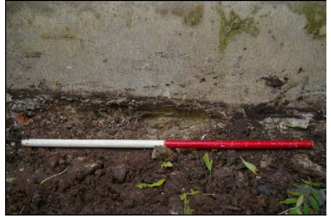
Figure 16: Test Pit 8, establishing depth of south elevation foundations, viewed from south (1m scale).
