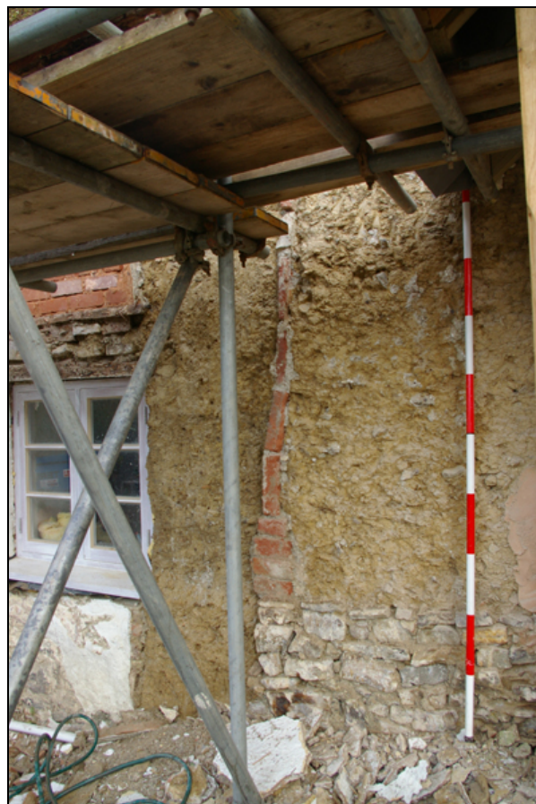
Figure 21: Exposed joint of west and main elements of the house, viewed from south (2m scale).
