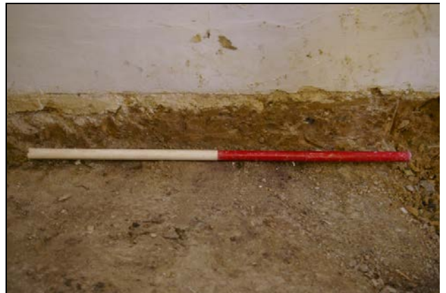
Figure 9: Room 4 entrance hall wall foundation and natural clay, viewed from south (1m scale).
