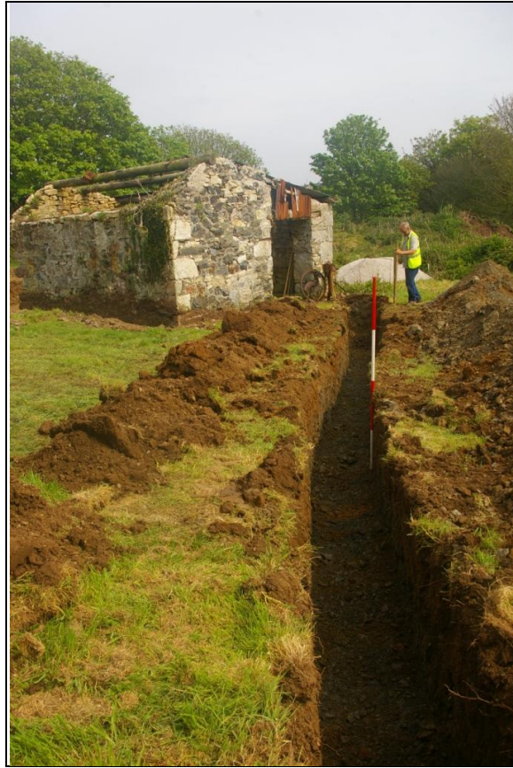
THE SERVICES TRENCH, FROM THE NORTHERN BOUNDARY TO THE BUILDING TRENCH; VIEWED FROM THE NORTH-WEST (2M SCALE).
