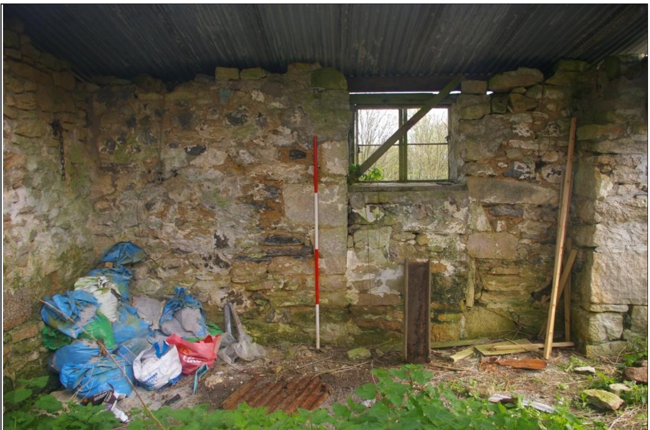
THE INTERIOR FACE OF THE SOUTH ELEVATION, SHOWING THE BLOCKED DOORWAY; VIEWED FROM THE NORTH (2M SCALE).
