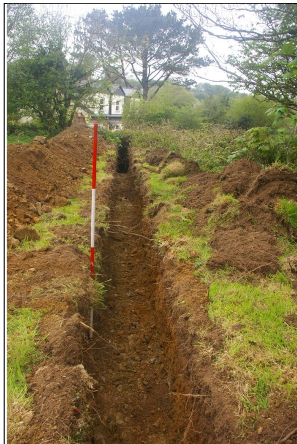
THE WESTERN RUN OF THE SERVICES TRENCH, LEADING TO THE WESTERN BOUNDARY; VIEWED FROM THE NORTH-EAST (2M SCALE).
