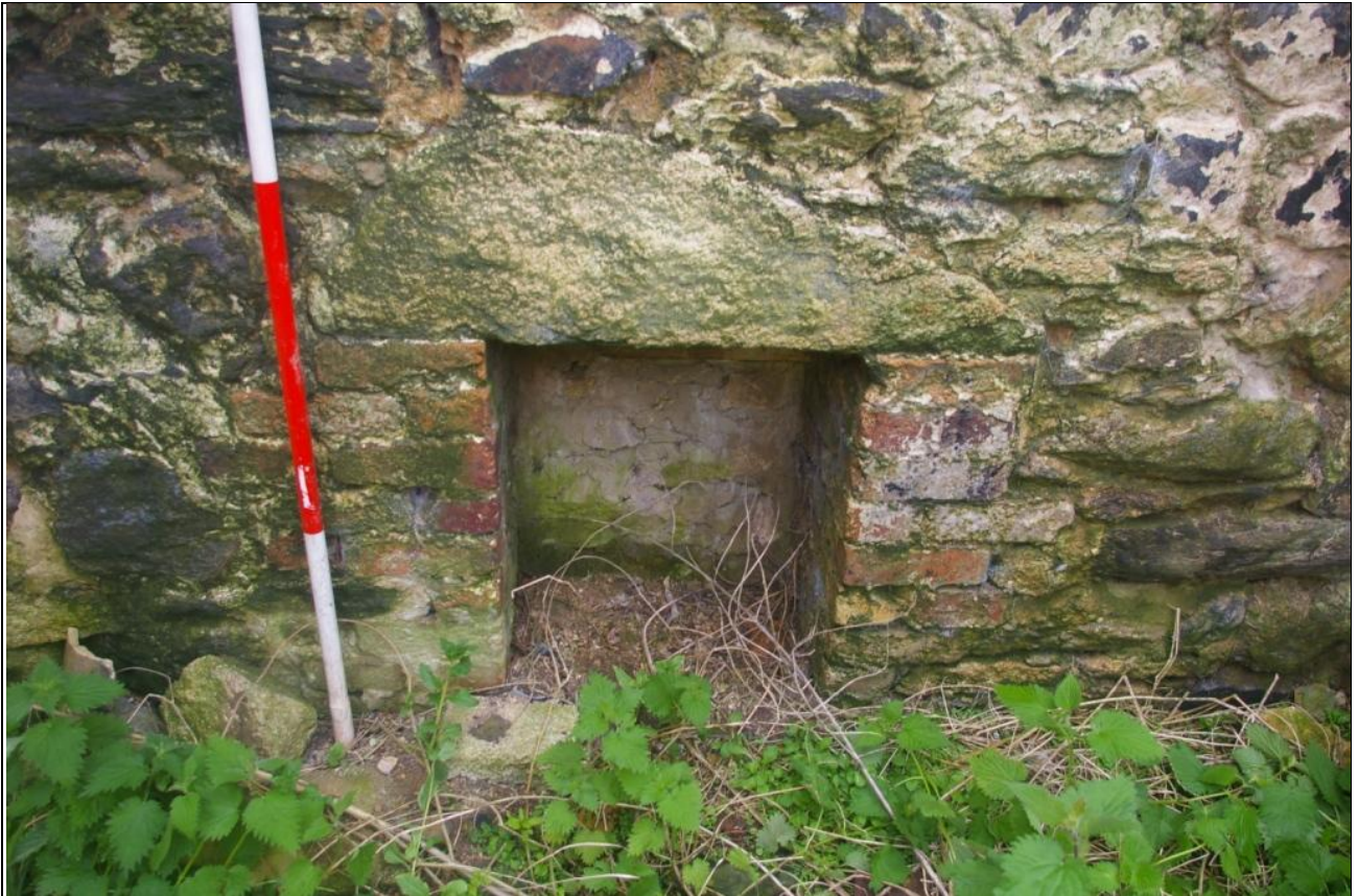
THE FIREPLACE INSERTED INTO THE WEST ELEVATION, WITH CEMENT BONDED BRICKS; VIEWED FROM THE EAST (2M SCALE).
