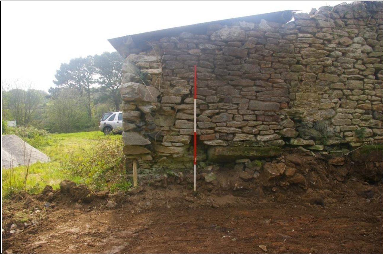
THE RAGGED EASTERN END OF THE SOUTH WALL AND THE INFILLED EAST WALL; VIEWED FROM THE EAST (2M SCALE).
