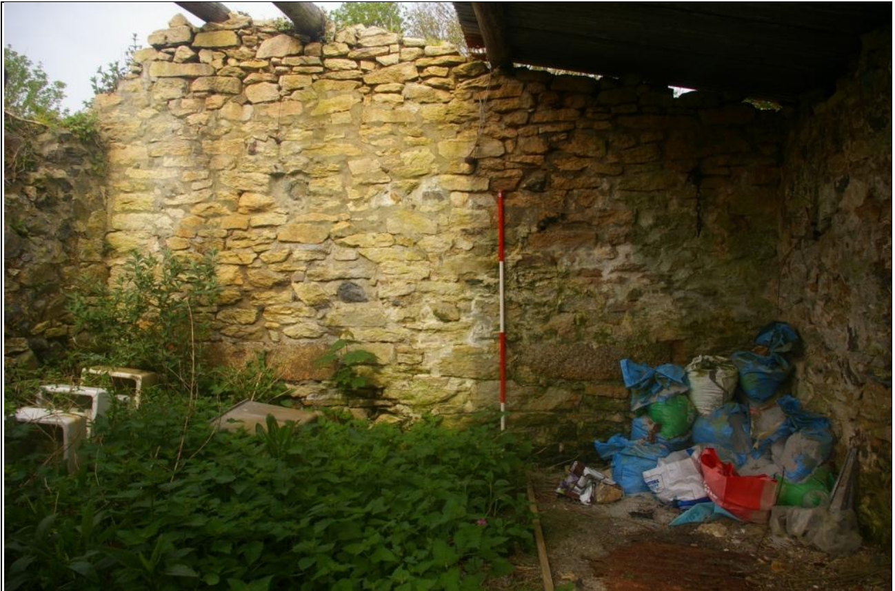
THE INTERIOR FACE OF THE EAST ELEVATION; VIEWED FROM THE WEST (2M SCALE).
