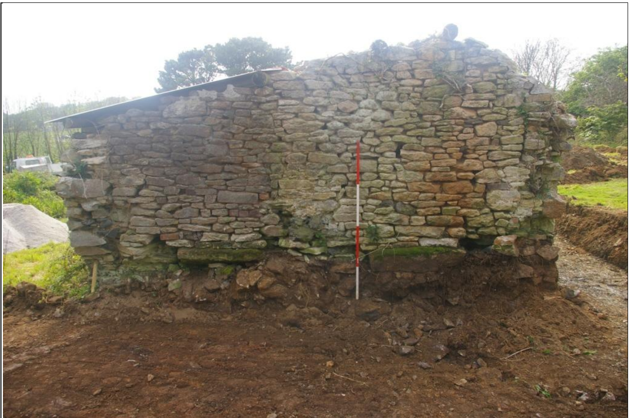
THE EAST ELEVATION OF THE BUILDING; VIEWED FROM THE EAST (2M SCALE).
