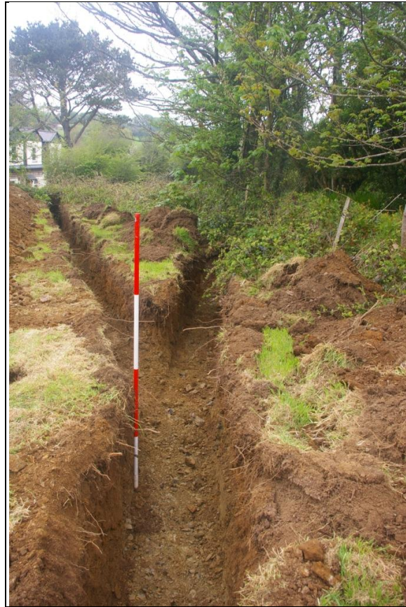
THE SERVICES TRENCH, WHERE IT FORKS, ONE SHORT RUN, LEADING TO THE NORTHERN HEDGEBANK FOR THE ELECTRICS, THE OTHER RUNNING WEST TO THE WESTERN BOUNDARY; VIEWED FROM THE EAST (2M SCALE).
