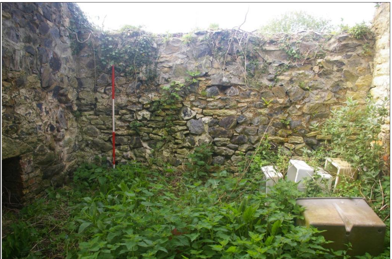
THE INTERIOR FACE OF THE NORTH ELEVATION; VIEWED FROM THE SOUTH (2M SCALE).
