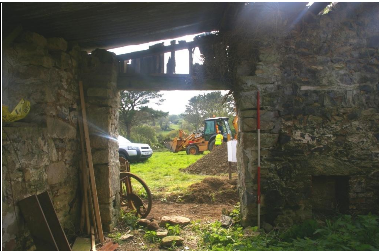
THE DOORWAY IN THE WEST ELEVATION; VIEWED FROM THE EAST (2M SCALE).
