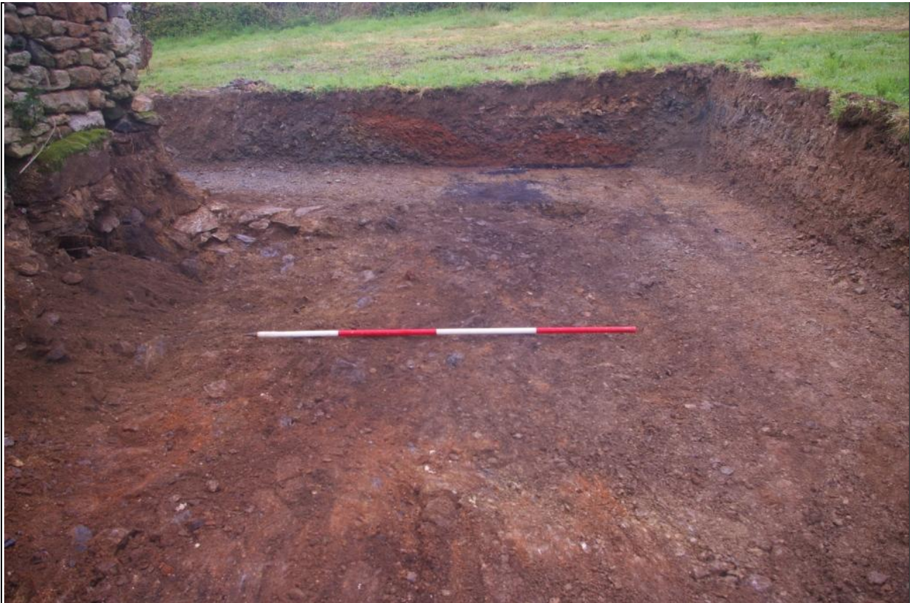
THE LOOSE RUBBLE WHICH BACK-FILLS THE DEMOLISHED EASTERN END OF THE BUILDING; VIEWED FROM THE SOUTH (2M SCALE).
