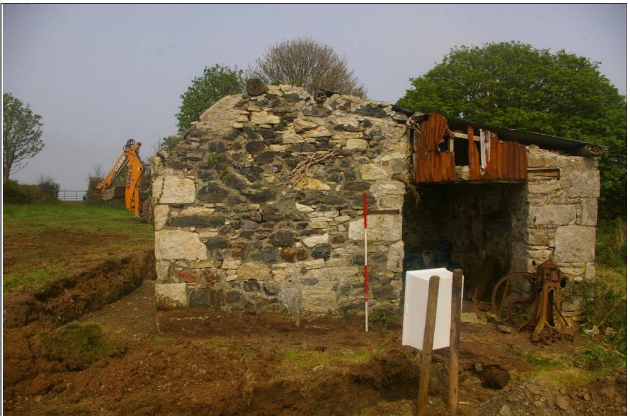
THE WEST ELEVATION OF THE BUILDING; VIEWED FROM THE WEST (2M SCALE).
