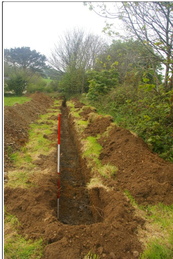
THE SERVICES TRENCH, WHICH FOLLOWS ALONG THE NORTHERN BOUNDARY OF THE FIELD; VIEWED FROM THE EAST (2M SCALE).
