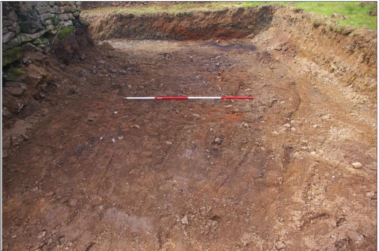
THE STRIPPED AREA TO THE EAST OF THE BUILDING; VIEWED FROM THE SOUTH (2M SCALE).
