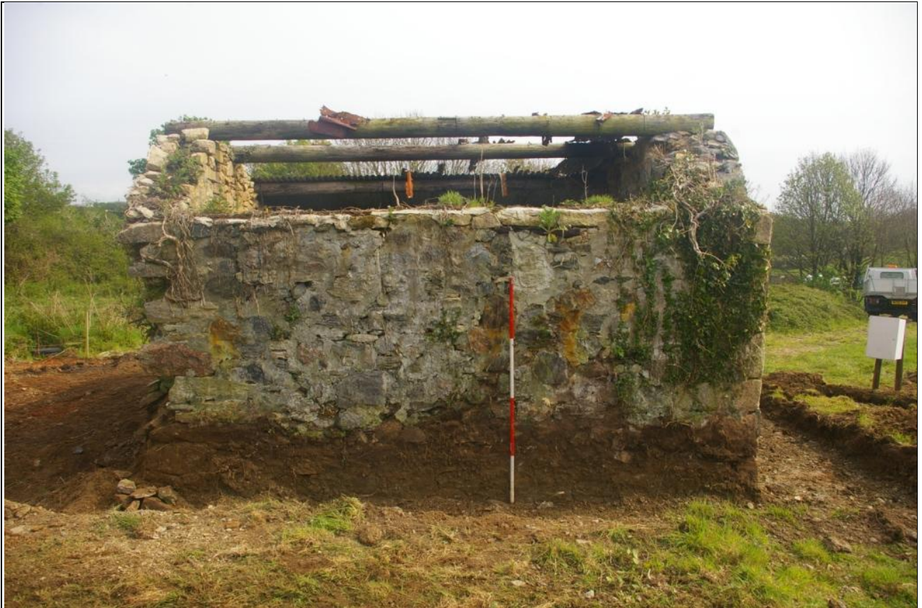
THE NORTH ELEVATION OF THE BUILDING; VIEWED FROM THE NORTH (2M SCALE).
