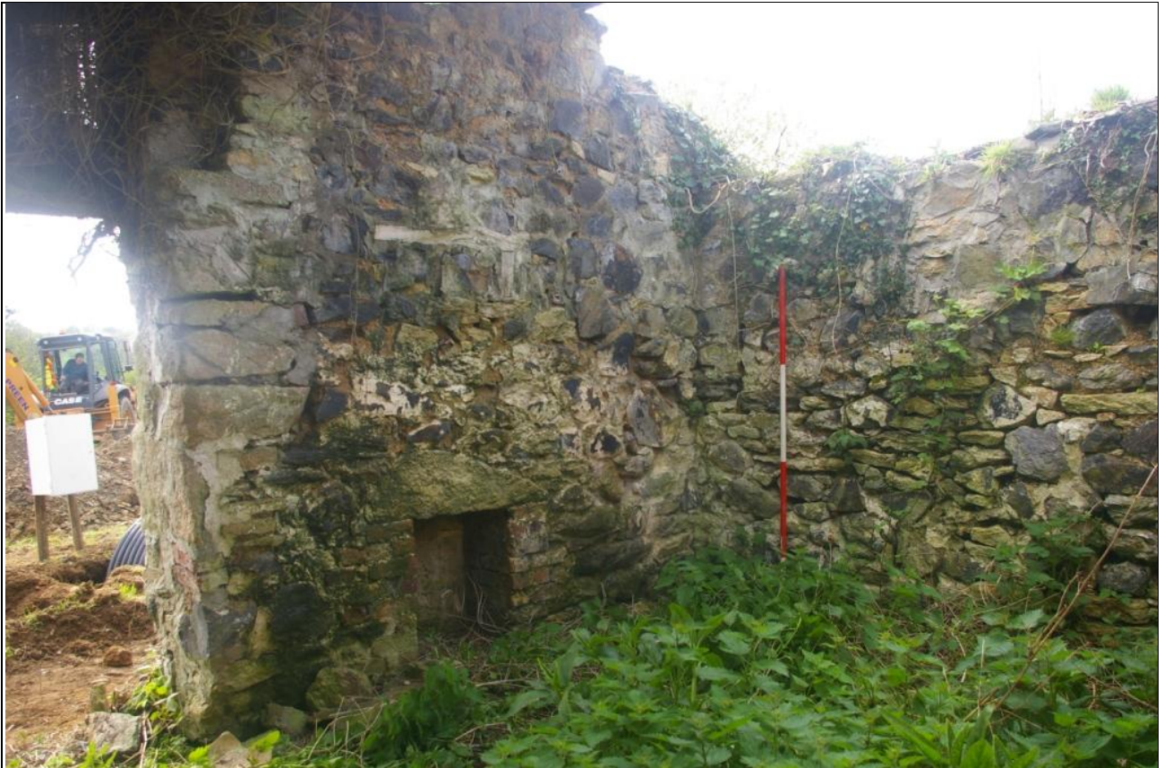
THE INTERIOR FACE OF THE NORTH-WEST CORNER; VIEWED FROM THE SOUTH-EAST (2M SCALE).
