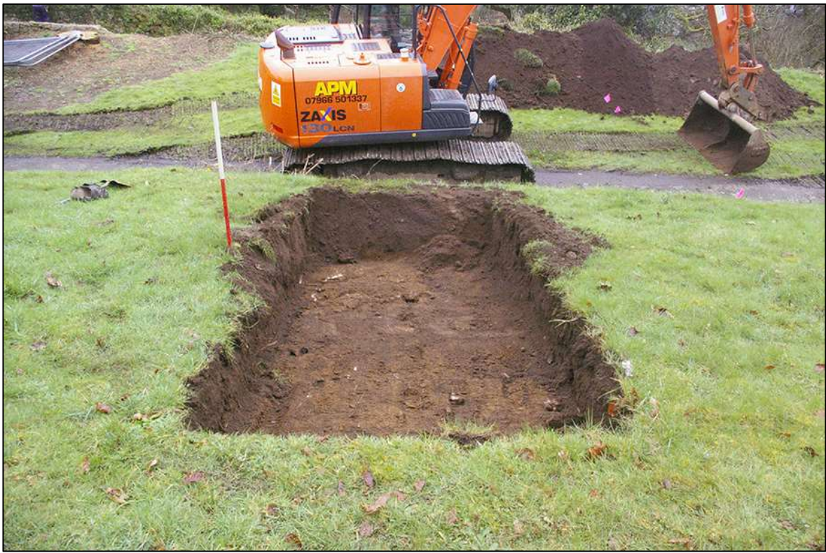
FIGURE 2: TRENCH ACROSS PROPOSED BUILDING PLOT, POST-EXCAVATION; VIEWED FROM THE WEST (1M SCALE).
