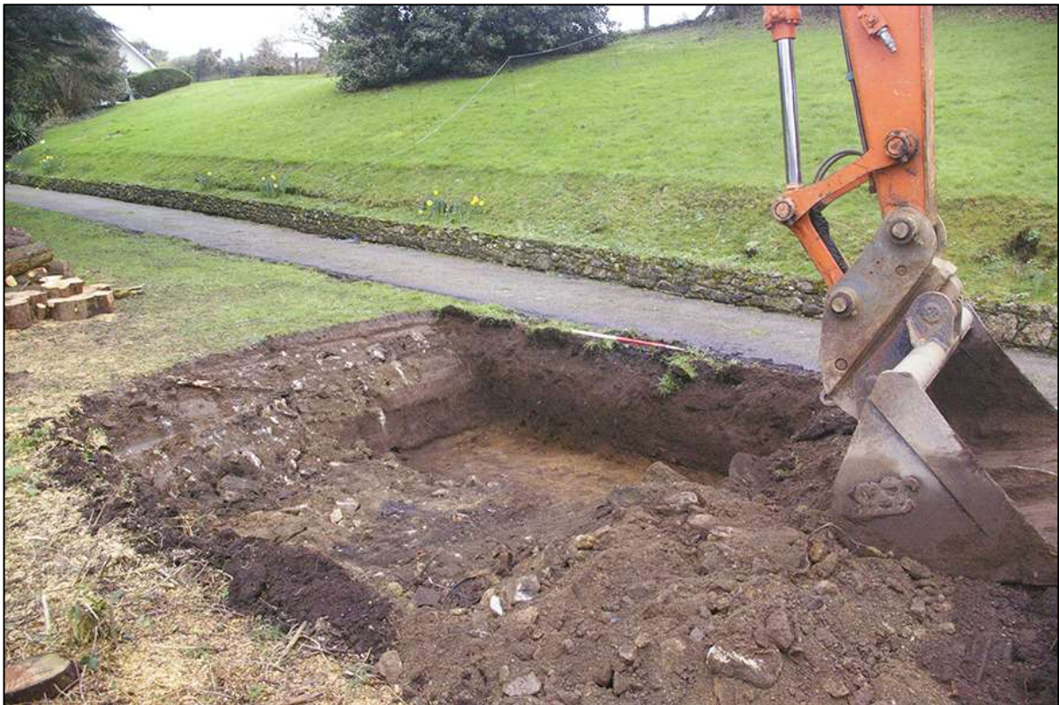
FIGURE 3: AREA OF PROPOSED NEW ACCESS TRACK, MID-EXCAVATION; VIEWED FROM THE NORTH-EAST (1M SCALE).
