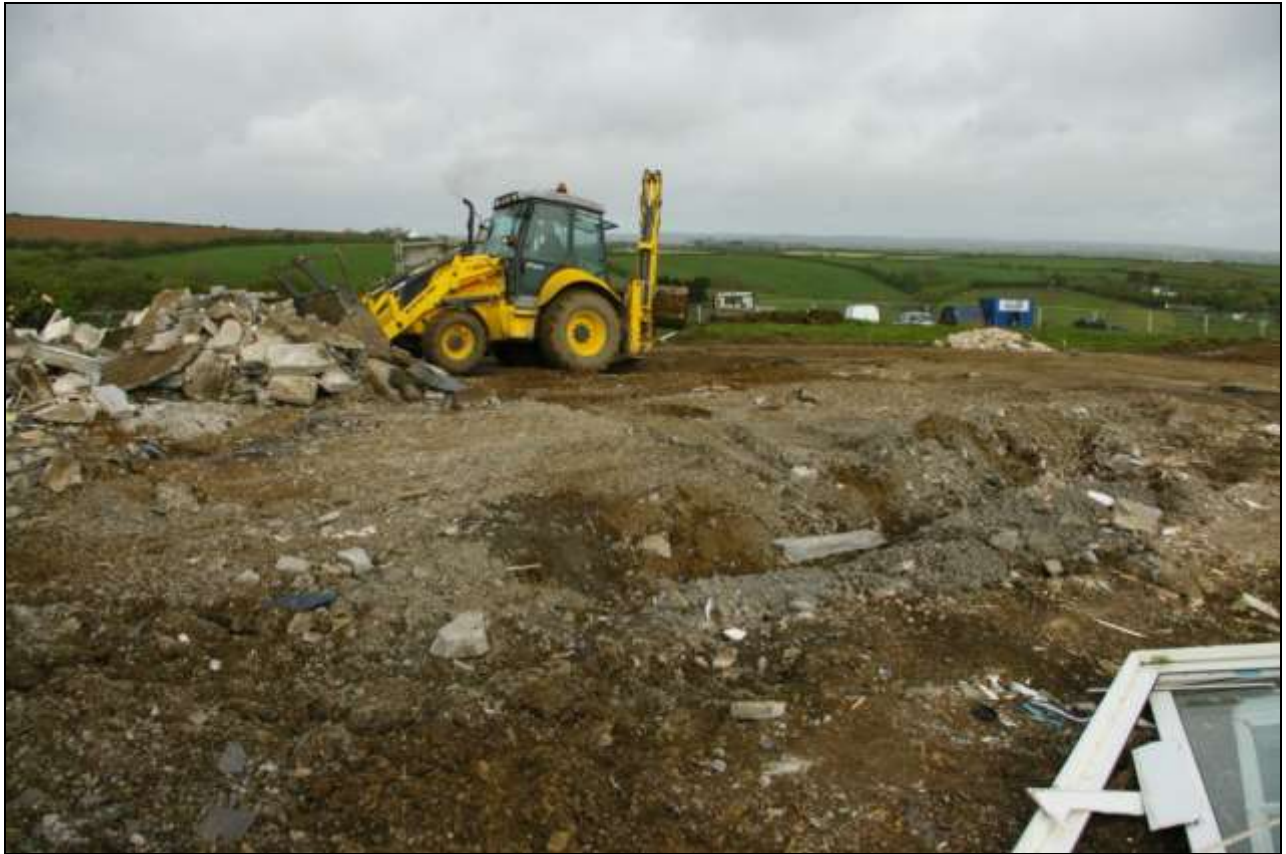
Shot showing the area of the demolished bungalow, viewed from the south.
