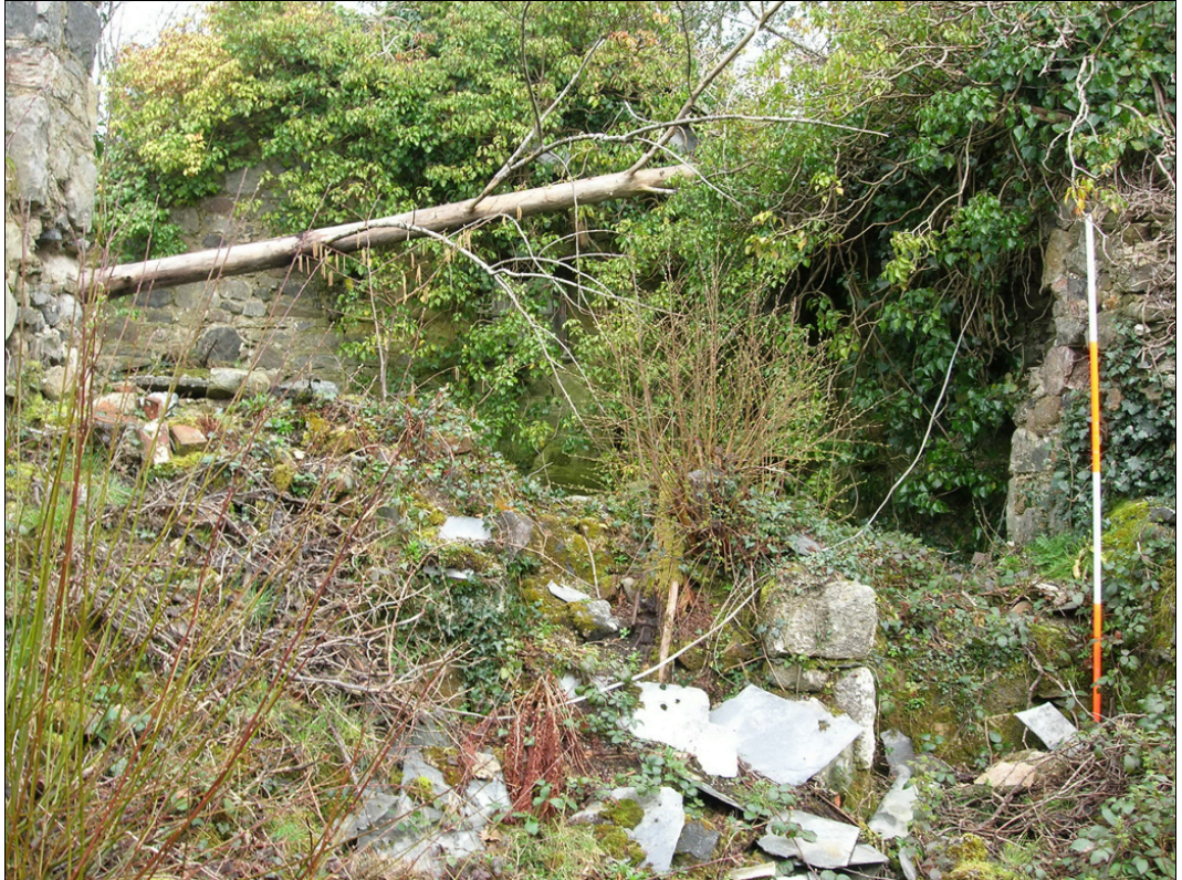
The collapsed wall between the Mill and the Cottage, viewed from the south-east.
