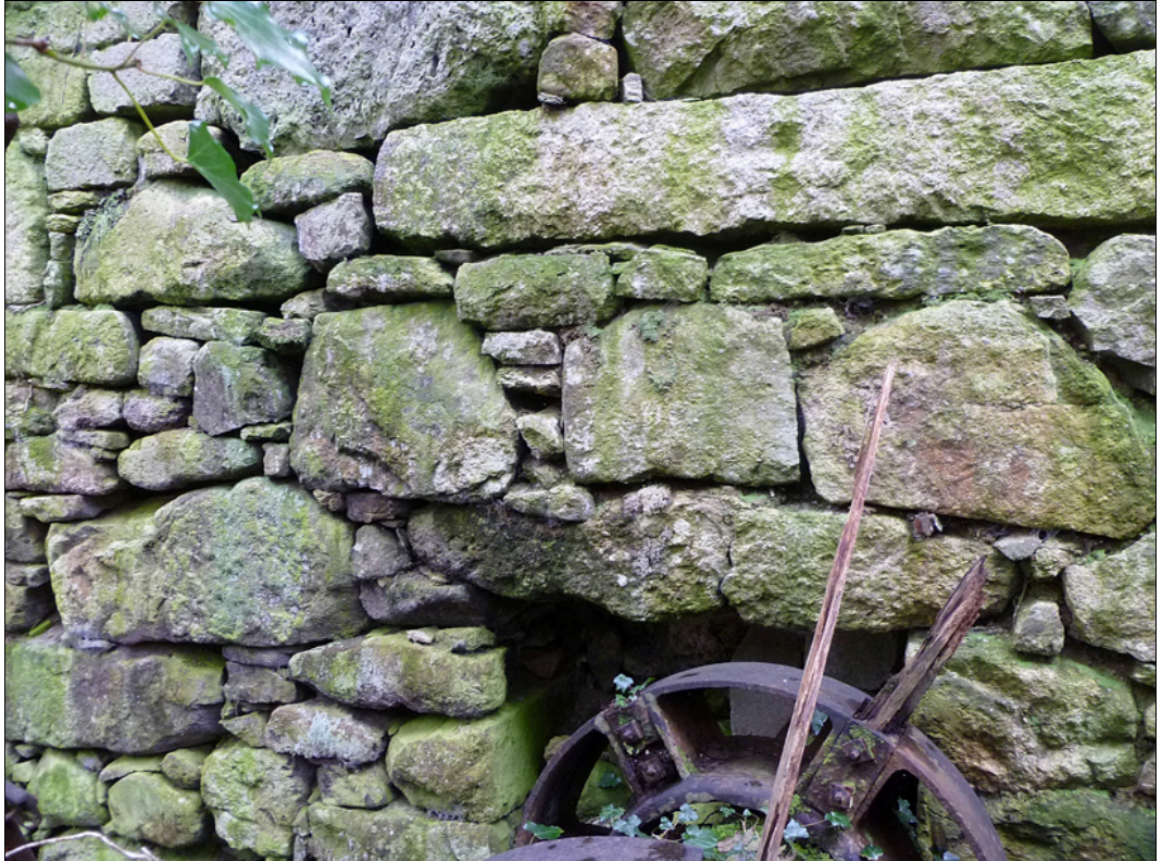
Detail of the opening and shaft through the wall into the Mill.
