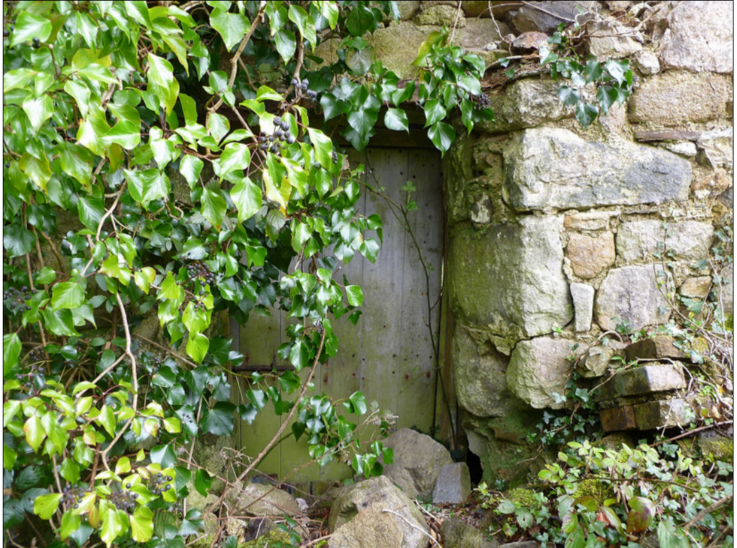
Detail of the internal face of the south-east elevation, showing the doorway.
