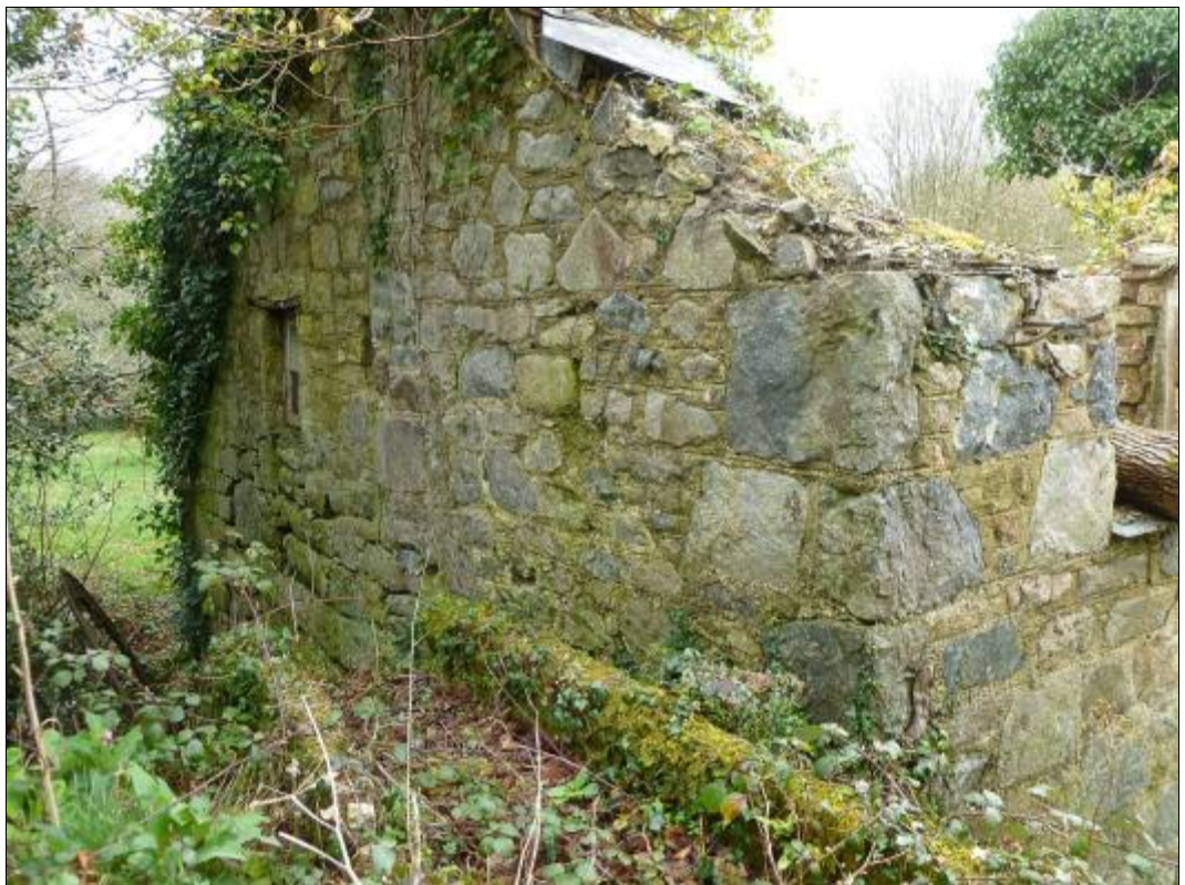
North-west corner of the Mill, upper part of pit wall, with granite trough in foreground.
