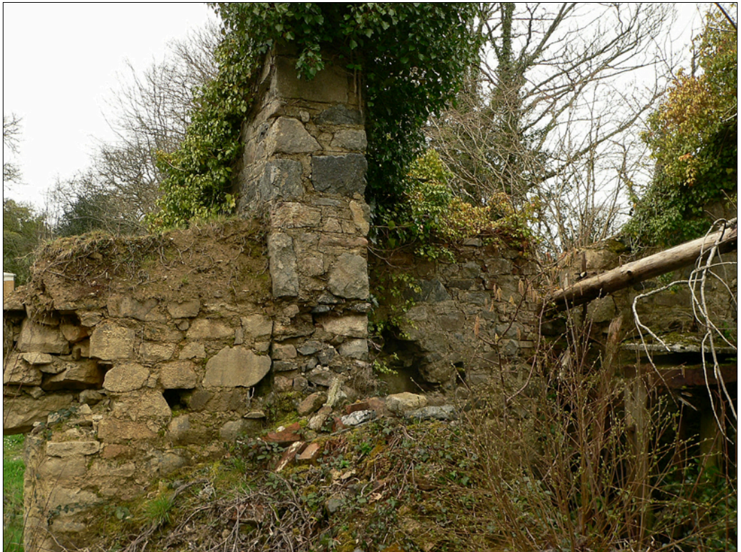
The (now collapsed) partition between the Mill and the Cottage, viewed from the south-east. Note the Cottage walls about the Mill, and the probable presence of a door between the two at first-floor level.
