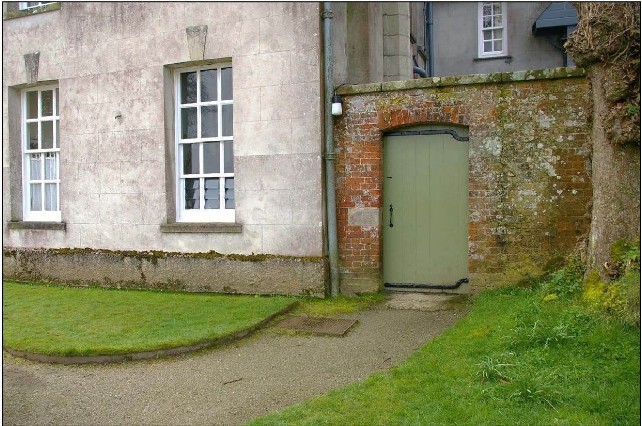
View of the north-west corner of the House and abutting brick wall to the west, showing the location of the proposed entrance of the pipework into the building, beneath the end window; from the north-west.
