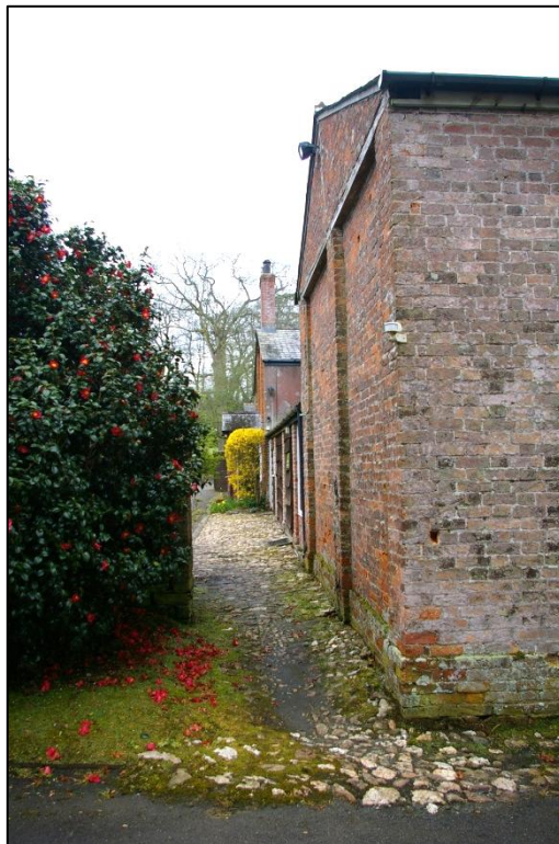
View along the southern elevation of the former stables pavilion building from the West Pavilion, showing the limited views from the ground floor of the West Pavilion; from the east.
