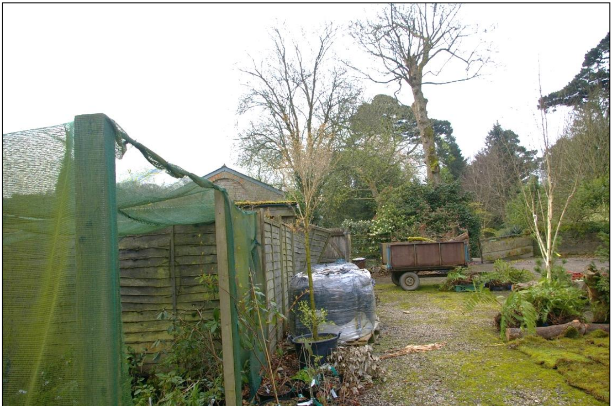
View up the western side of the proposed location of the biomass building site, showing the line of the second run of trenching; from the north.
