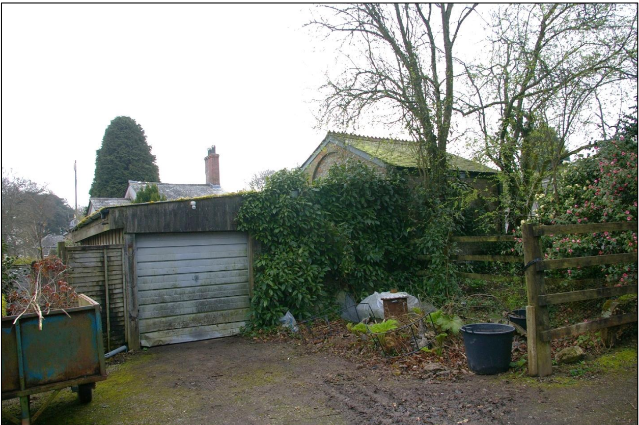
View of the west pavilion of the brick former stables and the adjoining mono-pitch timber-framed shed, which will be retained; from the north-west.
