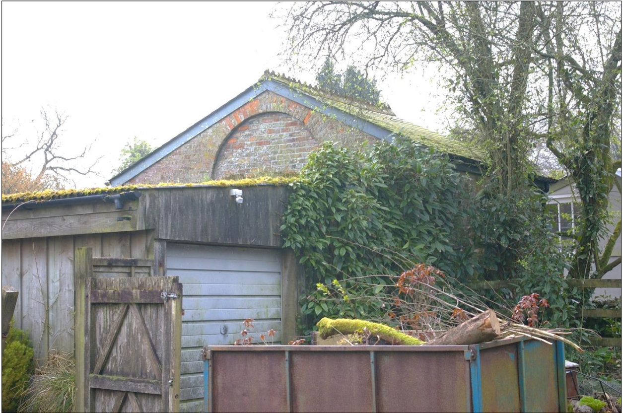
The western pavilion of the former stables building, showing how it is now abutted by a timber-framed shed; from the north-west.
