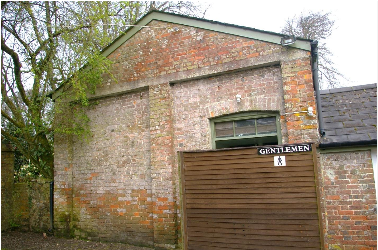
The south elevation of the building to the west of the former stables pavilion; from the south-east.
