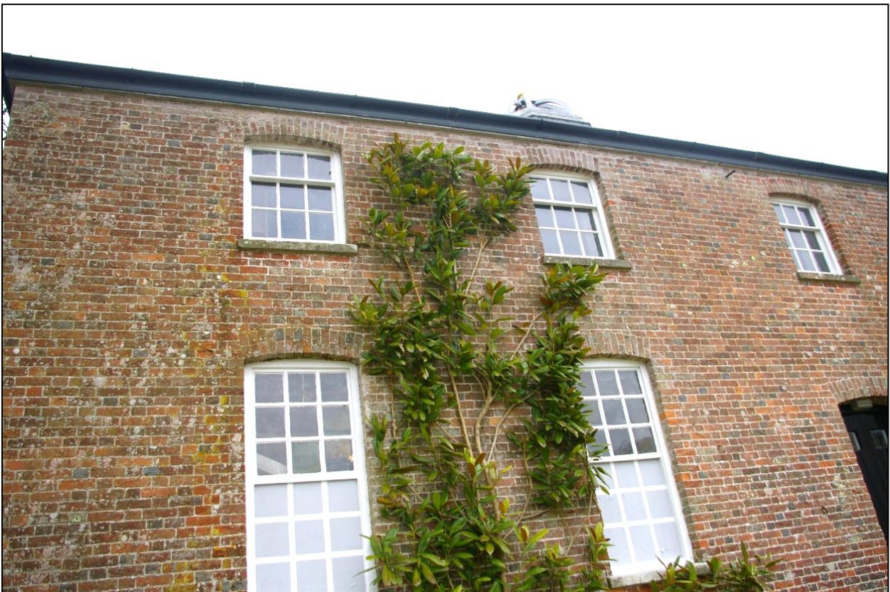
View of the four windows at the northern end of the western elevation of the East Pavilion, which may have some views to the proposed biomass boiler building; from the north-west.
