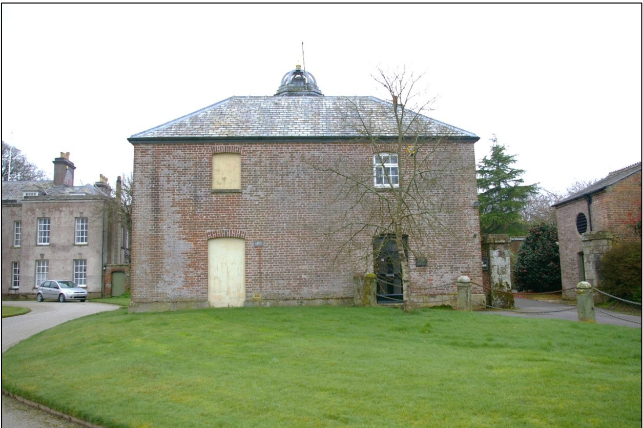
The north elevation of the West Pavilion, showing the blocked openings and one first-floor window to the north-west corner that might have very limited views to the proposed biomass boiler building; from the north.
