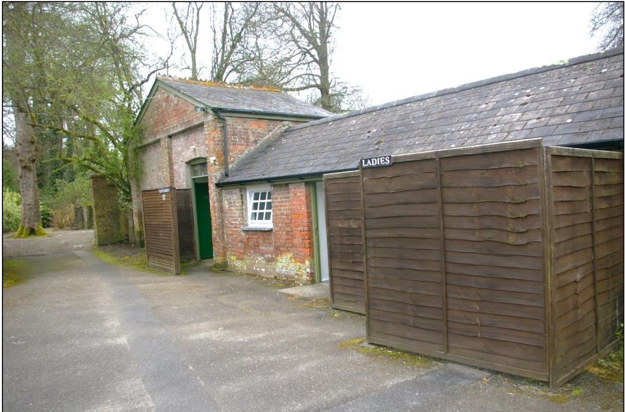
View back along the western end of the building where the trench line will run, also showing a current scar of a service trench which has been cut into the tarmac, indicating this area has been disturbed before; from the south-east.
