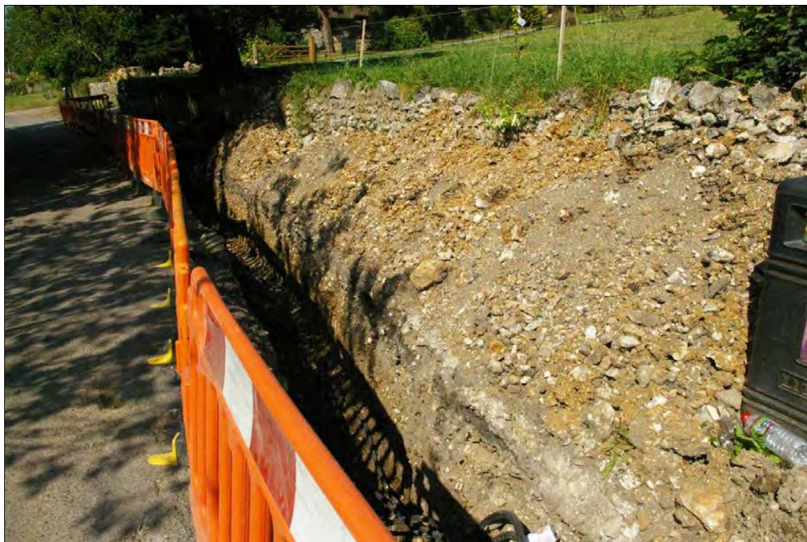
Figure 23: South facing section of Trench 06, showing modern road build-up layers; looking north-west.
