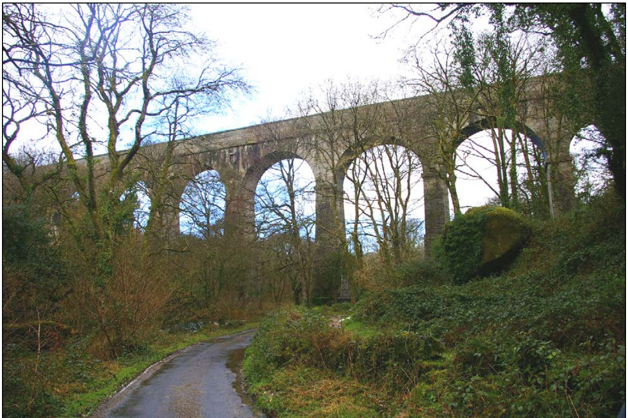
View from within Luxulyan valley, showing the Treffry Viaduct; from the south-east.
