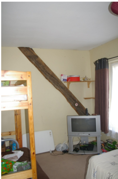
View of one of the 17th century truss blades, now within an internal partition, showing how the roof to the north side has been raised; from the south-east.
