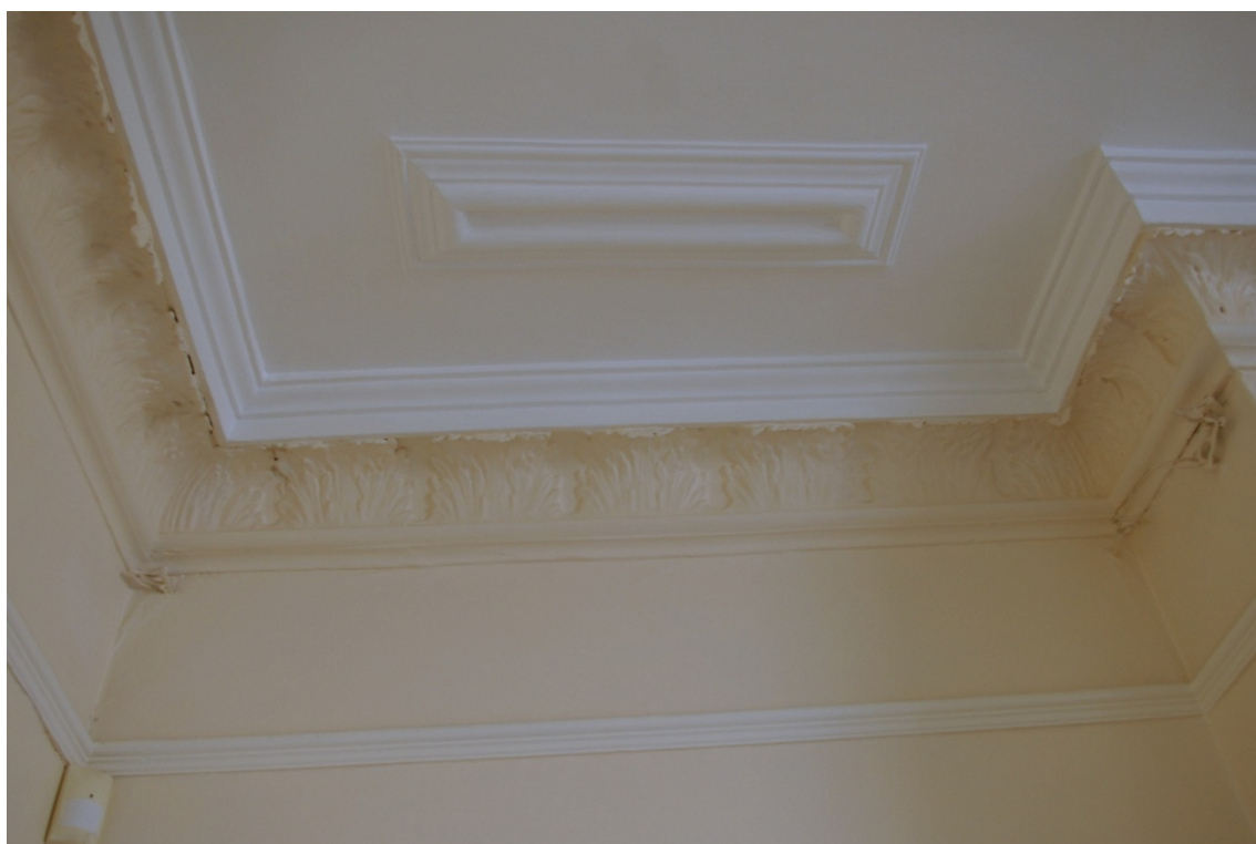
Room 2, the detail of one of the small ceiling panels in the southern alcove and the small bell pulls which survive, also showing the later 19th century addition of the acanthus leaves to the cornice; from the east.
