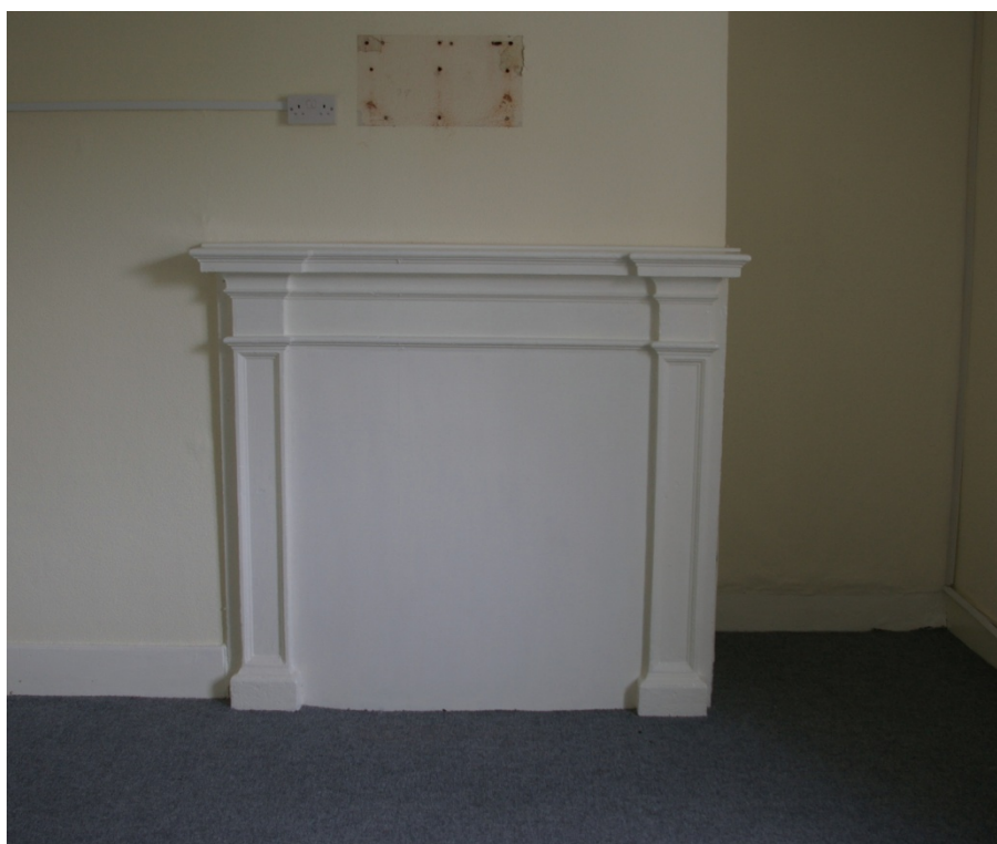
The fireplace in room 5, where it can be seen to project slightly away to the south from the south side of the chimney stack; from the west.
