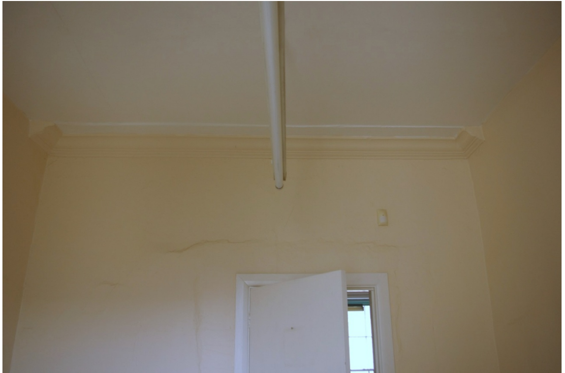
Figure 7: Room 3, the north wall showing the surviving section of cornice and the scar around the door opening; from the south.
