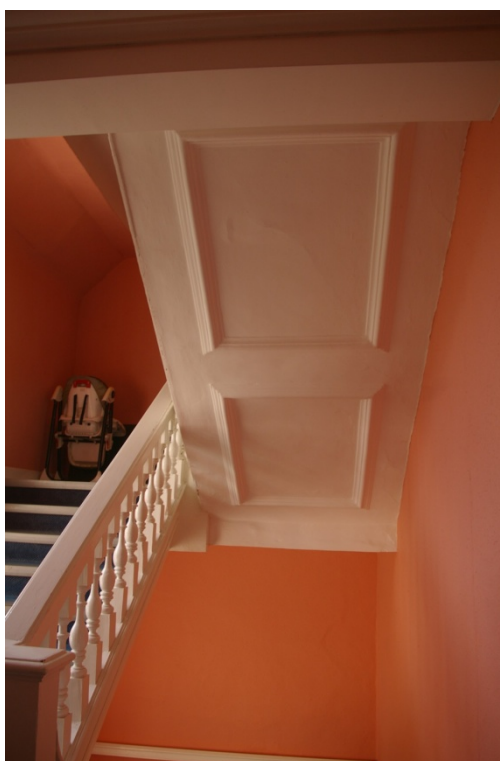
View of the moulded plaster panels on the cantilevered sections of the stair, visible from the first floor landing; from the east.
