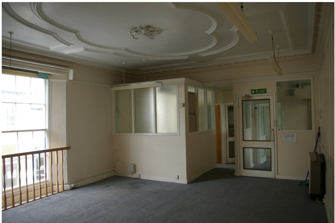
Figure 6: View across Room 2, towards Room 1 and Room 1A, showing how the historic wall of the original lobby has been removed and modern partitions inserted, also showing the large 19th century window in the north wall; from the south-west.
