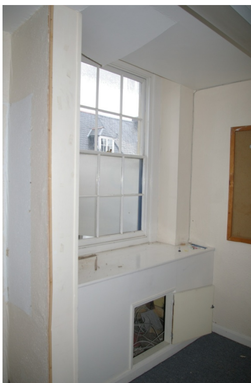
Room 1A, the stub of the historic wall of the lobby and the reuse of the 17th century window opening, now with a 19th century sash; from the south-west.
