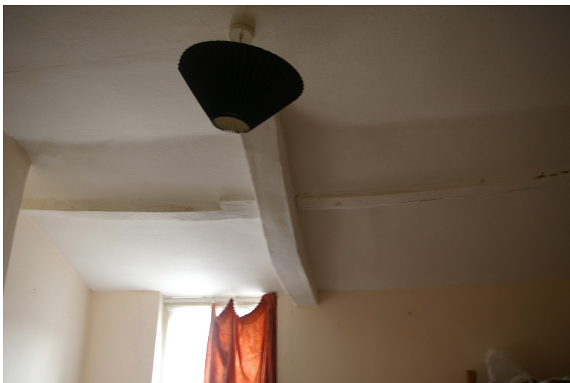
View of part of one of the 17th century trusses and purlins within the second floor; from the north-west.
