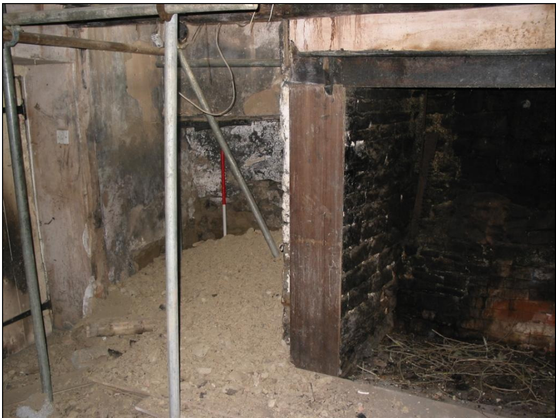
Figure 11: The fireplace in the eastern room of Unit 1 and the blocked opening in the northern alcove, viewed from the southwest (1m scale).
