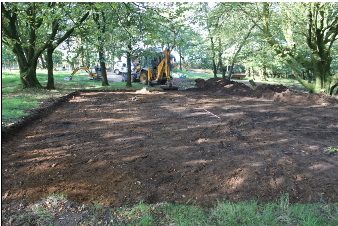
Figure 4: Shot of the area stripped for the middle lodge, viewed from the north-east (2m scale).
