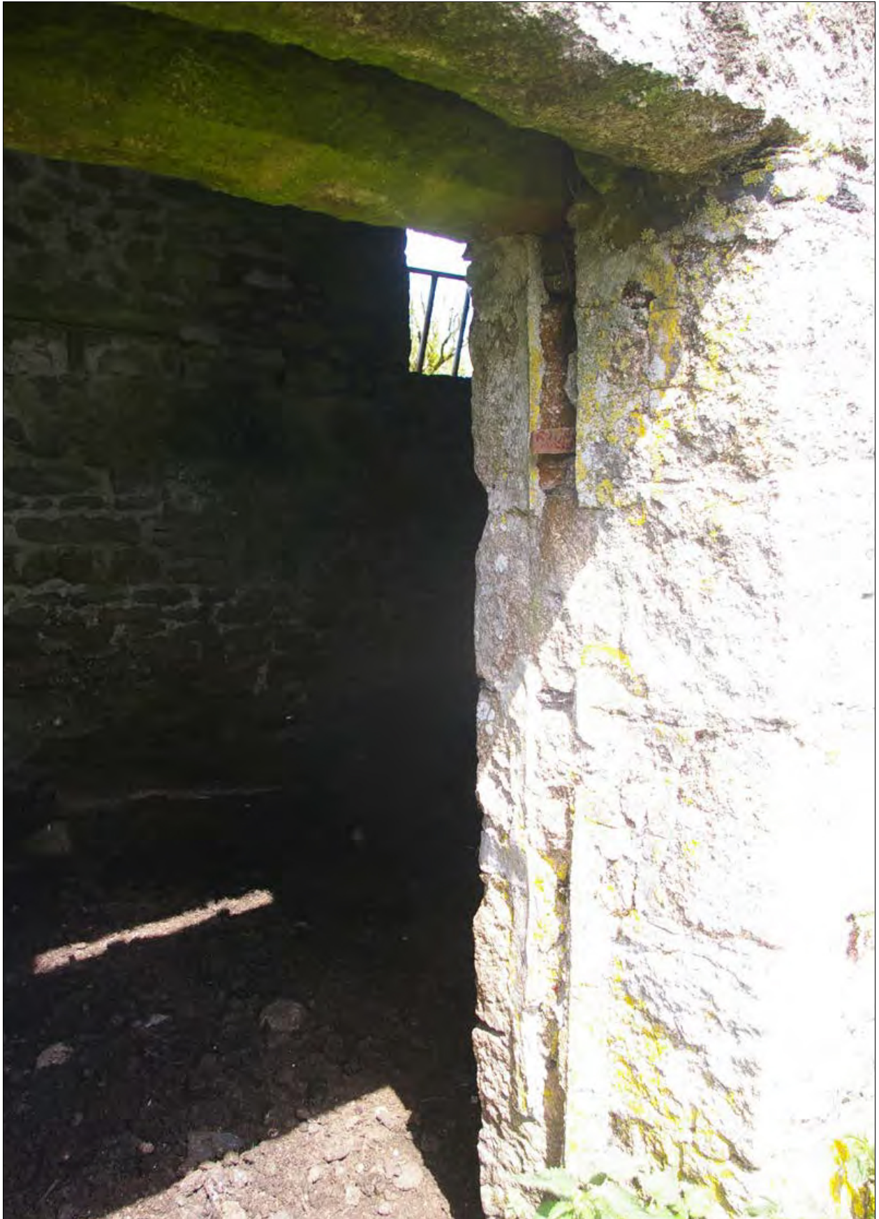
The entrance to the barn, on the south elevation, on the ground floor, showing the granite slabs which form the doorway; from the south-west.
