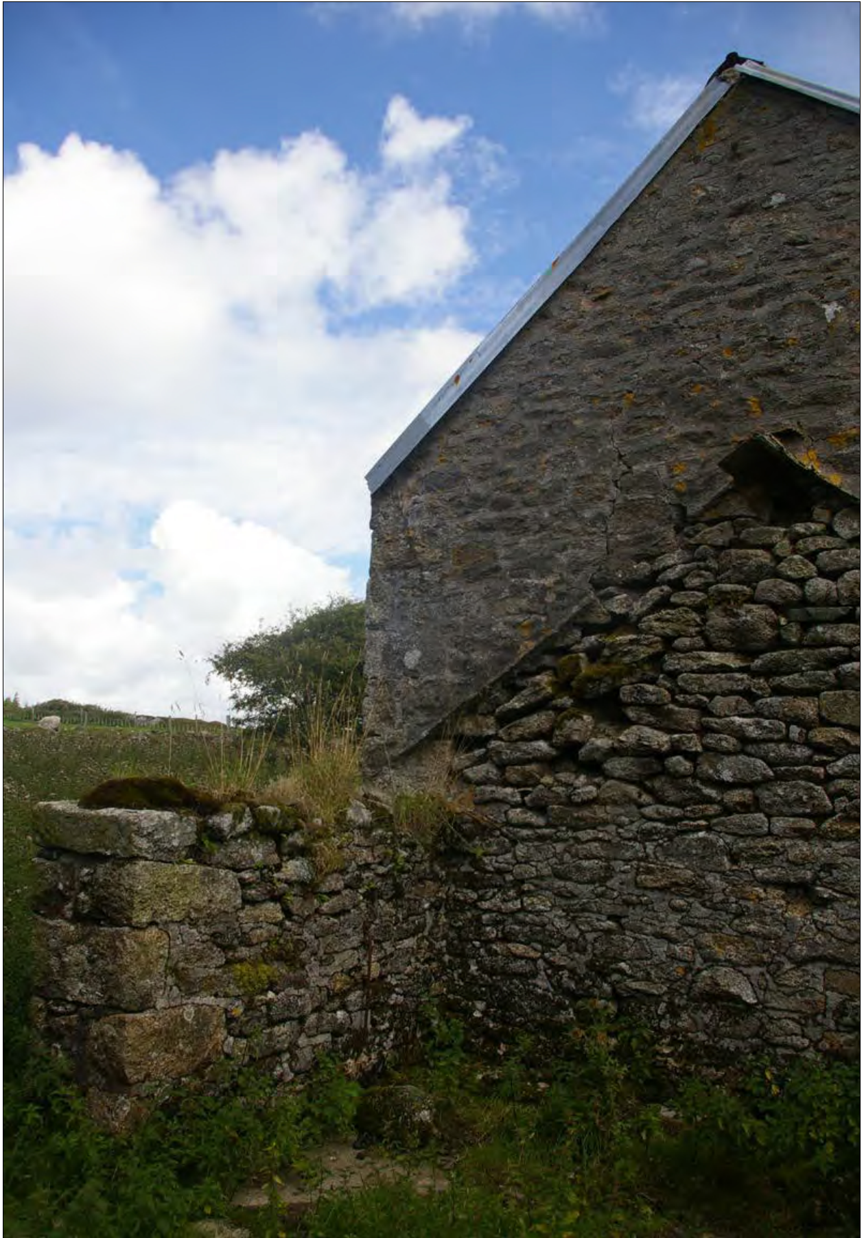
The adjoining buildings, Building 1 and Building 1a, on the north side; from the south-west.
