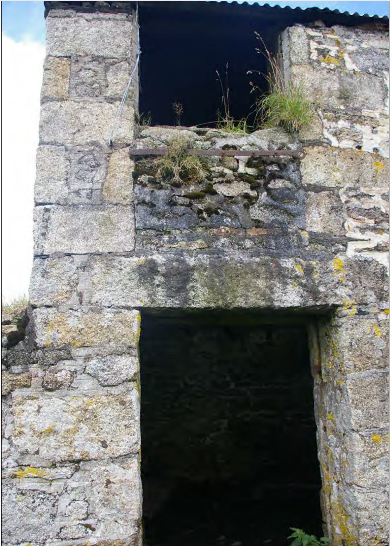
The symmetrically placed openings at the western end of the south elevation of Building 1; from the south.
