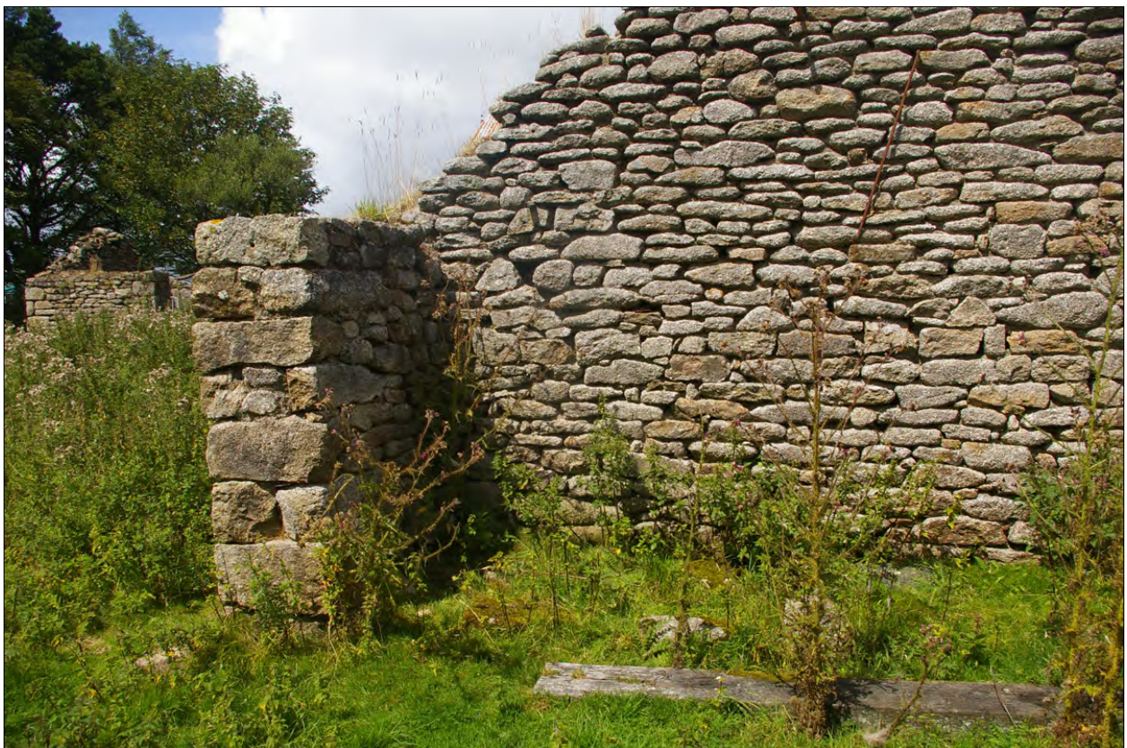
The north gable wall and short section of west wall of Building 2a; from the south, south-east.
