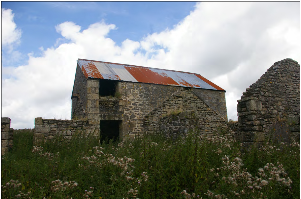
Figure 12: South elevation of Building 1, showing the roofline scar of Building 2c; viewed from the south-west.
