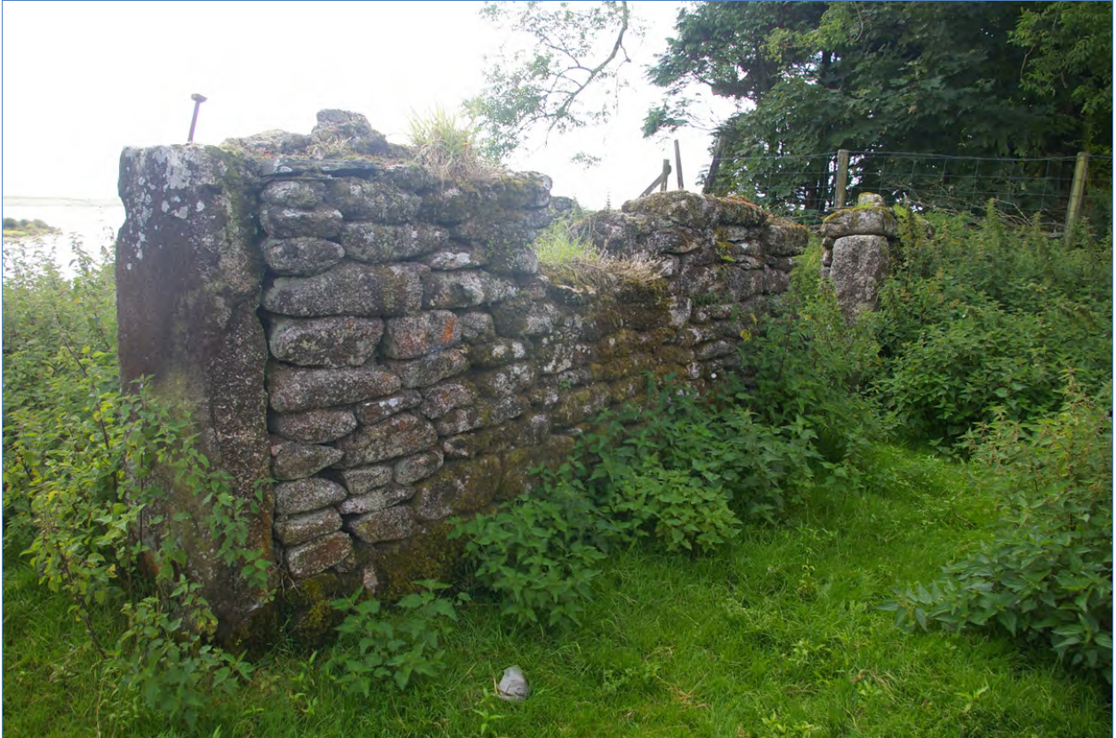
View of the north elevation of Building 3a, the western end, showing the use of granite slabs to brace the openings; from the north-east.
