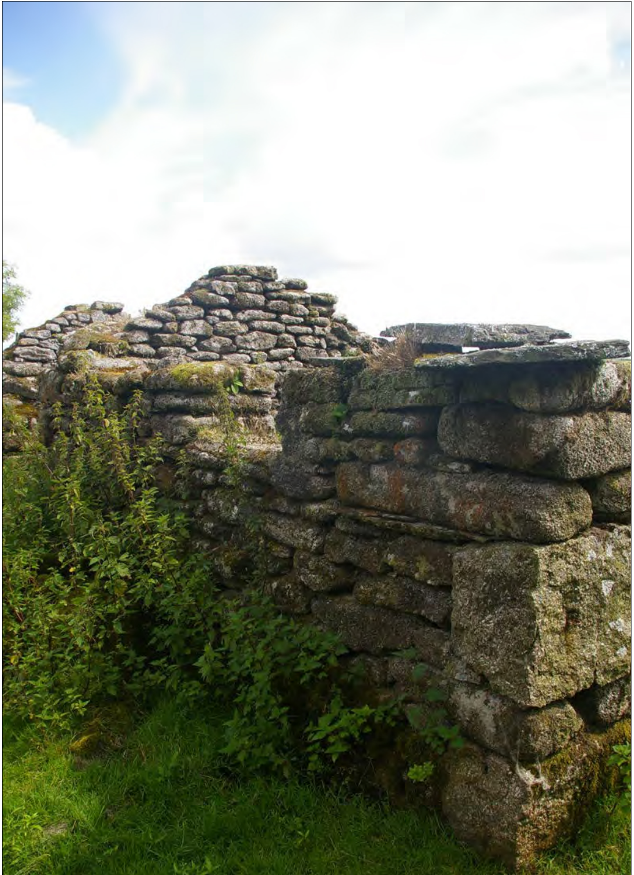
View of the north elevation of Building 3a, the eastern end, the earliest structure within the building range, showing the use of stone quoins, with slate levelling courses; from the west, north-west.
