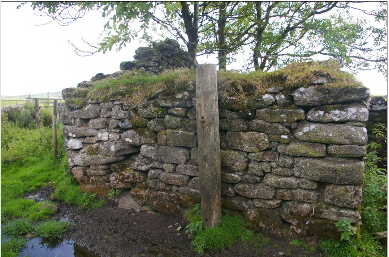
View along the north elevation of Building 3d; from the north, north-west.
