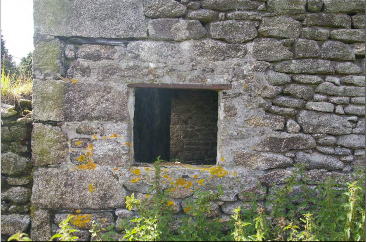
The opening in the east wall of Building 1, showing the disturbance around the opening, which appears to have been forced into the stonework; from the west.
