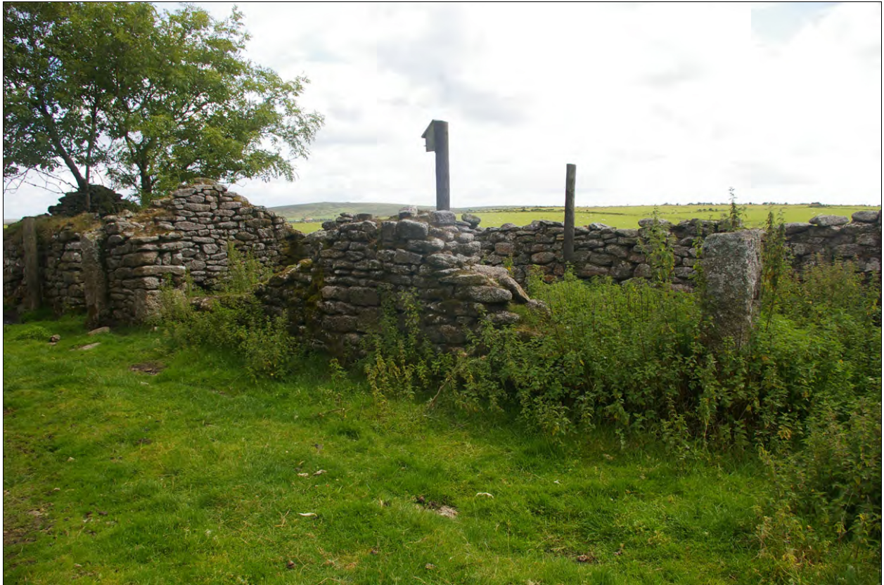
The north elevation of Building 3c, showing the ruinous status of the building; from the north-west.
