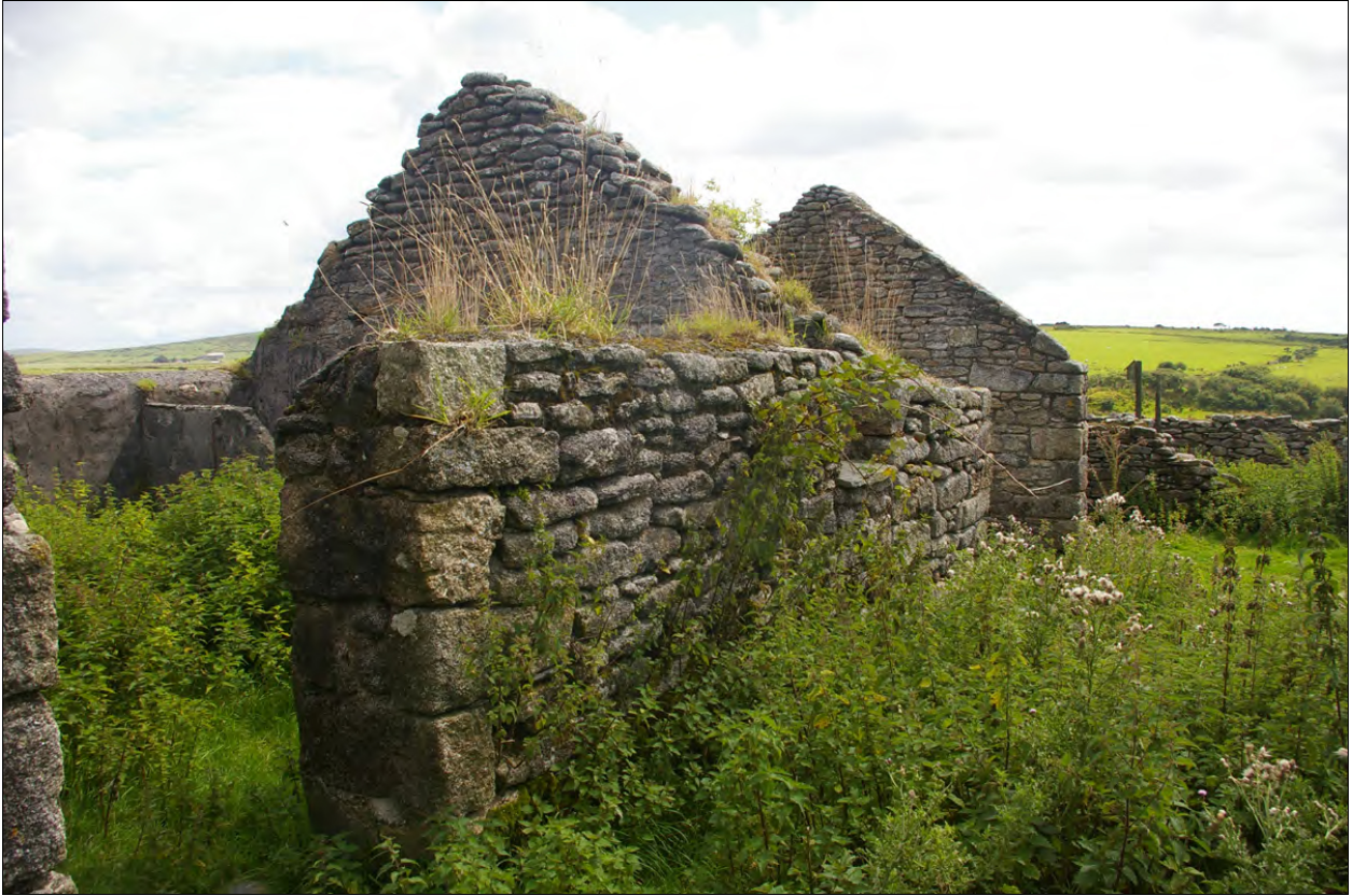
View along the west elevations of Building 2a and Building 2b; from the north, north-west.
