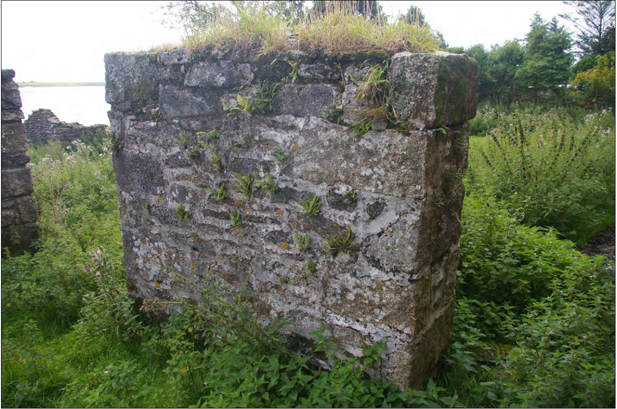
The interior face of the west wall of Building 2c; from the north-east.
