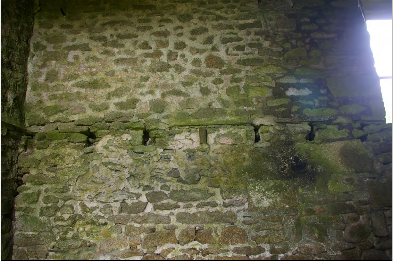
The western end of the north wall of Building 1; from the south.
