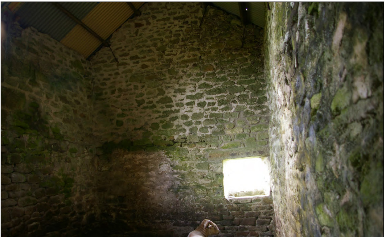
The eastern end of the north wall of Building 1 and the north-east corner of Building 1, the internal face; from the west, south-west.
