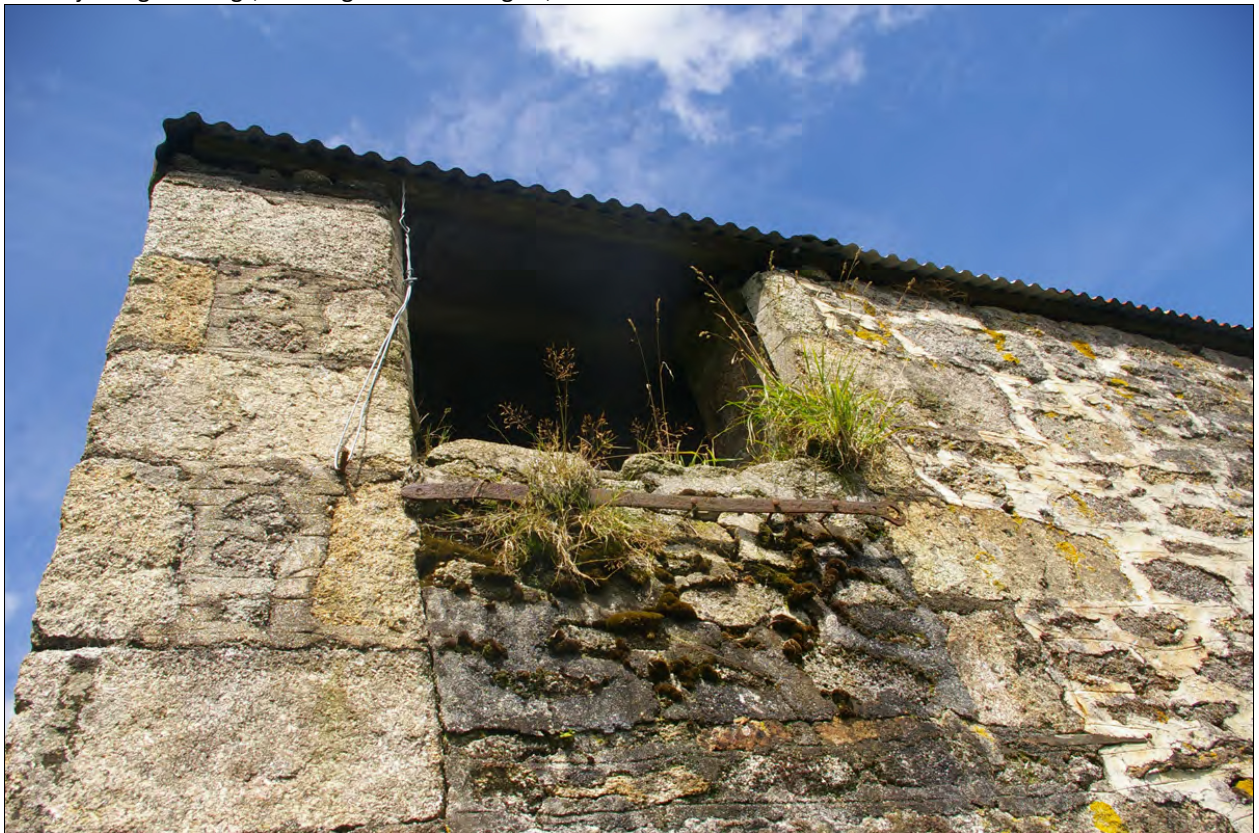
The first floor opening in the south elevation of Building 1, to the western end; from the south-west.
