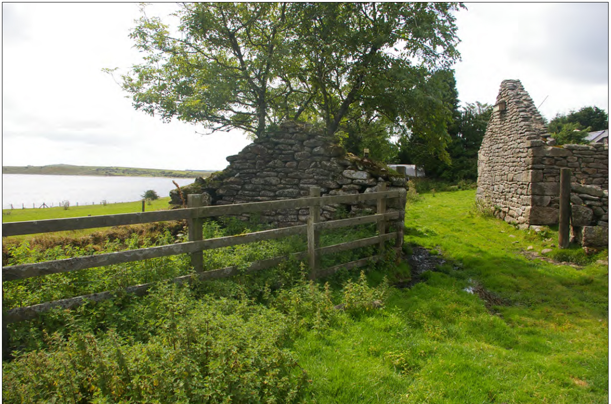
View of the east elevation of the building range Building 3, which forms the east gable of Building 3d; from the east.
