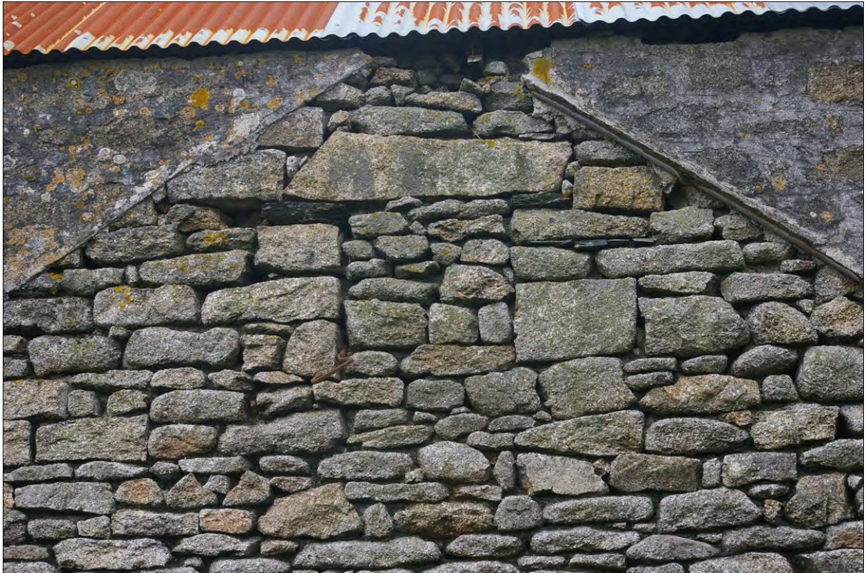
Detailed view of the blocked opening in the south elevation of Building 1; from the south.
