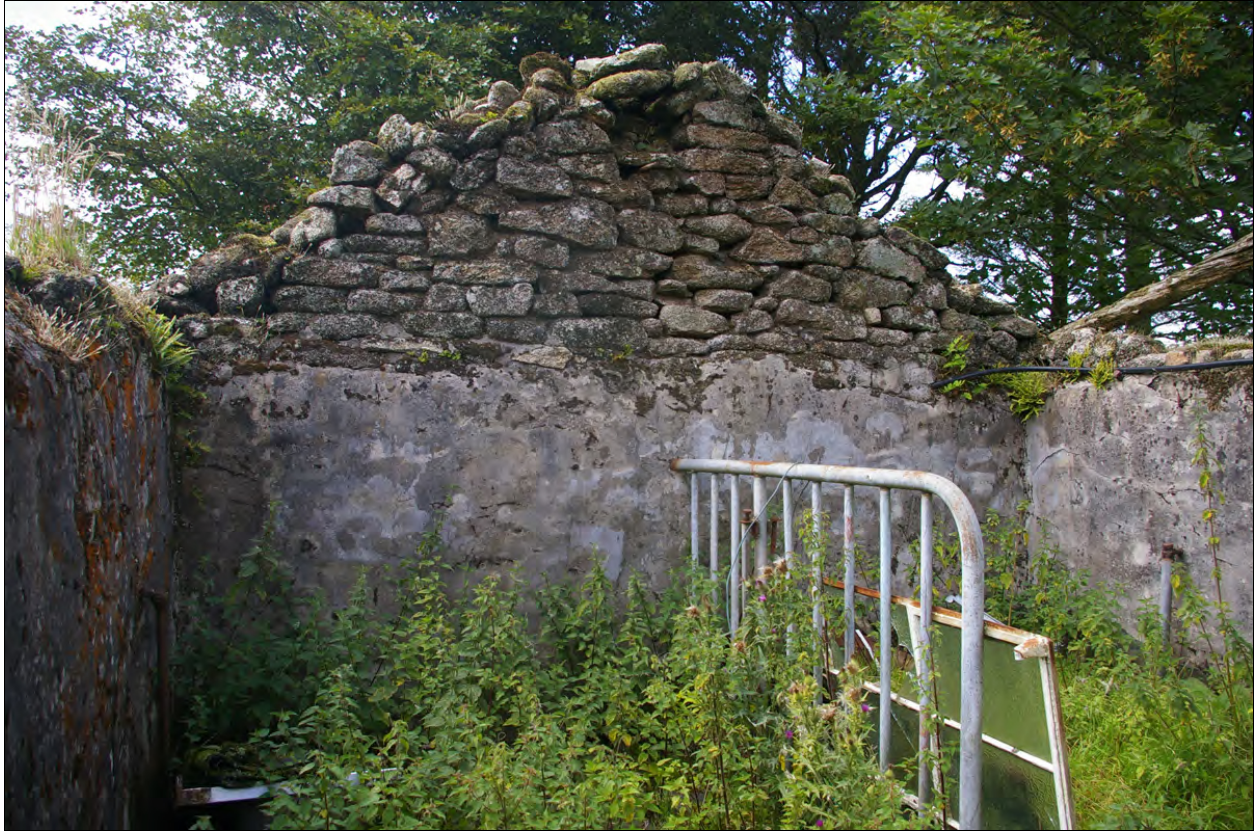
The interior face of the west gable of Building 1a; from the south-east.
