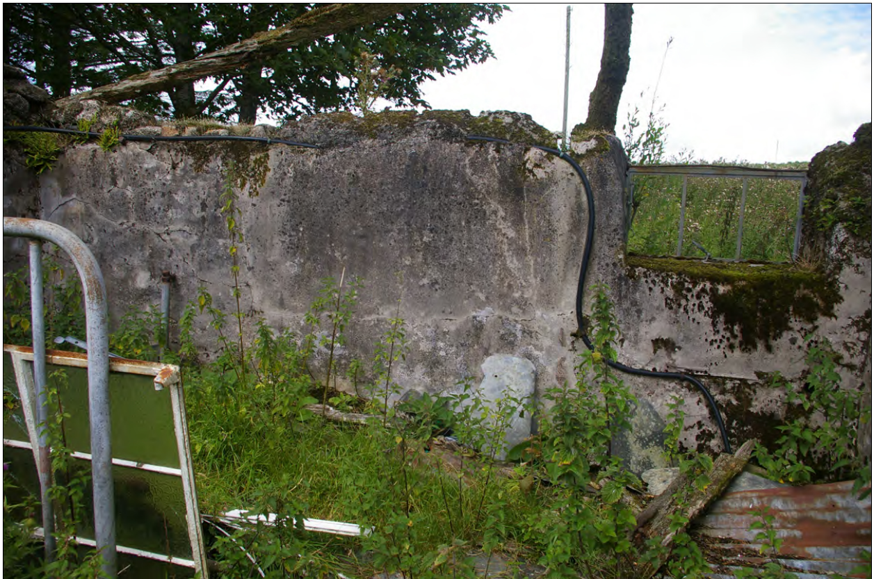
The north wall within the western compartment in Building 1a, with window with surviving metal frame; from the south-east.
