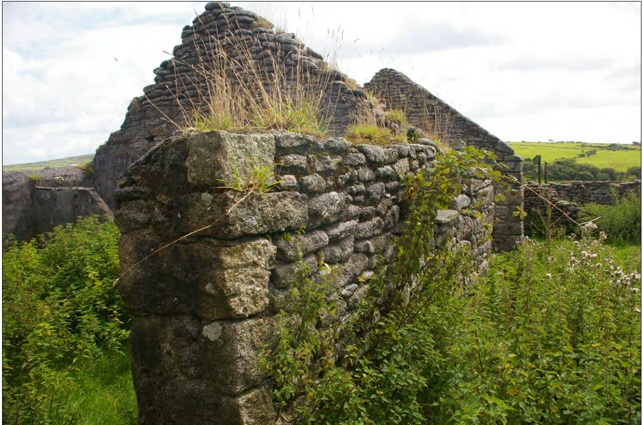
View along the west wall within Building 2b, a later addition; from the north-west.
