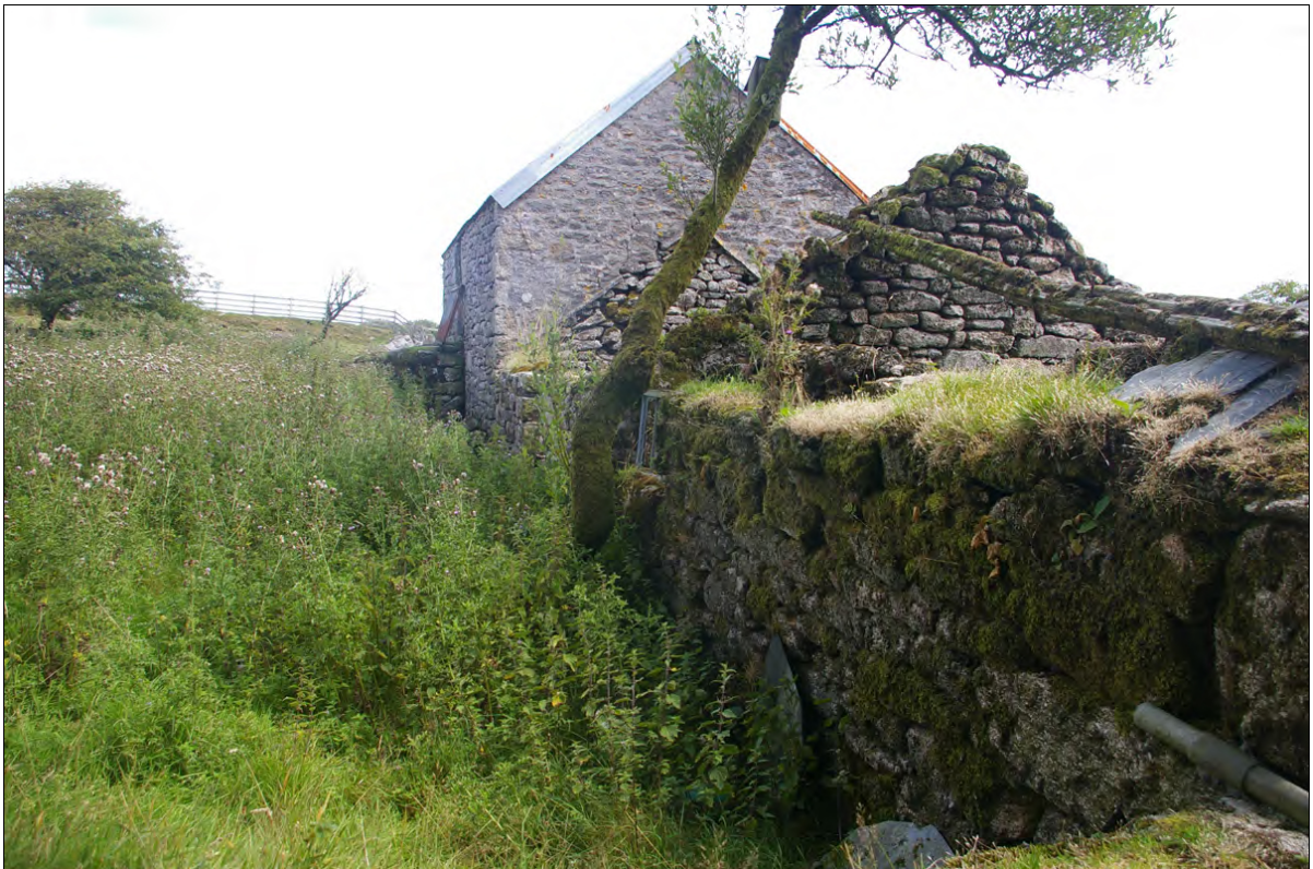
Figure 10: Shot along the north elevations of Building 1b (foreground) and Building 1a (with roof); viewed from the west.
