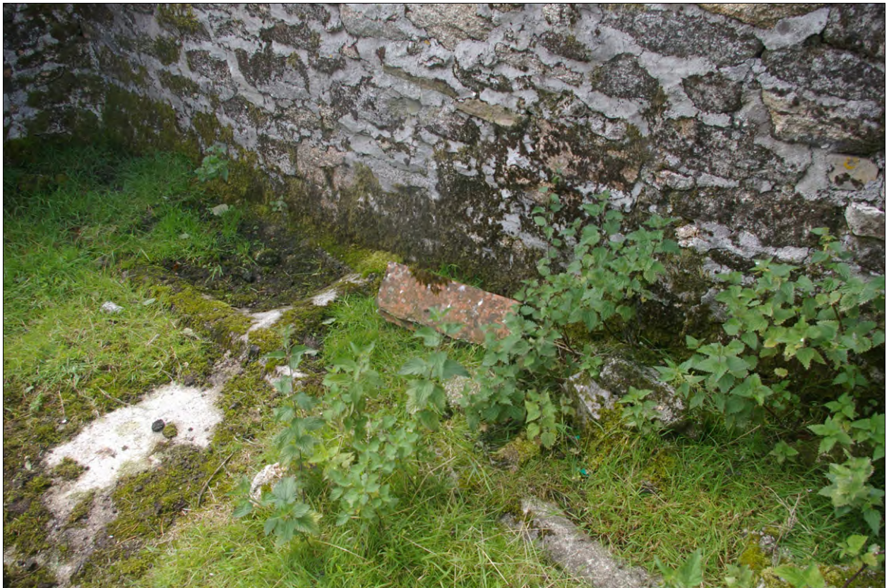
The remains of the former concrete pens, within the eastern compartment in Building 1a; from the north-east.
