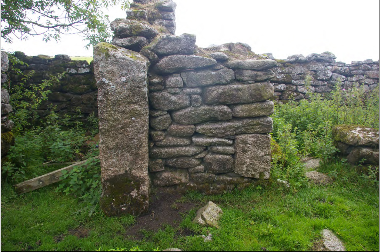
The north elevation of Building 3c and Building 3d; from the north.
