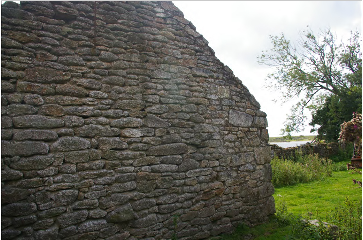
The south gable wall of Building 2a, showing the potentially rebuilt section; from the north-east.
