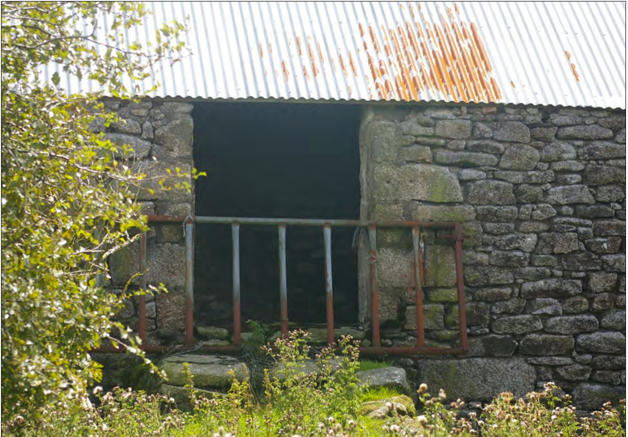
The loading door within the first floor of the north elevation of Building 1; from the north.
