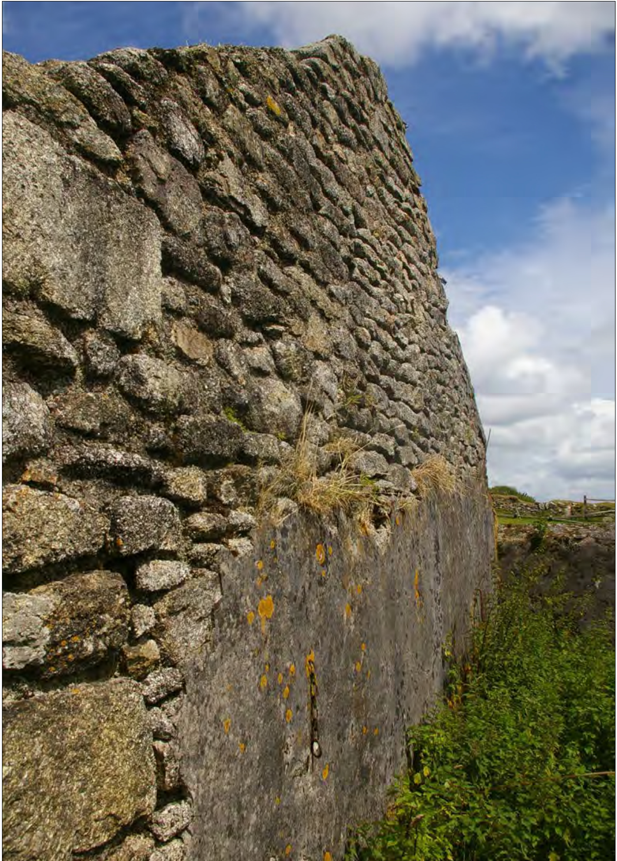
View along the north gable wall of Building 2b, showing the later cement render; from the west.
