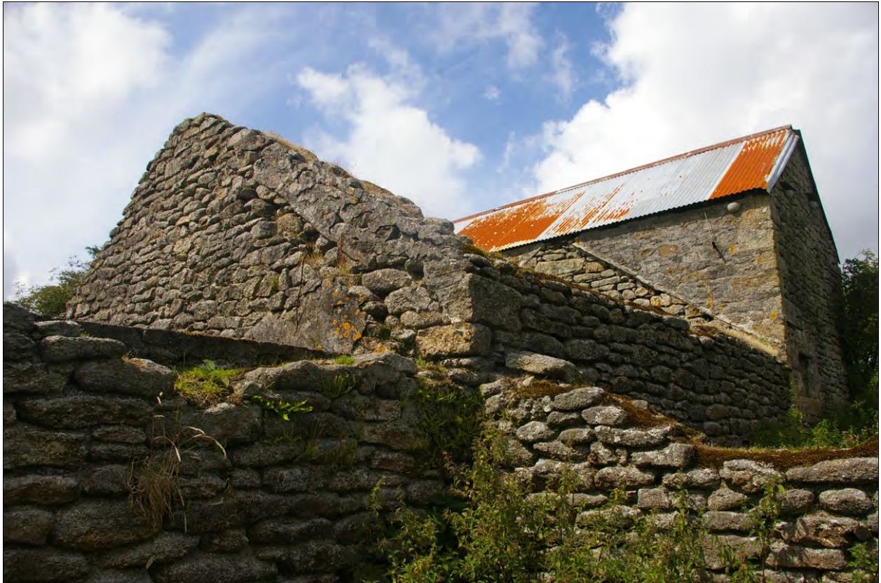
View of the north gable of Building 2b, showing how it has been raised, to allow for the new wall to Building 2c, to the north; from the south-east.
