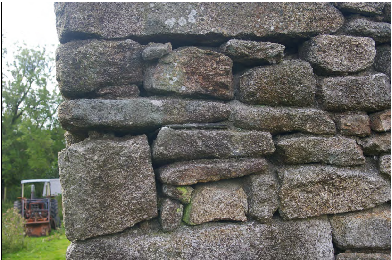
Detail showing the slate levelling courses between the granite block quoins of Building 2a; from the east.
