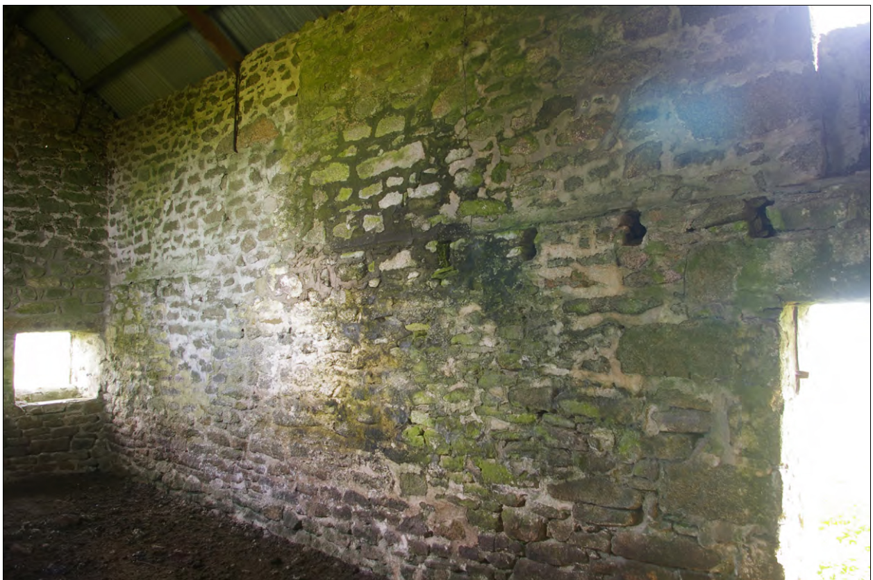
The internal face of the south wall of Building 1; from the north-west.
