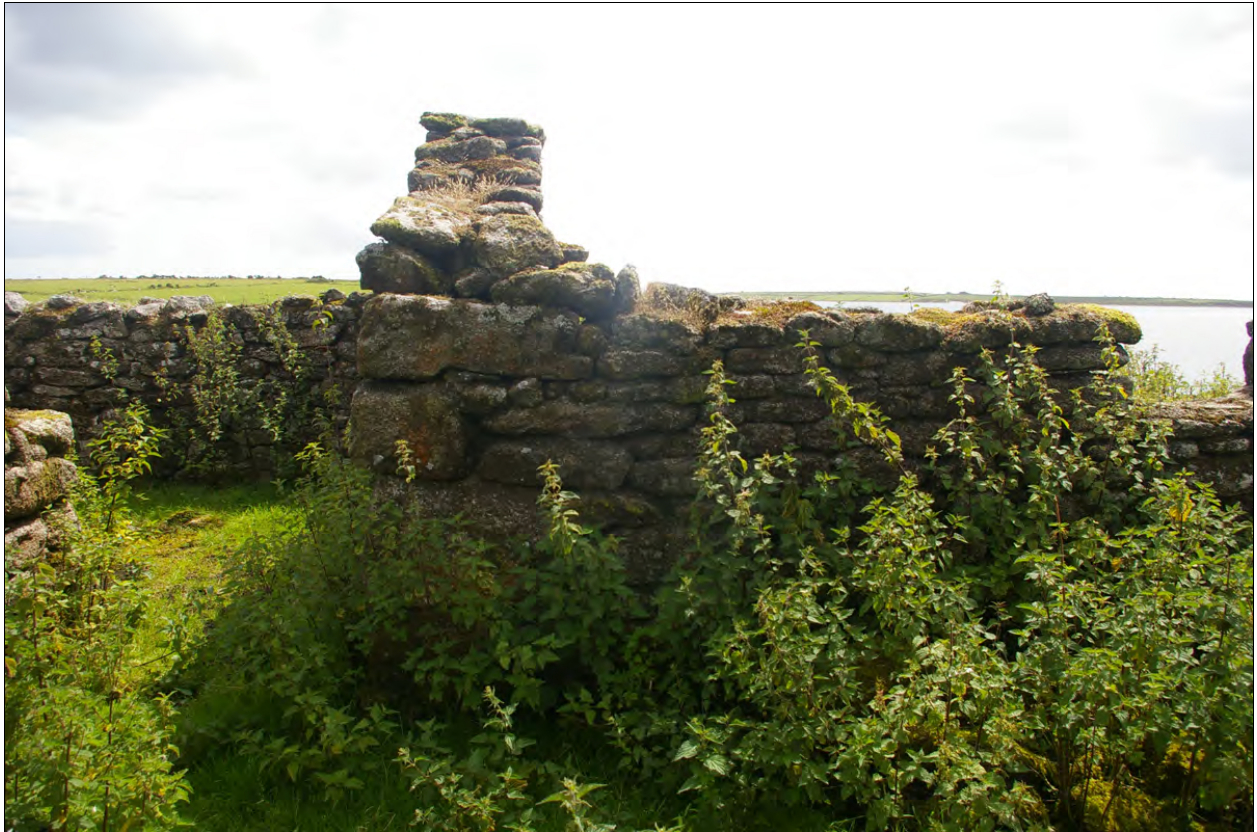
The north elevation of Building 3a, showing the large granite quoins on the eastern gable end of the building; from the north.
