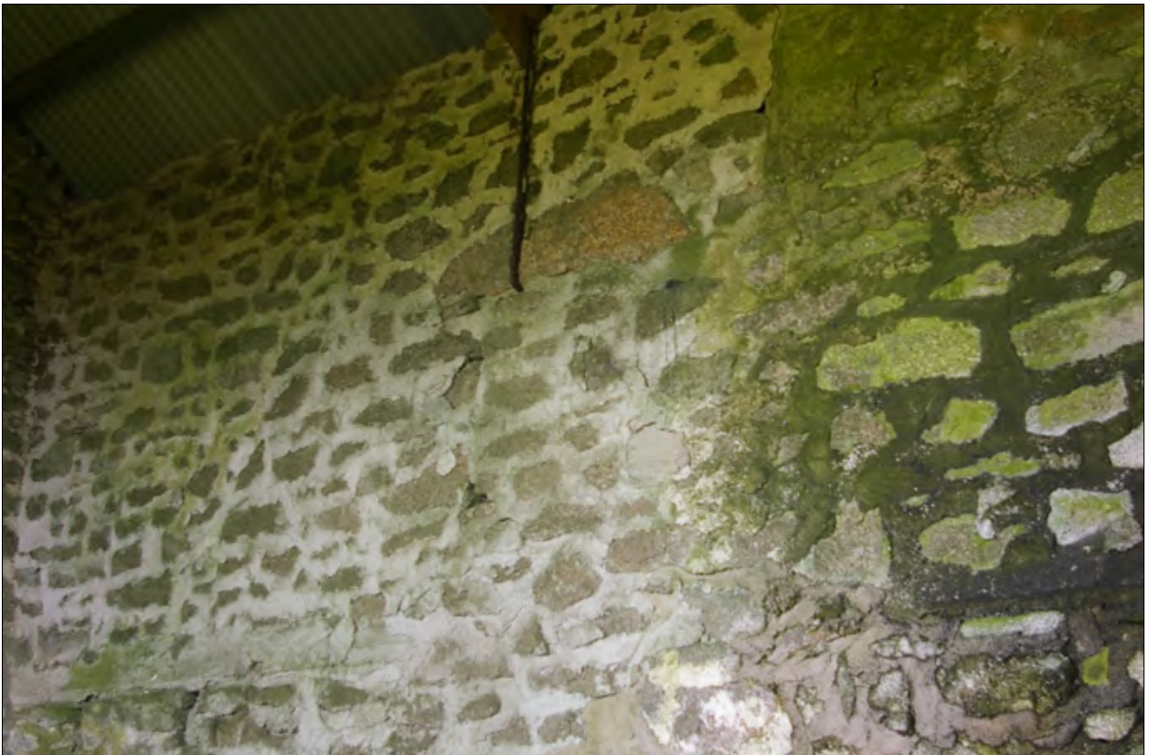
The interior face of the blocked opening in the south wall of Building 1; from the north-west.
