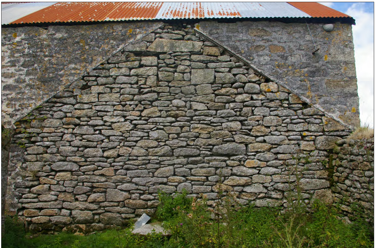
The roofline scar and sockets for timbers within the south elevation of Building 1, for the roof over building 2c, to the south; from the south.
