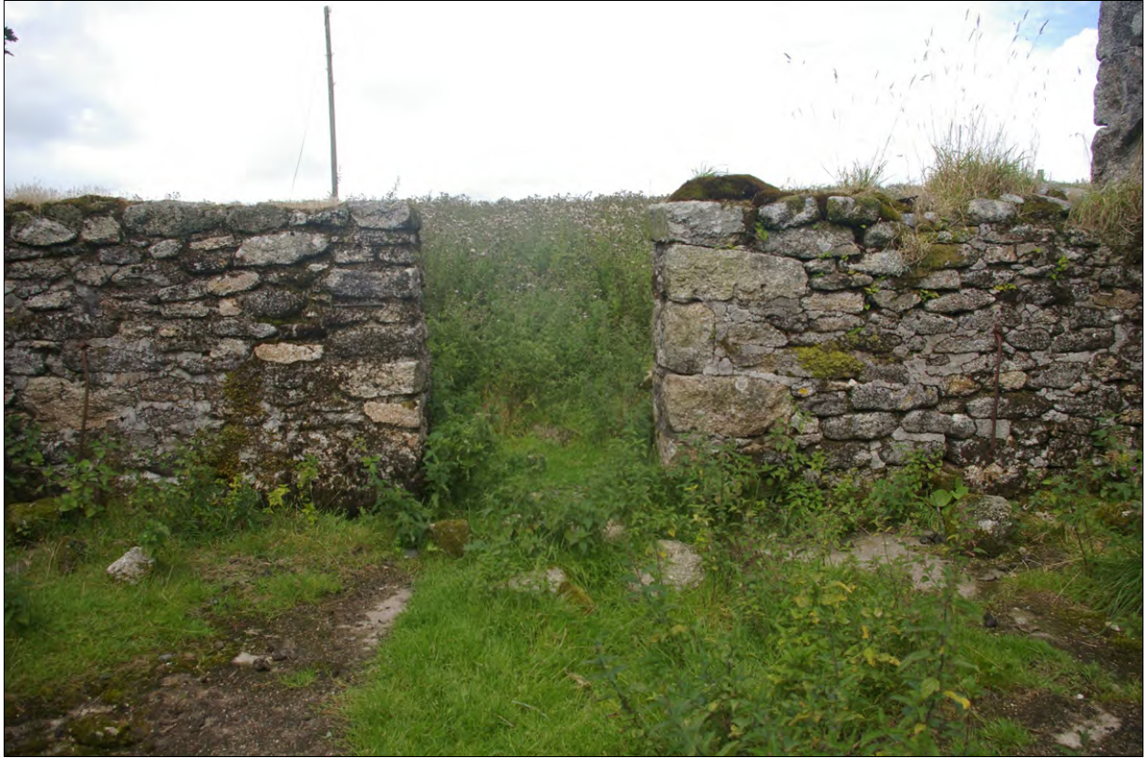
The north wall of the eastern compartment in Building 1a, the interior face; from the south.
