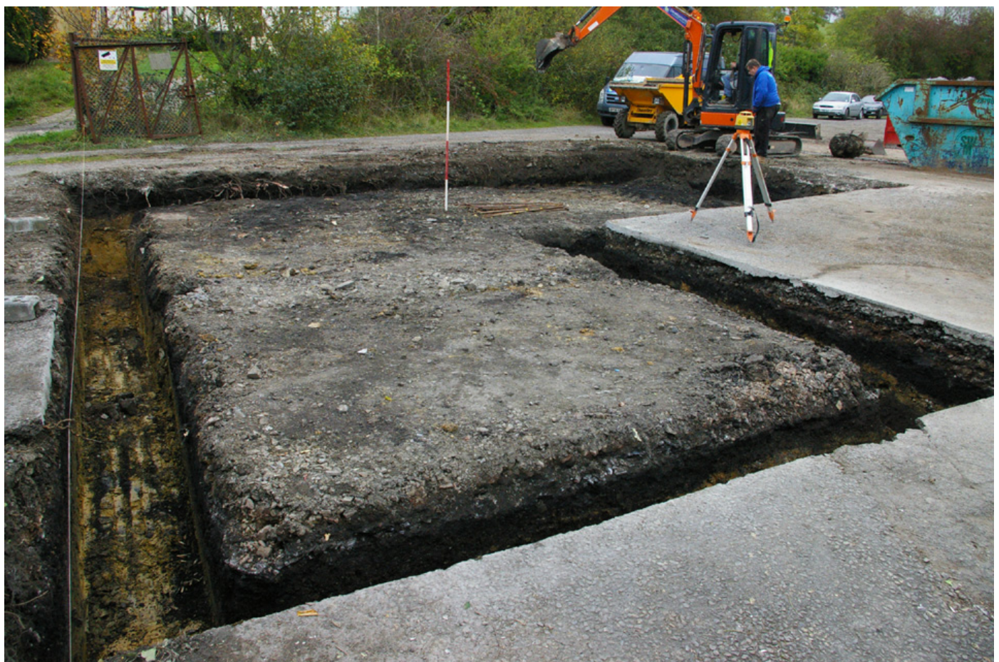
Figure 3: The excavated area, following the site strip and trenching; viewed from the west-north-west (scale 2m).
