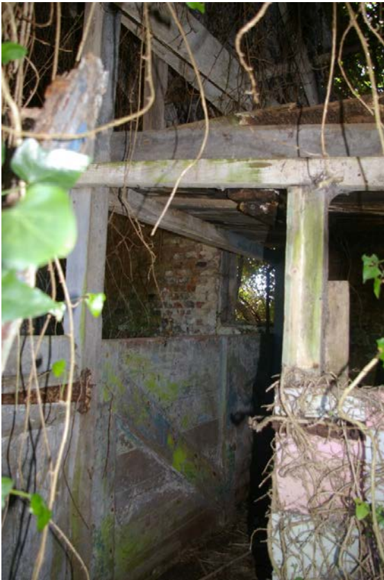
View of the interior of the two storey section of the building range, showing internal timber stalls; from the north-east.
