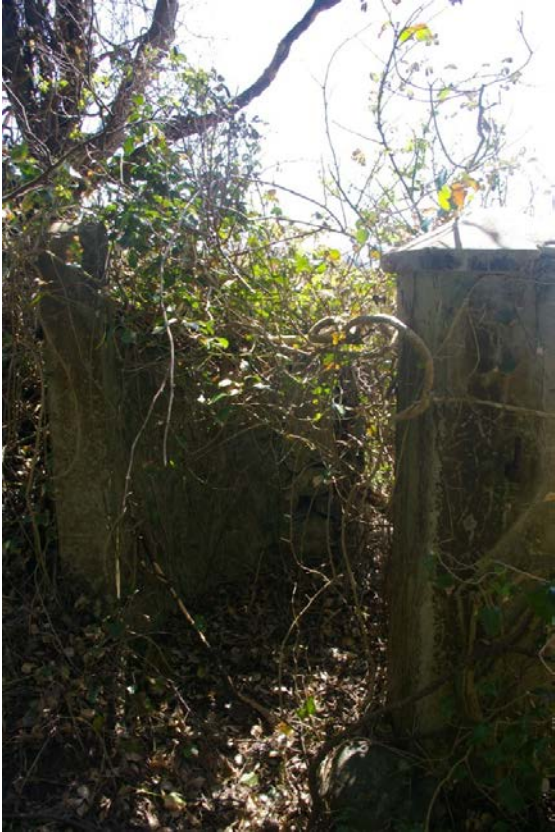
Detail of the curving flanking walls and gate piers; from the north-west.
