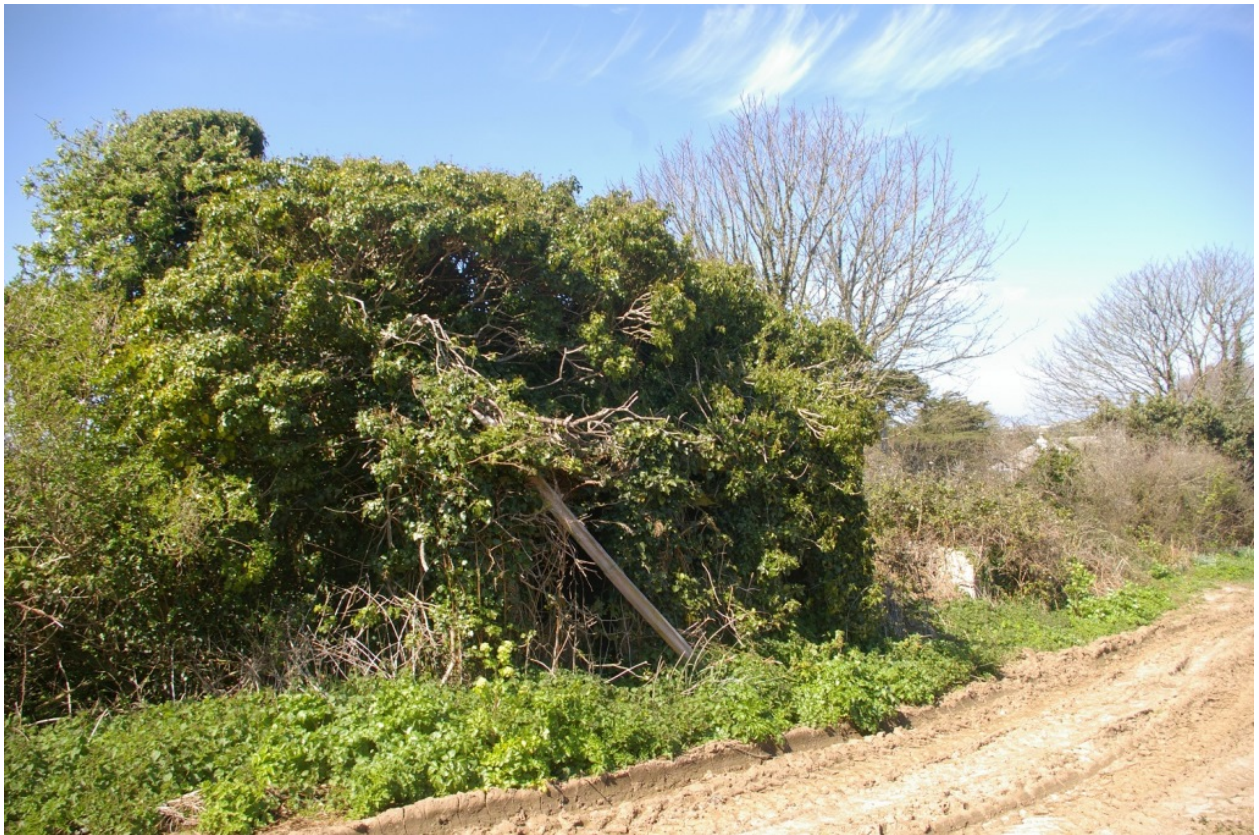
The brick and stone outbuildings, built up against the western boundary of the small field south of The Beeches; from the south-east.
