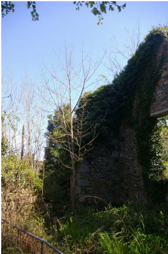
View to the south-east across the southern gable of the ropeworks; from the north-west.
