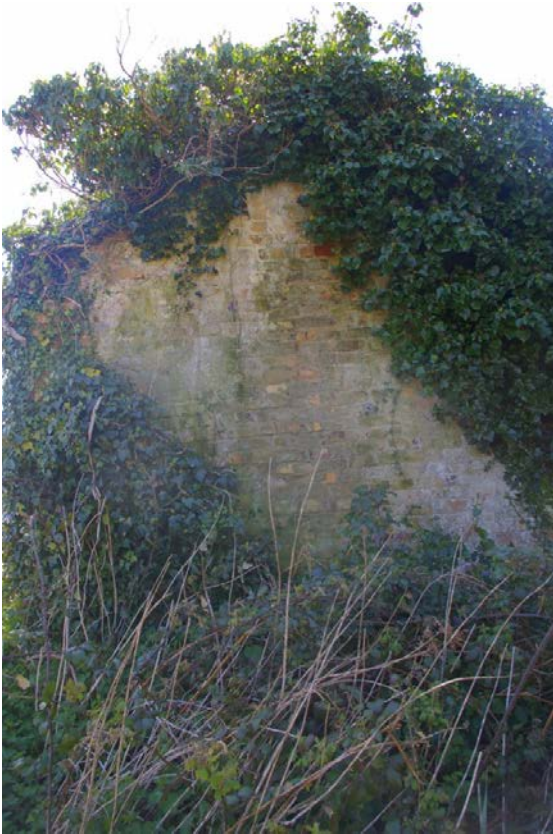
View of the tall gable end of the two storey section of the building range, built in brick; from the north.
