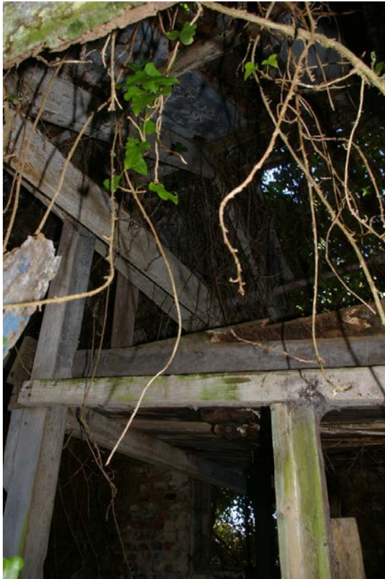
View up into the bolted A-frame timber roof structure of the building; from the north-east.
