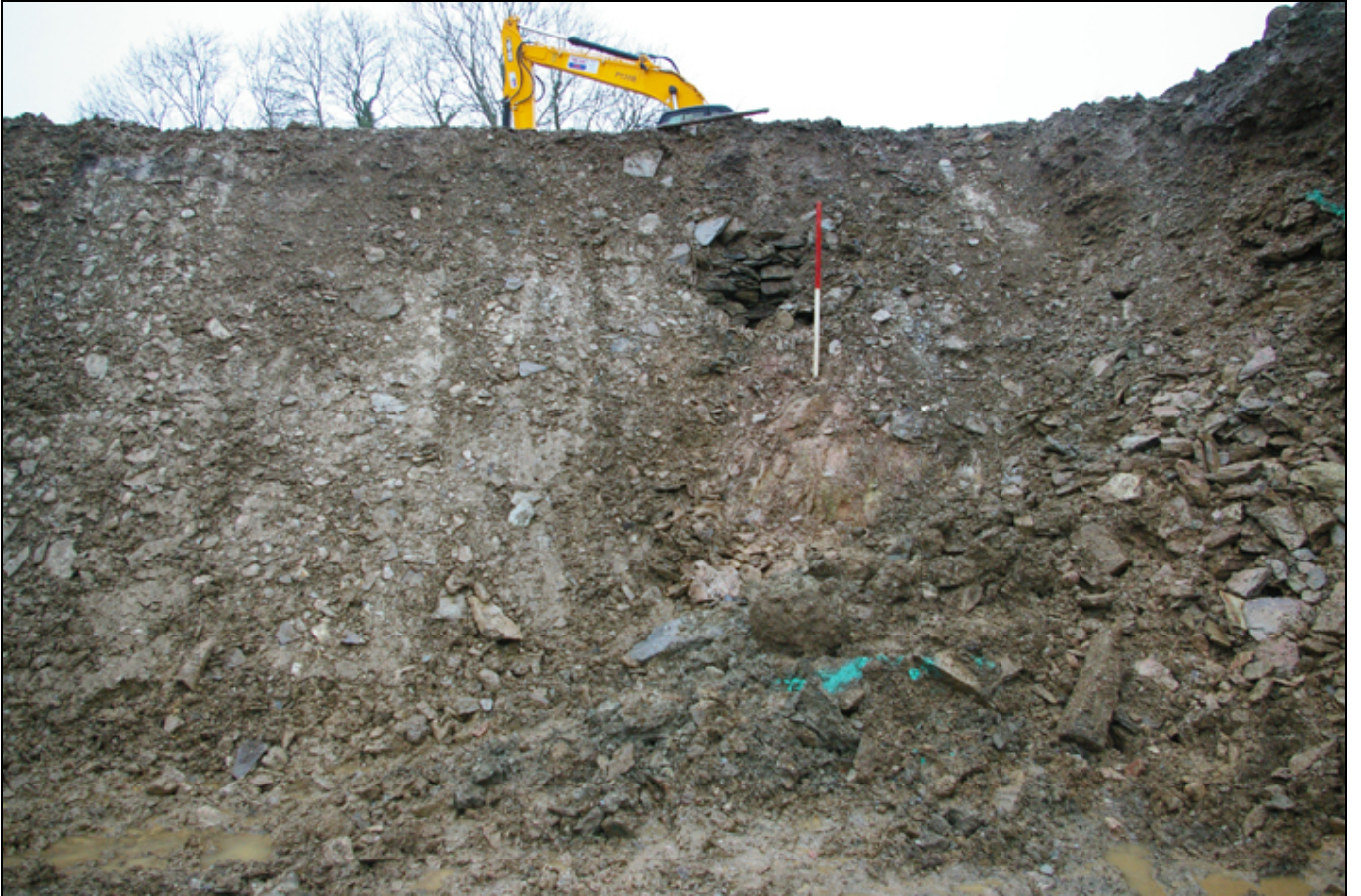
Figure 6: The first well, shown emerging from the battered slope of the excavation; viewed from the south-east (1m scale).
